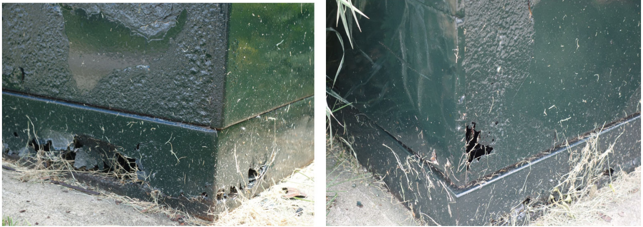
Figure 30: Excessive Corrosion of Enclosures on UG Pads
