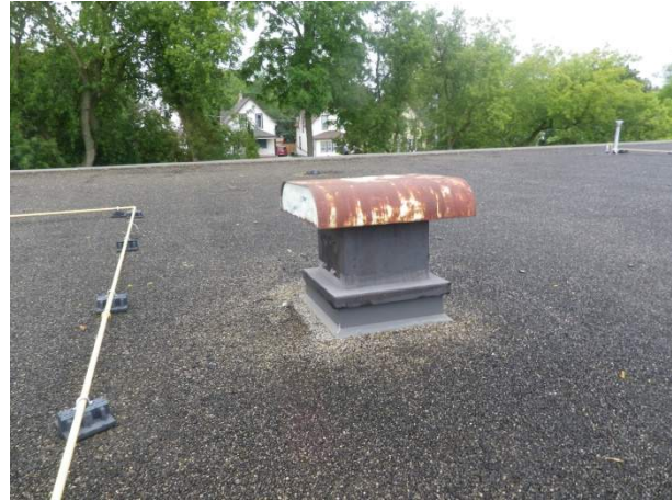
Exhaust fan hood for truck bay area
