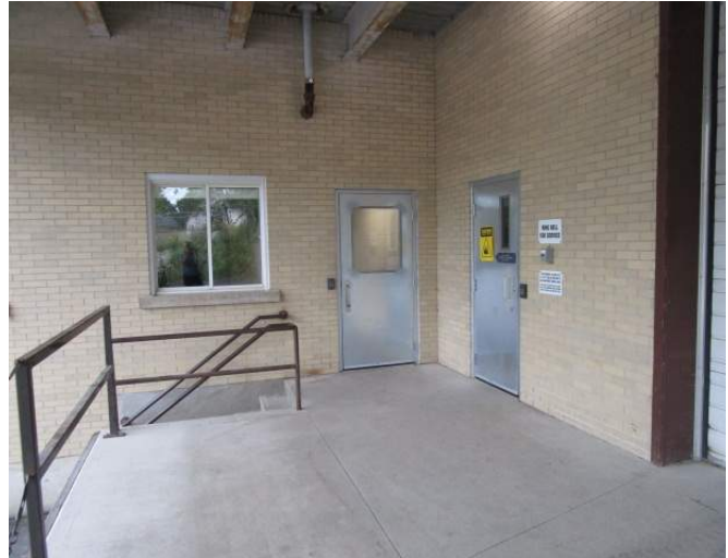
New metal doors / metal frames installed to provide access to the office area and the receiving area
