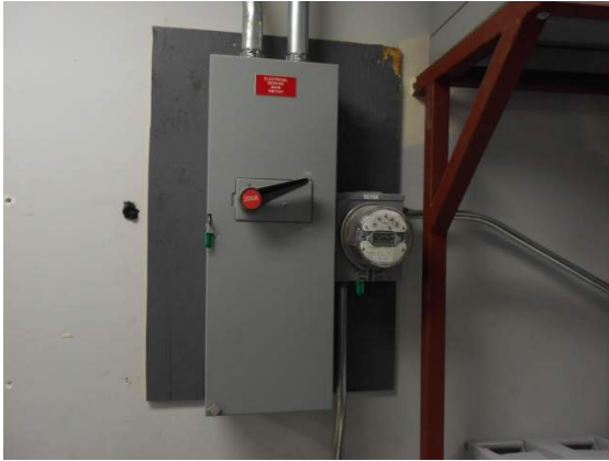
Main Incoming Service
