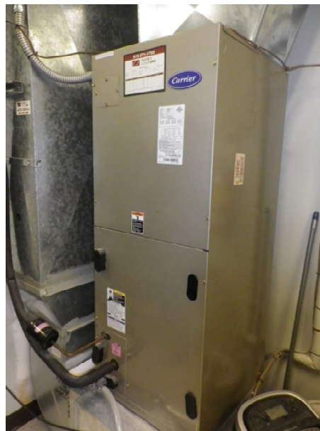
Fan Coil Unit – mechanical room
