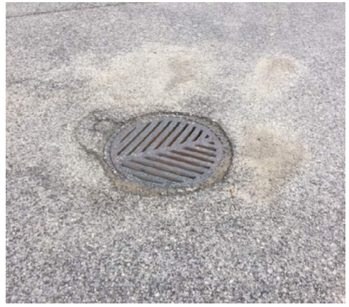
Storm Catch basin
