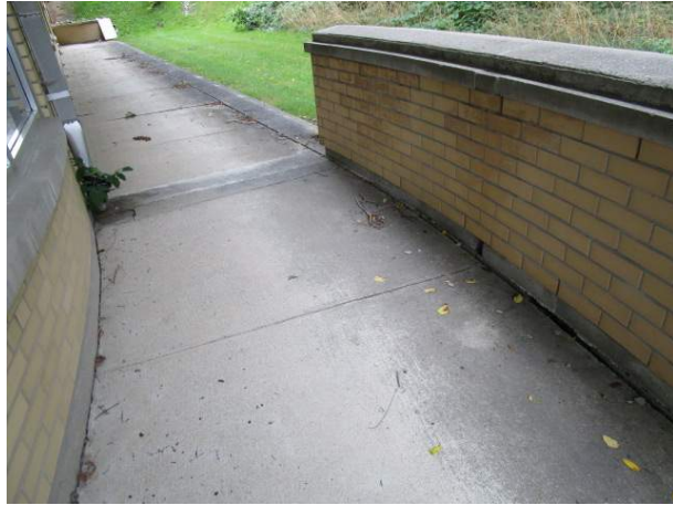
Roof drains empty behind the front 'feature' wall.
