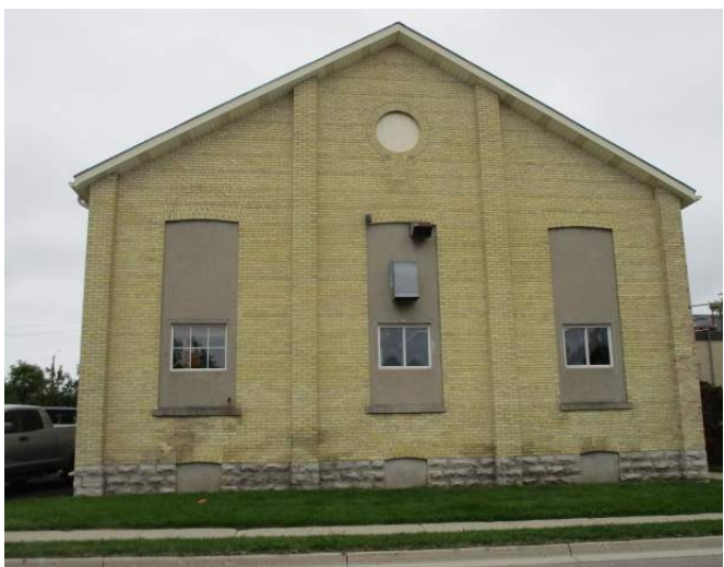
Original windows have been blocked in. Small, vinyl windows have been installed
