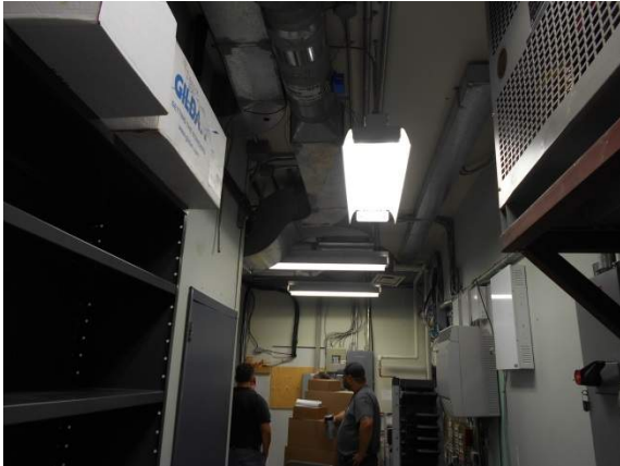
Ceiling Hung Light Fixtures.
