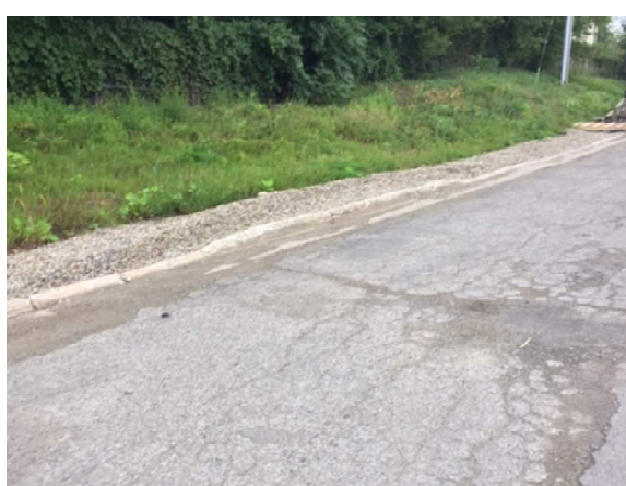
Deterioration in concrete curb
