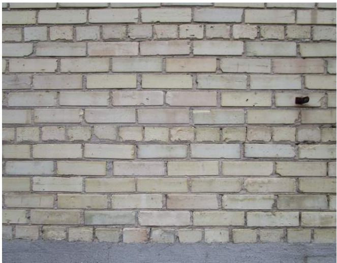
Brick masonry pattern, bonding course every 6 th row. Overall, masonry was found to be in good condition
