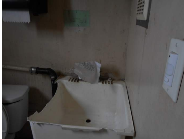
Broken washroom sink in truck bay washroom
