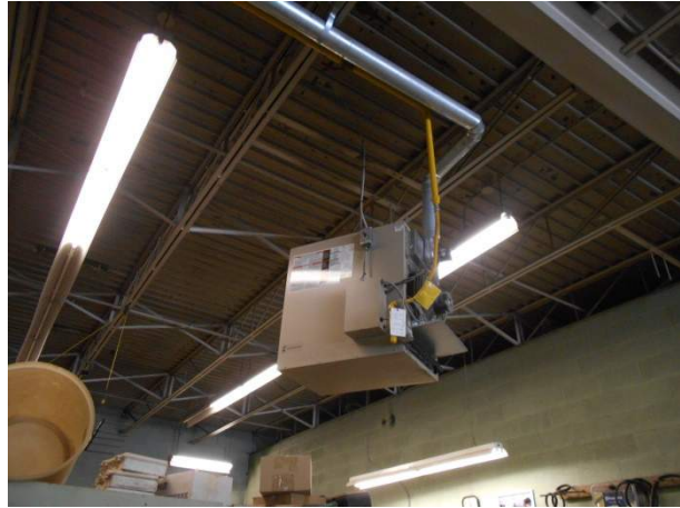
Unit heater in truck bay area
