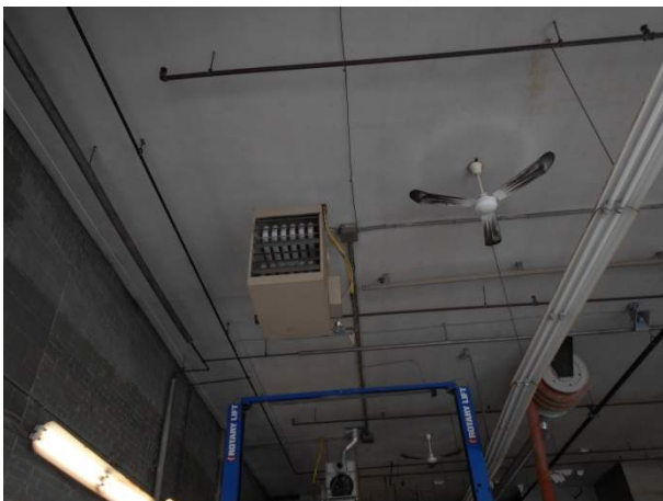
Unit heater and ceiling fan
