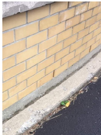
Efflorescence visible on wall
