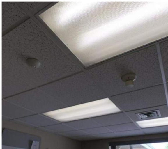
Heat and smoke detectors in addition
