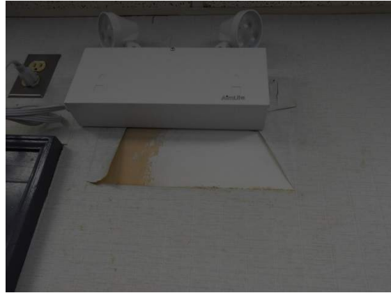
Emergency Battery with two Heads
