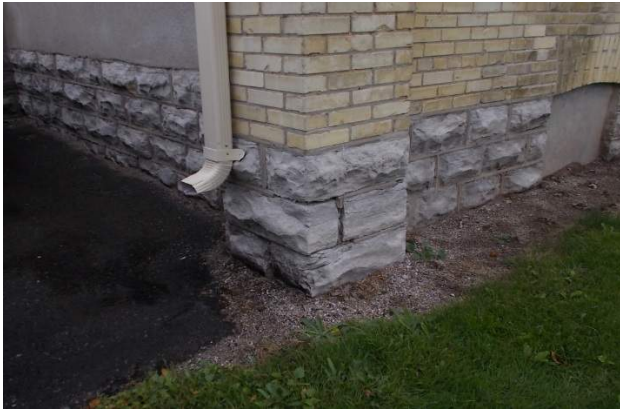
Missing mortar on stone block foundation of north truck bay building.
