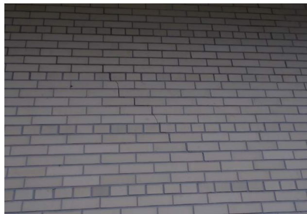
Step crack in exterior brick wall
