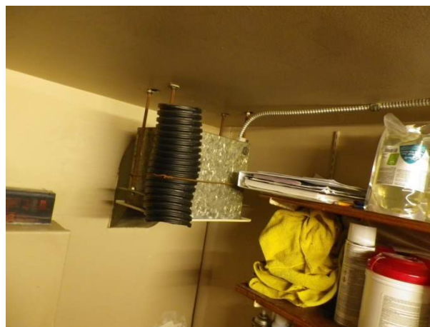
Janitors room exhaust fan on first floor
