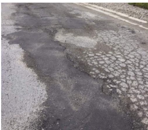
Deterioration in asphalt area north of building
