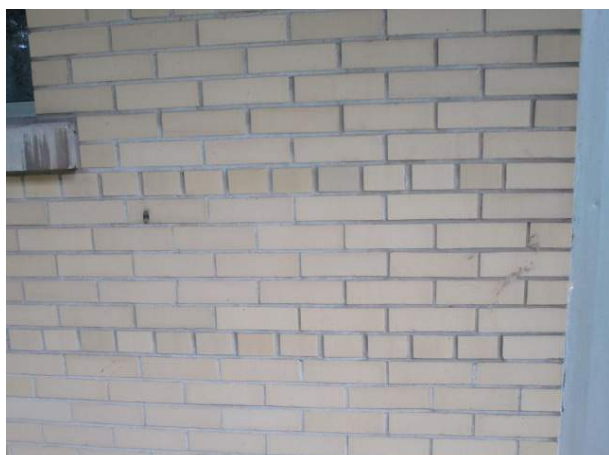
Overall view – brick masonry. Note bonding course every 6 th row of bricks.
