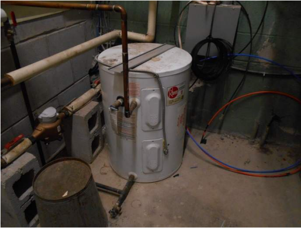
Domestic hot water heater in vault
