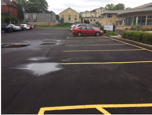
Longitudinal surface cracks and ponding in the north asphalt parking lot
