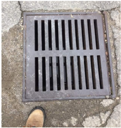
Storm Catch basin
