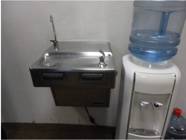
Drinking water fountain
