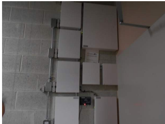
BAS / Security System control panels
