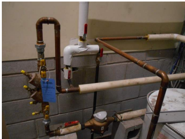
Domestic water meter and backflow preventer
