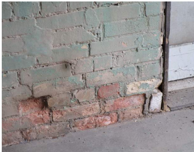
Tiny amount of masonry deterioration at the base of the door frame
