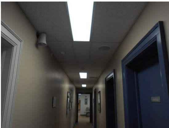
Ceiling mounted Speaker Smoke Detector and Horn
