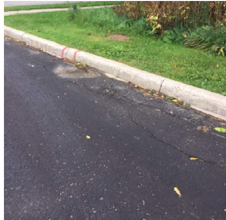
Longitudinal surface cracks in the east parking area
