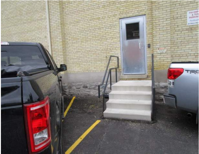
Upgraded, insulated metal door and frame installed in the 1920 section of the building
