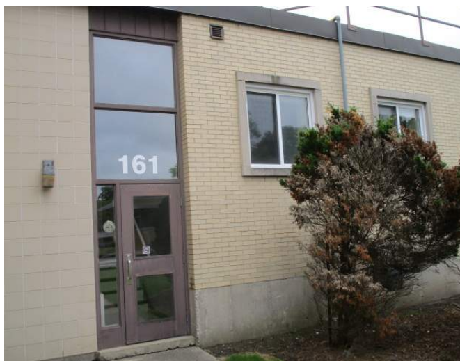
Original, entrance area to 1950's section of building. Original windows have been replaced with vinyl slider style windows.
