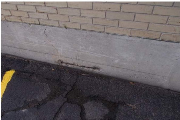
Spalled concrete at rebar.
