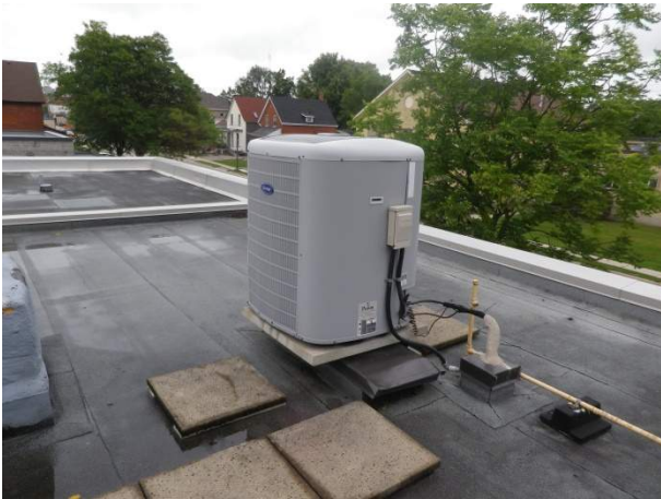
Fan coil condenser on roof
