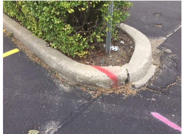
Area of deterioration on concrete curb
