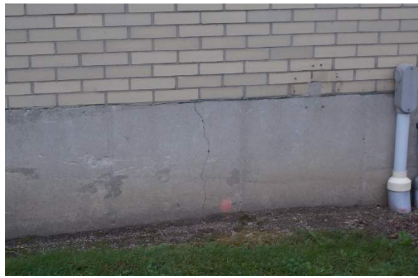
Cracking in foundation wall
