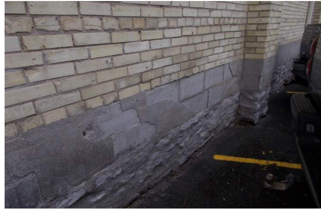
Stone rubble and concrete block with damaged parging on north truck bay building.
