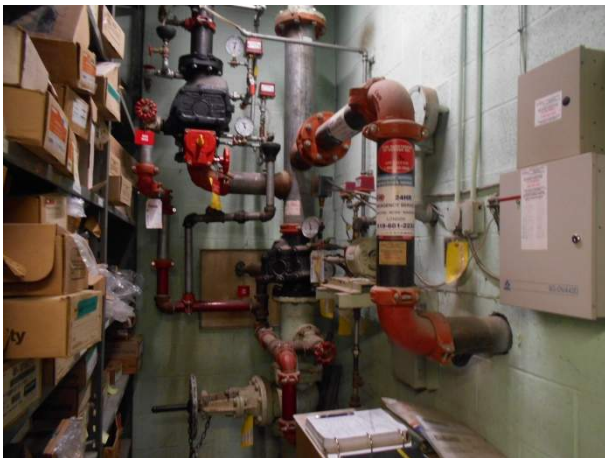
Fire sprinkler check valves
