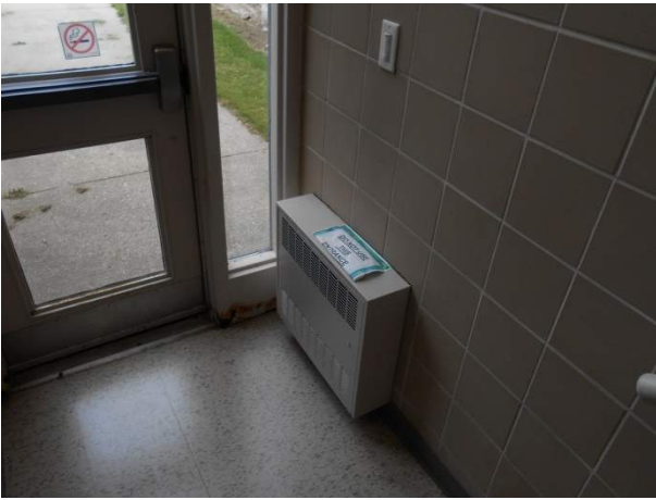
Cabinet heater in entrance
