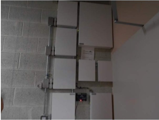
BAS / Security System control panels.
