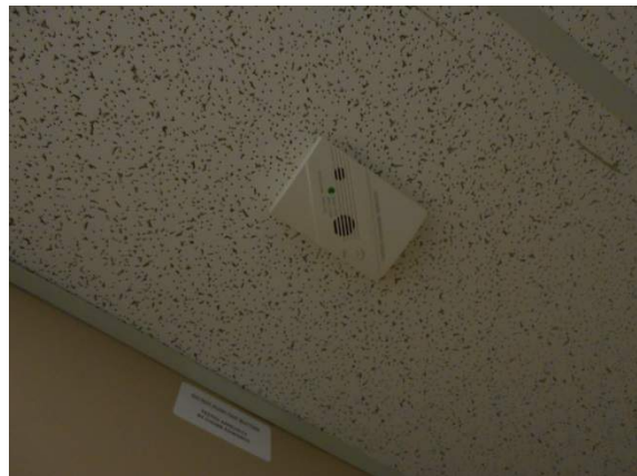
Ceiling mounted Motion Sensor
