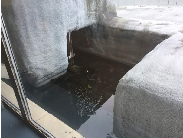
Ponded water at roof top unit.
