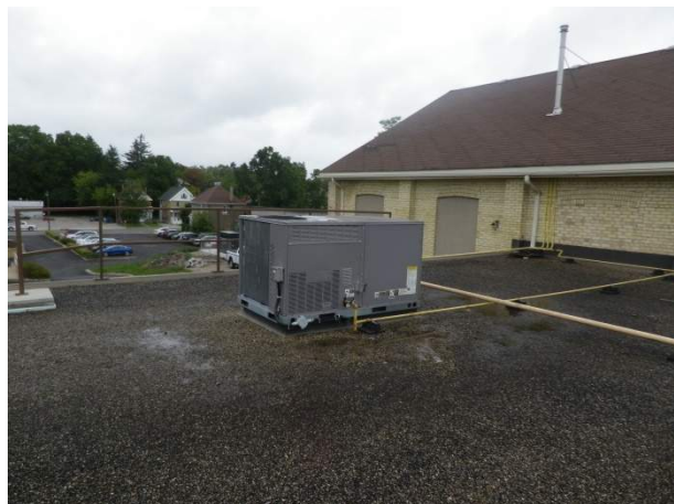
Rooftop unit serving office area
