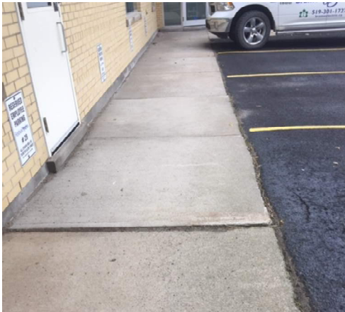
Area where settlement and heave is evident on concrete walkways
