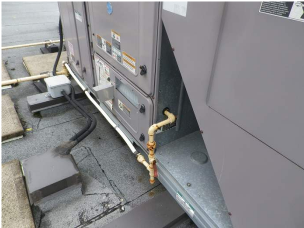
Rusty gas pipe connection
