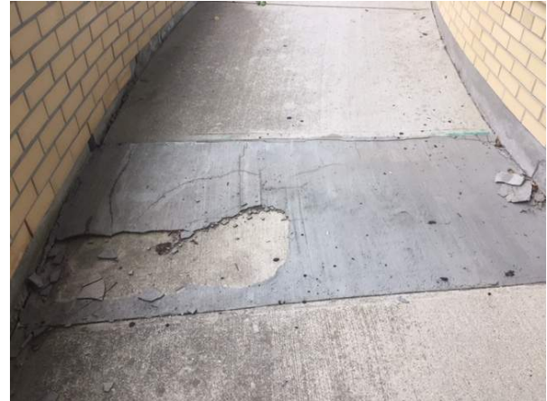
Area of deterioration on concrete walkway
