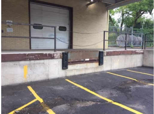
Deterioration in asphalt at loading bay
