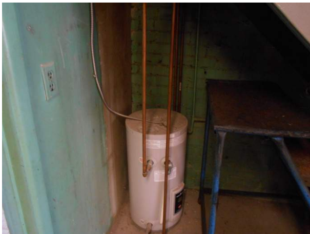
Domestic water heater in truck bay area
