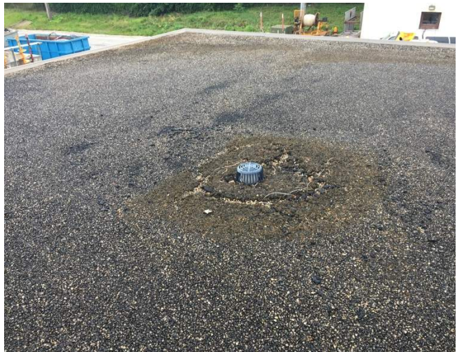
Debris at drain should be cleaned up to promote drainage of the roof.
