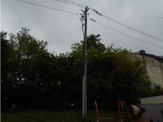
Main Incoming Service
