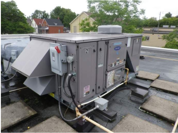
D3052 – Rooftop unit on high roof
