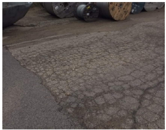
Deterioration in asphalt area north of building
