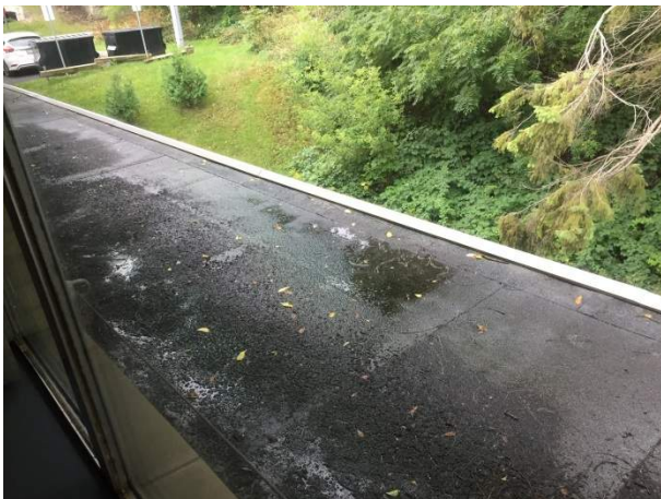
Lower canopy roof area – debris / low parapet
