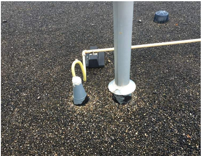
Roof cone for gas line, storm collar, well sealed with caulking
