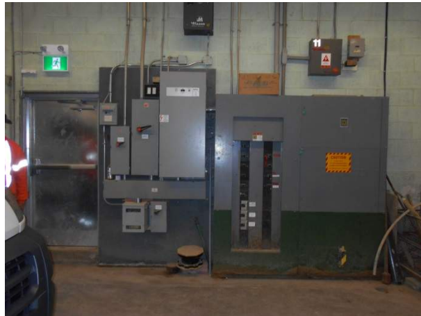
Main Distribution Panel and Transfer Switch
