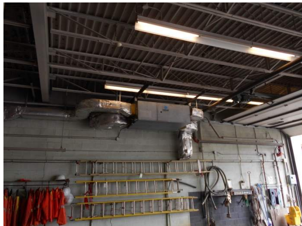
Heat recovery ventilator
