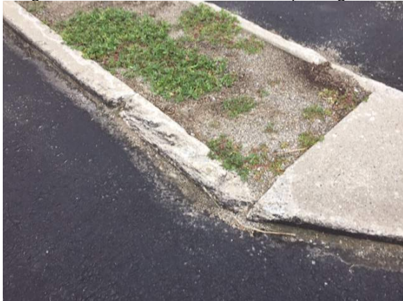
Area of deterioration on concrete curb
