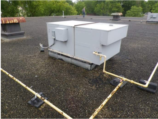
MUA unit serving large truck bay area
