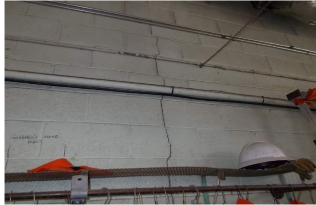
Crack in block wall of east truck bay building.
