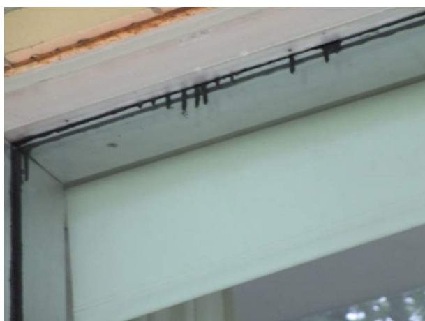
Glazing tape failure in original windows
