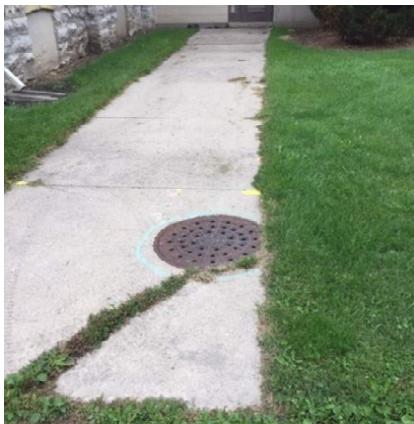
Area of deterioration on concrete walkway
