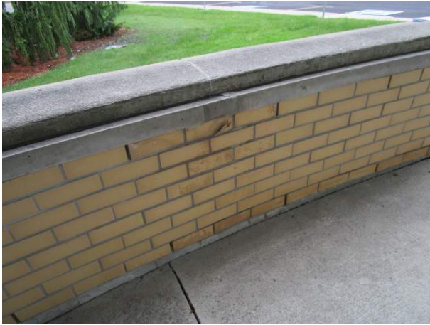
Tiny amount of brick deterioration – one brick.
