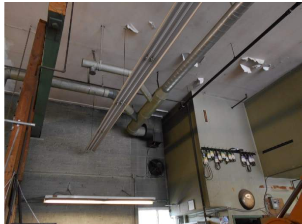
Two exhaust fans in truck bay area
