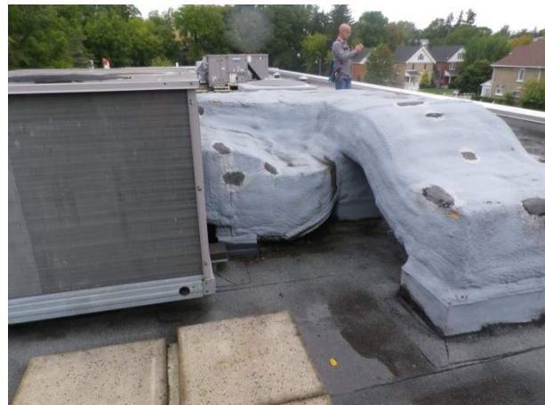
Exterior duct thermal insulation
