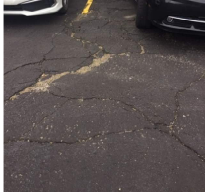
Deterioration in asphalt at loading bay
