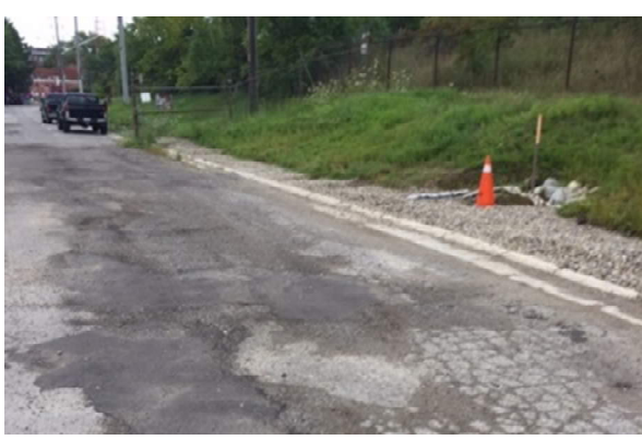
Deterioration in concrete curb
