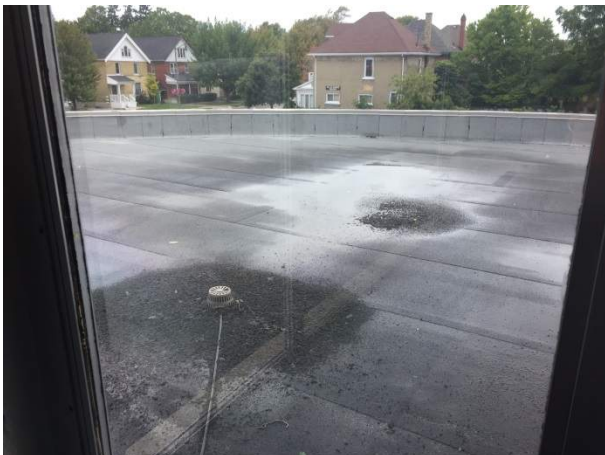
General view – low roof area – note debris at drain, ponding
