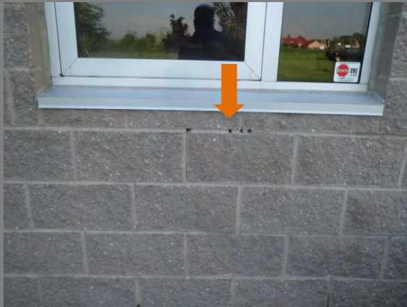
Repair: Minor holes in Masonry Location: West Wall
