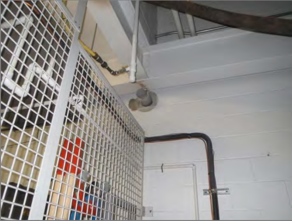
Repair: Abandoned penetration not sealed Location: Inventory Storage Room
