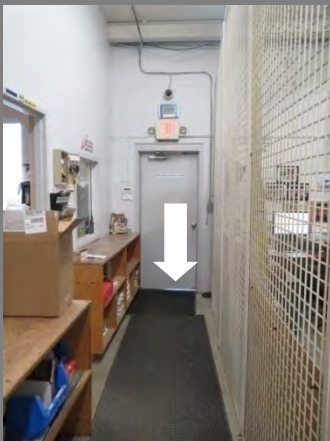
Repair: Weatherstripping missing Location: Shipping & Receiving
