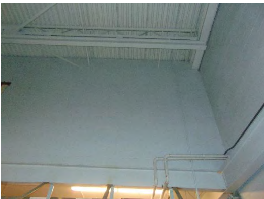
Possible Lateral stability issue Location: Storage Area
