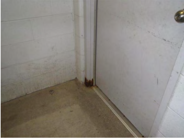
Repair: Door Frame starting to rust Location: Stair No 3
