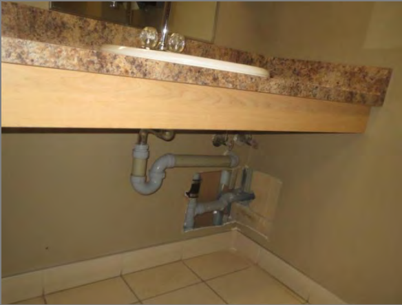
Partition Damaged due to plumbing repair Location: Office -Men's Washroom
