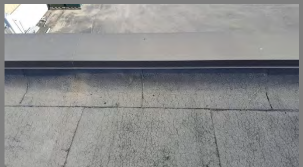
Roof inFair Condition – Cracking on surface Location: Over Second Floor Office
