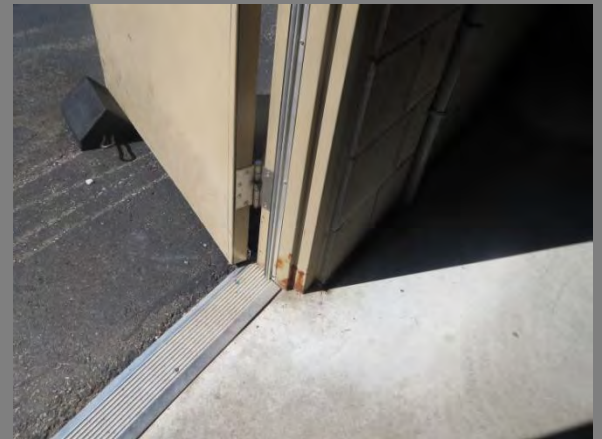
Repair: Door Frame rusting – frame does not fit masonry opening Location: Works Garage
