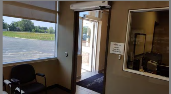
Door Operator In working Condition Location: Customer Entrance
