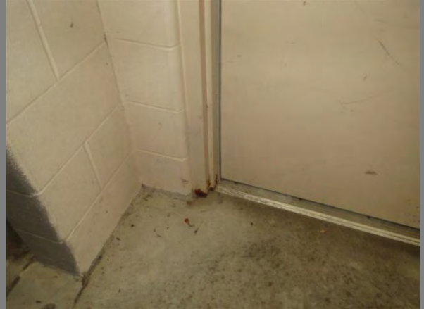
Repair: Door Frame starting to rust Location: Stair by Gym
