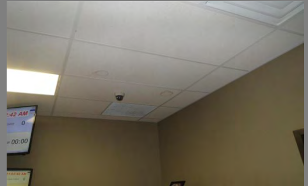
Sample: Ceiling tiles water damage Location: 1 storey First Floor
