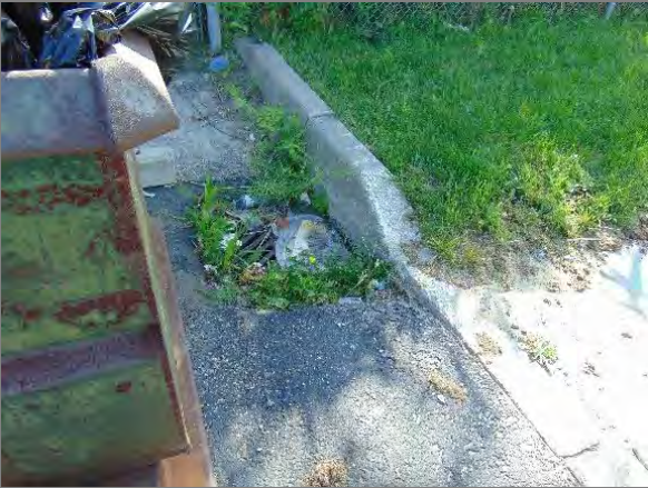
Catch Basin Settlement Location: North Service Area
