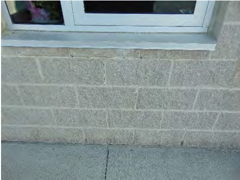
Cracking in Exterior Facade Location: South Wall
