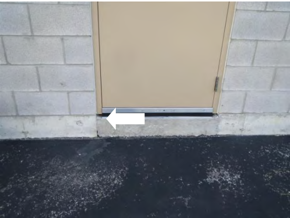
Repair: Frame does not suit masonry opening Location: Works Garage
