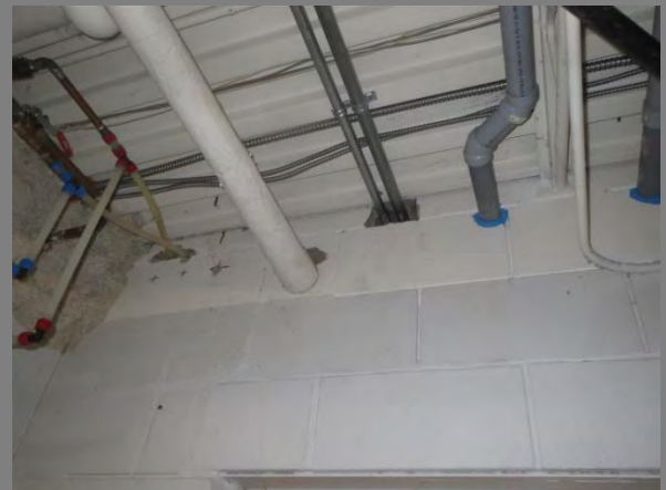
Penetration not fire caulked. Location: Mechanical Room
