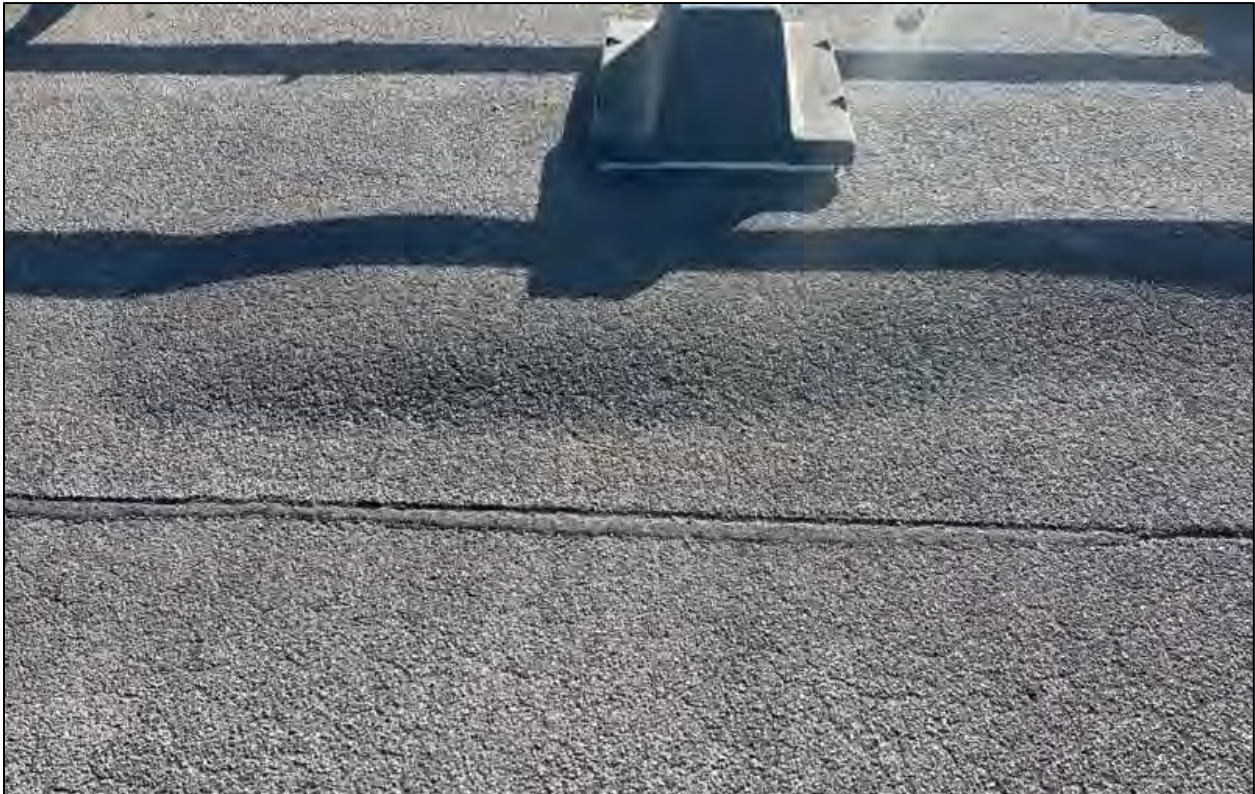
Blisters forming in roofing membrane
