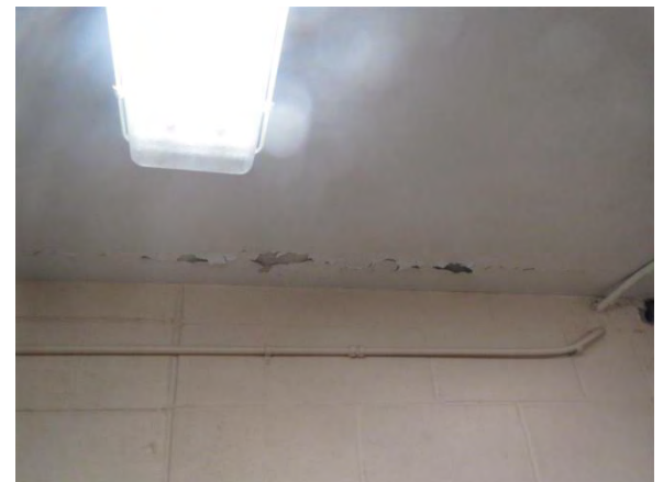
Repair: Paint peeling Location: Men's Shower | Change Room
