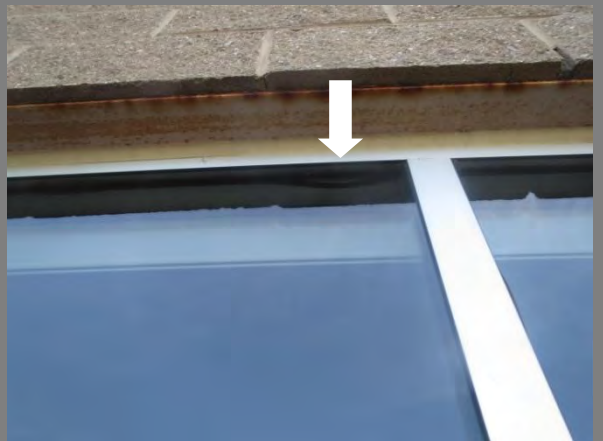
Repair: Gasket Failing and lintel rusting Location: west Wall
