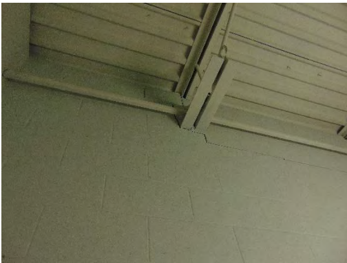
Cracking in Wall Location: North Stairwell
