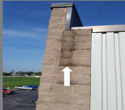
Monitor: Possible moisture intrusion Location: Front Entrance
