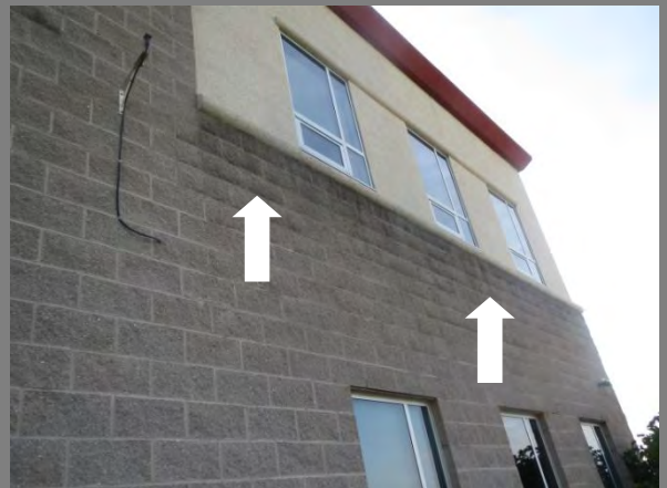
Monitor: Possible moisture intrusion Location: Southwest Wall
