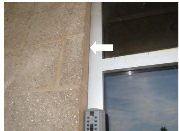
Repair: No Caulking around door frame Location: Employee Entrance
