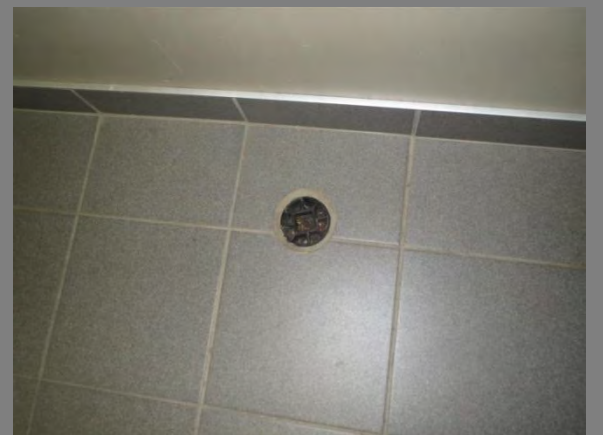
Sample- Cleanout missing cap – trip hazard Location: First Floor Kitchen
