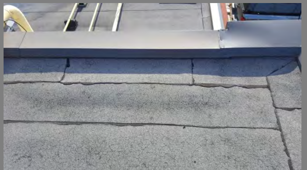
Roof starting to Bubble Location: One Storey Office Area - By Training Room
