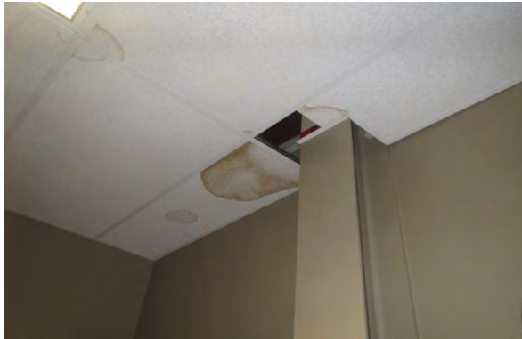
Sample: Ceiling tiles water damage Location: Office Space
