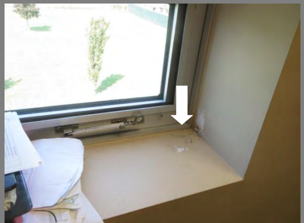
Repair: Window Leaking Location: Second Floor Office
