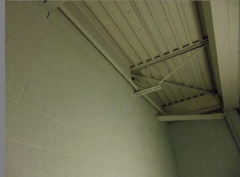
Cracking in Wall Location: North Stairwell
