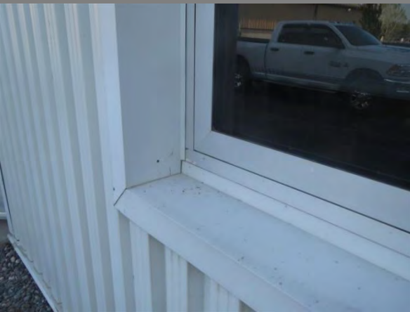
Sample: Window and Flashing in good condition Location: west Wall of Main Building
