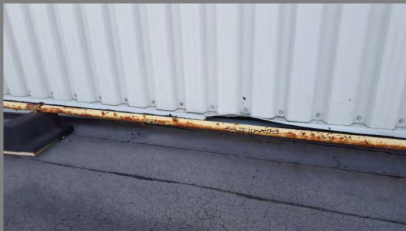
Rusted Counter Flashing at High Wall Transition Location: At Meter Shop – Office
