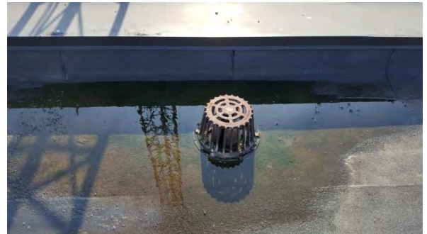
Roof Drain Clear – small ponding Location: Over Meter Bay
