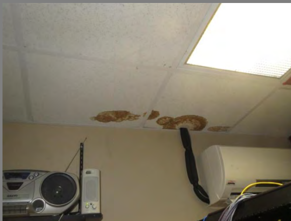
Sample- Ceiling tile damaged (condensation from HVAC Equipment) Location: Second Floor Communication Room
