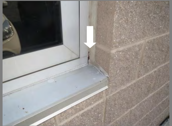
Repair: Caulking failing Location: Southwest Wall
