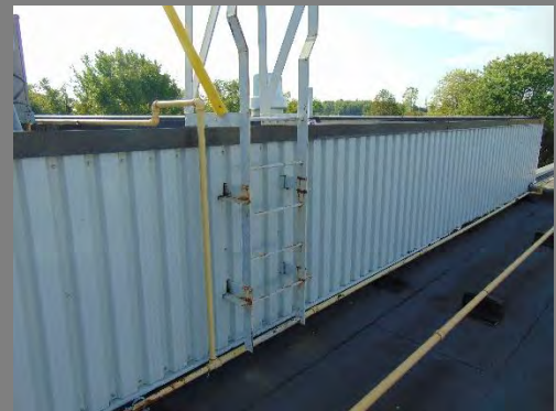
Typical Roof Ladder Location: Roof
