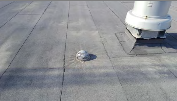
Exhaust fan c/w new seals on curbing Location: Over First Floor Office Area
