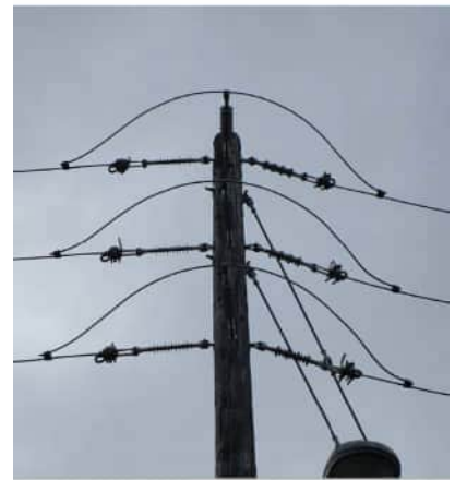
P11 (Existing Pole) – Overhead Conductors
