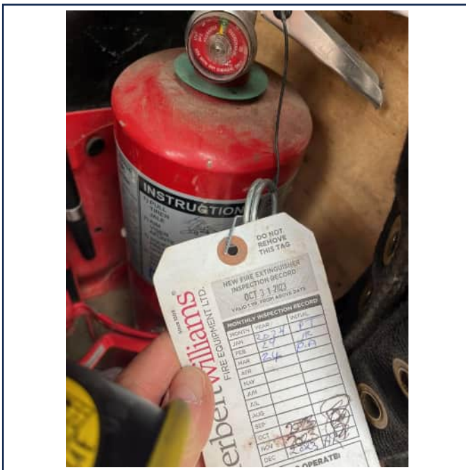
Fire Ext. Checked Fully Charged
