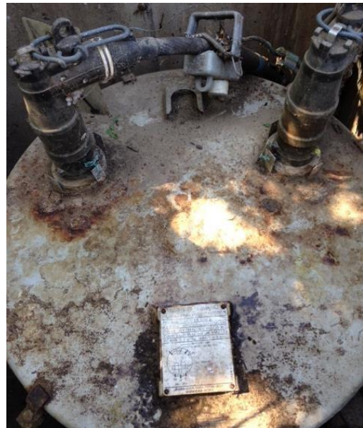
Figure 7: Corrosion on Top of a Transformer
