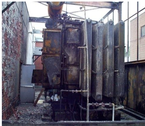
Figure 23: Damages to the MS Wall
