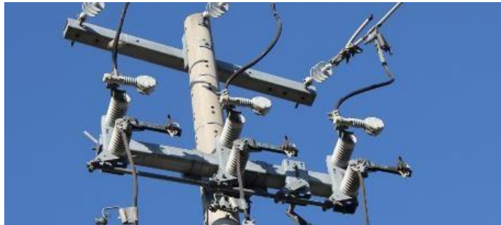
5 Figure 8: Manual Gang-Operated Switch
