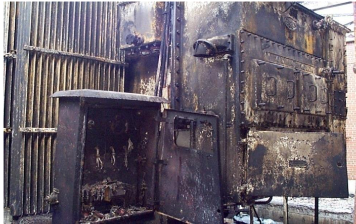
Figure 22: Failed Power Transformer
