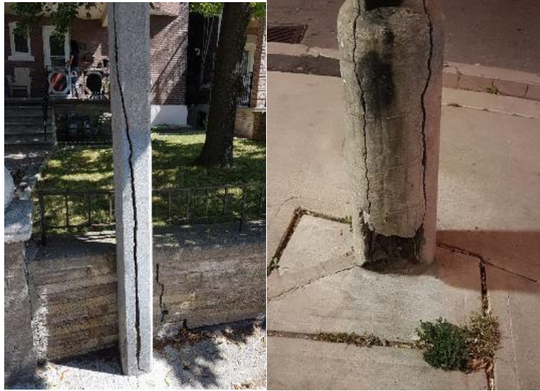
Figure 6: (Left) Longitudinal Crack on Pole, (Right) Cracked Concrete Base
