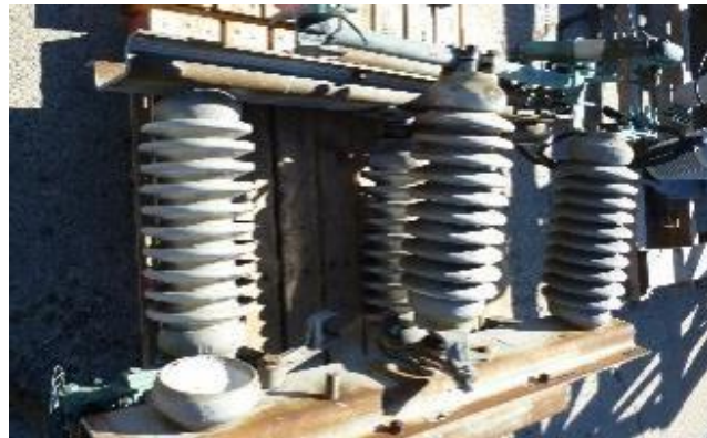
5 Figure 10: Broken Switch Insulator
