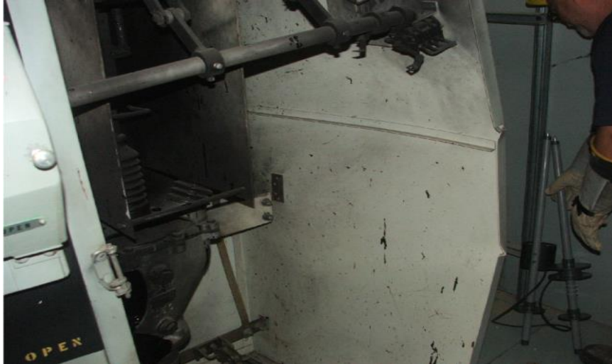
Figure 17: Impact of Internal Arc Fault in a Switchgear
