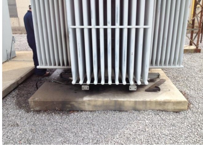
1 Figure 11: Oil Leak on a Station Transformer
