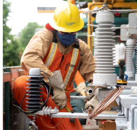
PLT - Overhead Plant
