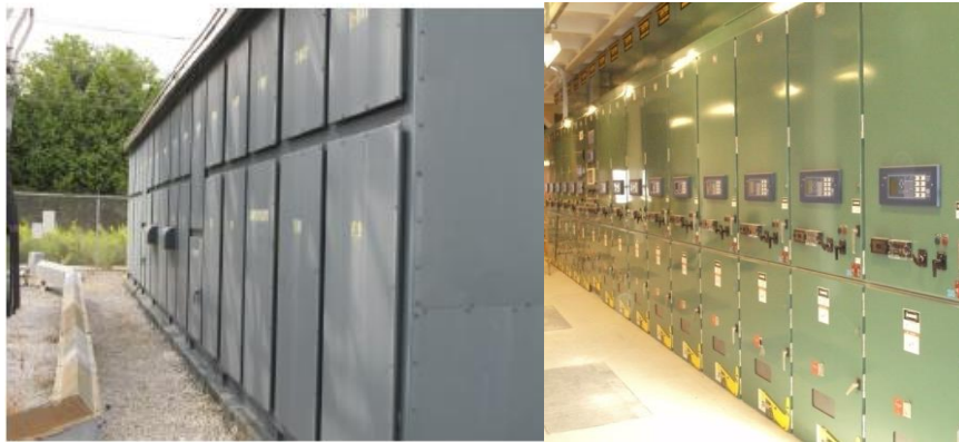
5 Figure 13: (Left) Outdoor Enclosure Housing Metal clad Switchgear. (Right) Indoor 6 Metal clad Switchgear
