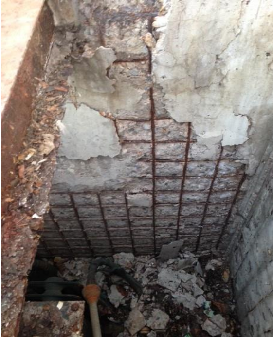
Figure 3: Crumbling Vault Roof with Exposed Rebar
