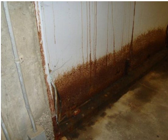
Figure 15: Rusted Switchgear Enclosure
