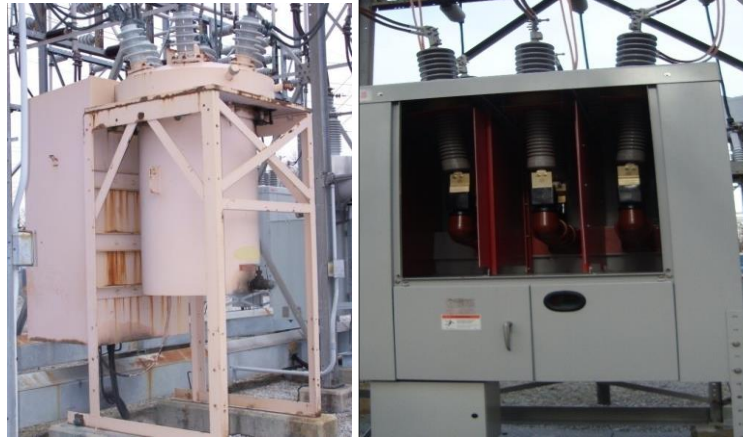
1 Figure 14: (Left) KSO Oil Circuit Breaker, (Right) Vacuum Circuit Breaker
