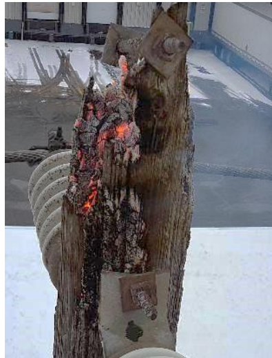
10 Figure 13: Pole fire on December 22nd, 2017
