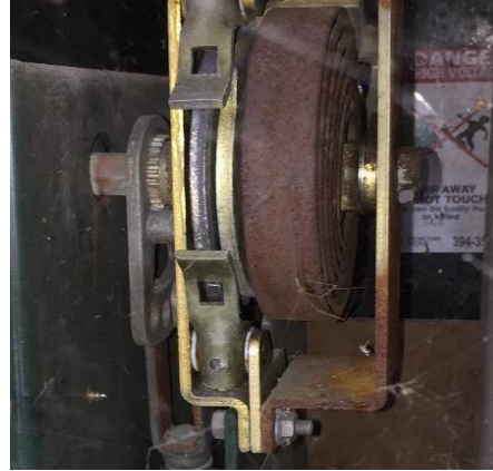
Figure 15: Padmounted Switch with Rusted Coil Spring
