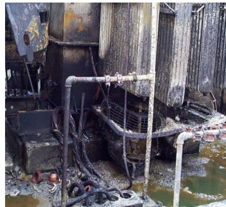
Figure 24: Leaking Fluids from Failed Transformer
