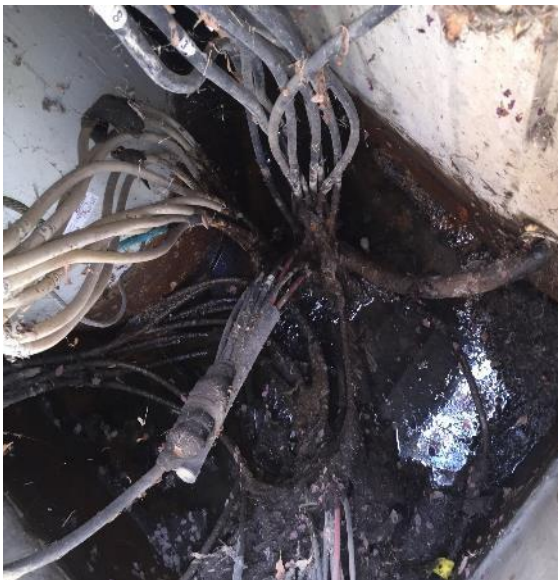
Figure 8: Oil Leaking from a Transformer Base Inside a vault
