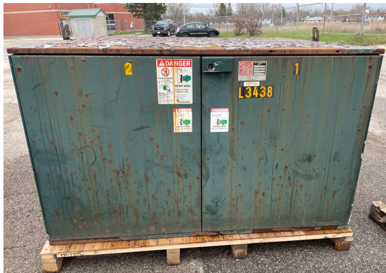
Figure 1 - PME switchgear that was removed from service due to excessive corrosion
