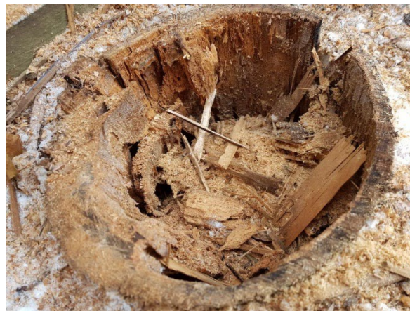
Figure 1 - Example of a hollow decayed pole that failed pole testing.
