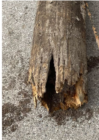
Figure 2 - Example of a decayed pole that failed pole testing and visual inspection.
