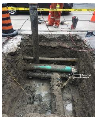
Figure 5.2-22: Leak investigation on vintage NPS 12 gas main
