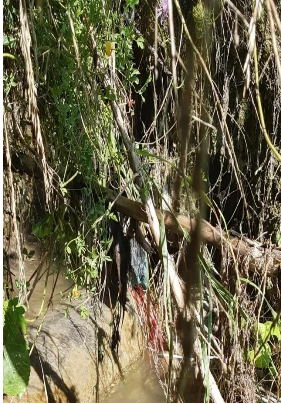
Figure 5.2-60: Exposed Pipe in Creek Crossing
