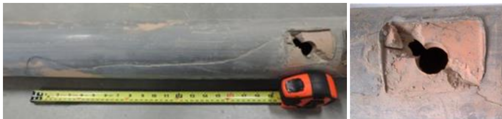
Figure 5.2-35: Rapid Crack Propagation on Aldyl A Pipe from Saddle Tee Fusion (Mississauga, ON)
