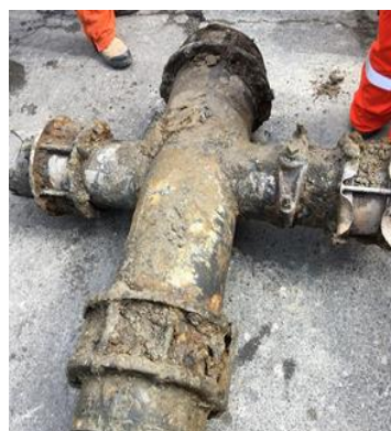
Figure 5.2-23: Detail of fabricated fitting after removal
