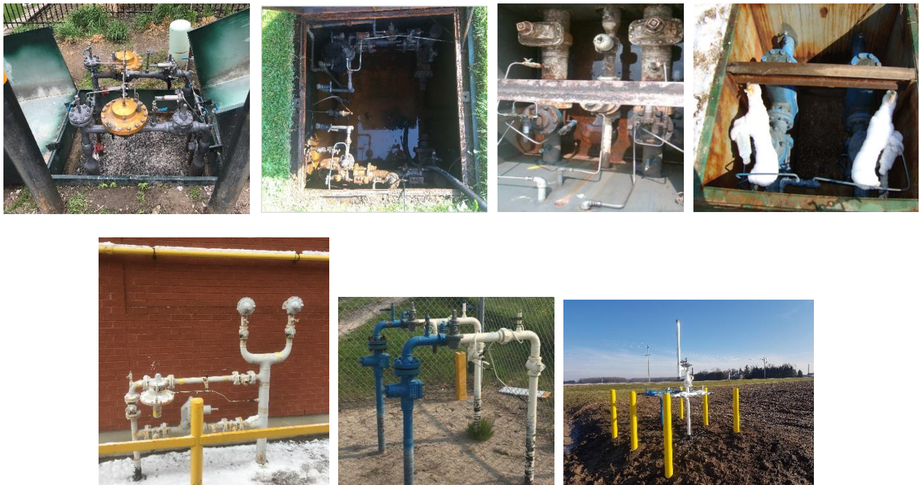
Figure 5.2-66: Examples of Distribution System Stations
