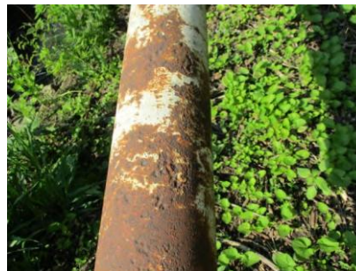
Figure 5.2-14: Coating degradation and corrosion pitting
