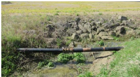
Figure 5.2-13: Aerial crossing with exposed mechanical fitting
