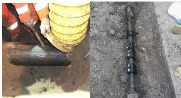
Figure 5.2-7: Bare and unprotected steel failures
