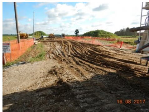
Aug 18 - P96 wet soils and ruts off the access ramp from hydrovac truck before mats installed
