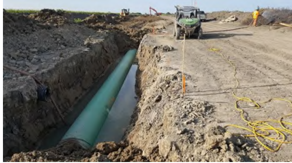
Aug 24 - P63 trench water sprayed onto topsoil piles causing minor eroding of soil
