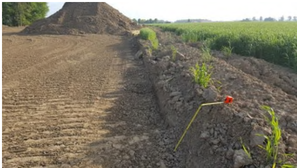
May 23 - P100 TLU topsoil stripping excessive with no separation of subsoil on topsoil pile
