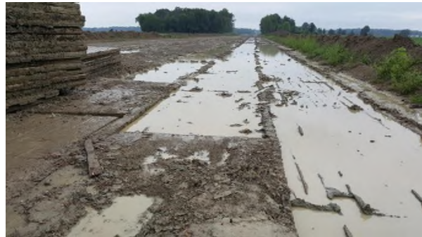
Aug 29 - P120 standing water on compacted subsoil after rain after wood mat lane removal
