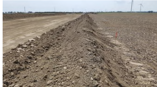
May 23 - P54 completed topsoil stripping of RoW into two piles, each with seconds pile at base
