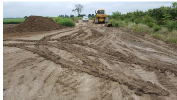
Aug 1/18 - P56 pickup turnaround tracks on wet soil just beyond mat lane
