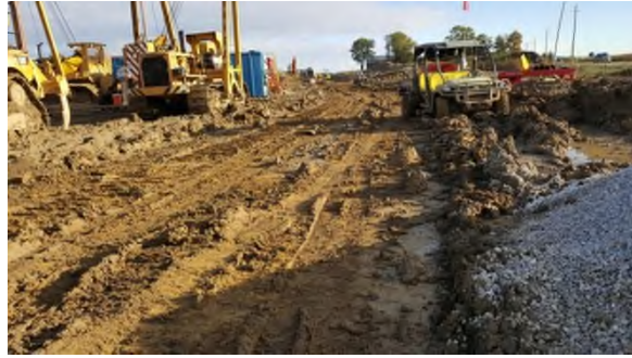
Oct 16 - P54 pipe work activity disturbance of drier subsoil after saturated subsoil pushed off
