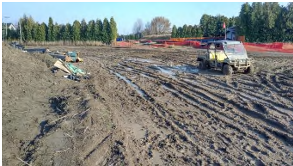
Nov 14 - P27 wet soil tracks from gator vehicle traffic during final construction activities
