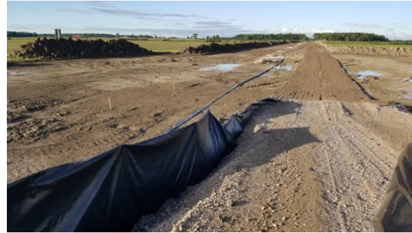
June 27 - P125 wood mat 4km lane covered in mud lying on wet clay soils and ponded water
