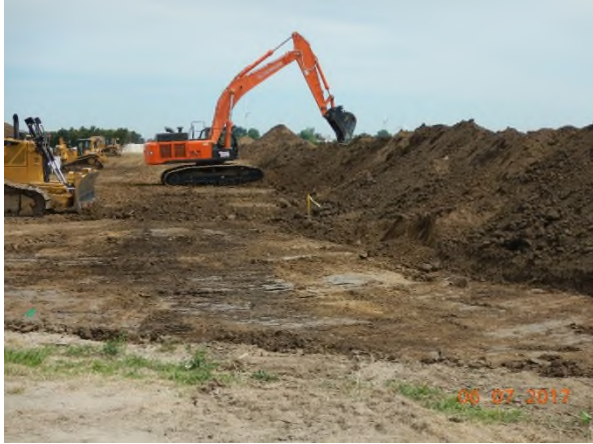
July 6 - P24 topsoil that spilled over the back of pile off easement being pulled back onto pile
