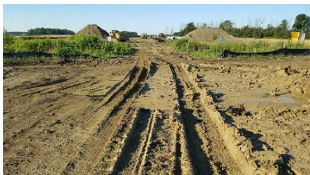
July 25 - P107 saturated subsoil pushed aside by bulldozer before rutted by fuel truck traffic
