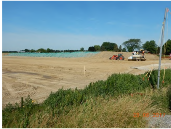
June 29 - P72 hydroseed spraying of topsoil piles in TLU of annual ryegrass on sandy soils
