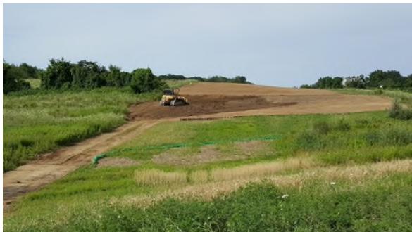
July 26 erosion features graded out and topsoil added though limited slope erosion protection
