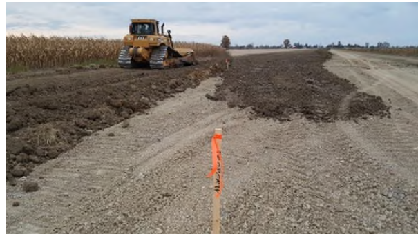
Oct 23 - P98 (SCN) and P97 (non SCN) boundary topsoil returned and separation maintained
