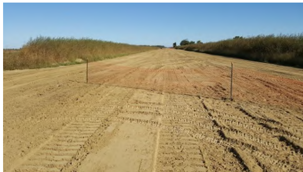
Oct 5 - P79 fenced off from fall soil restoration, several other sandy subsoils decompacted
