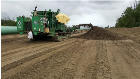
July 24 - P114 ditcher wheel making narrow trench and smaller subsoil pile, good separation
