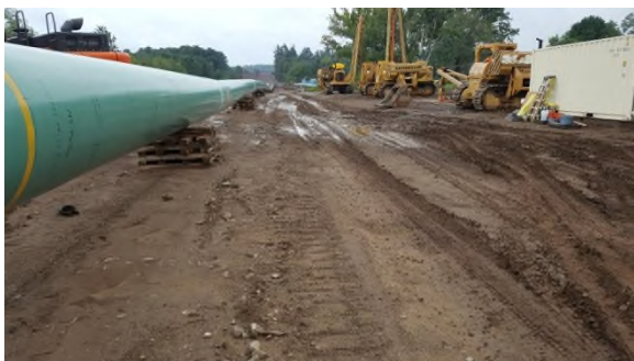
September 8 - HM38 traffic continued in wet soil conditions for water crossing activity
