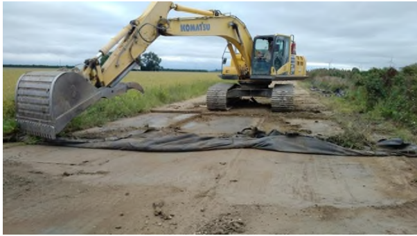
Sept 24 - P56 access lane mats and geotextile fabric lifting cleanly adjacent to Little Bear Creek
