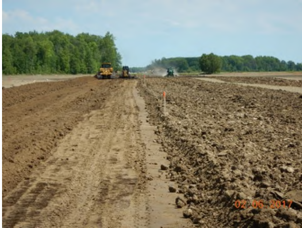
June 2 - P110 topsoil stripping sequence of discing, grader centre cut, bulldozer pushing windrow
