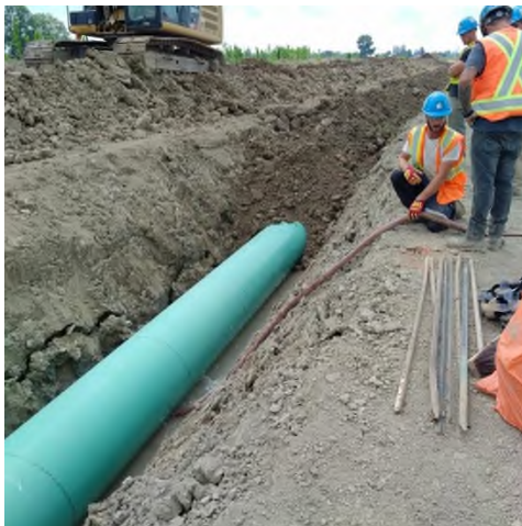
Aug 3 - P97 trench backfill using soft pile centre material first, deep heavy clay subsoil near top
