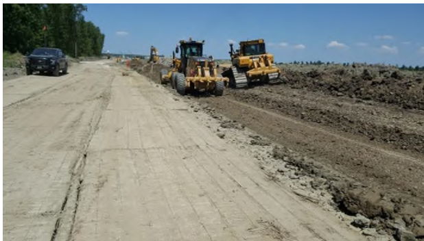
July 31 - P126 compacting subsoil material backfilled in trench using grader tires and bulldozer passes
