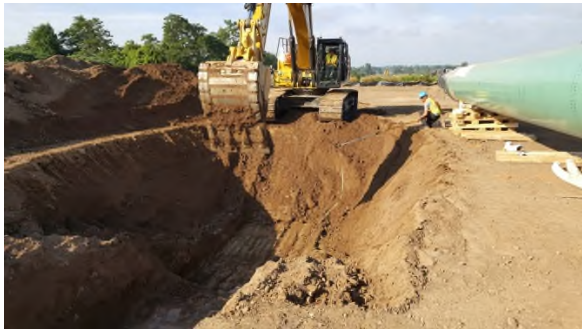
July 22 - HM40 trenching to proper depth checked regularly by suspended tape measure
