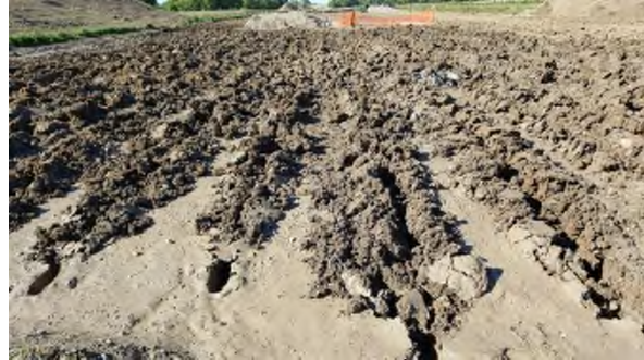
August 29 - HM44 ripper penetrated wet subsoil to aerate causing smearing, not decompaction
