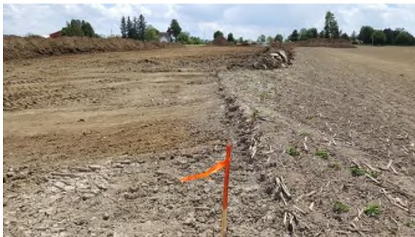
May 30 - P97 (non SCN) and P96 (SCN) boundary topsoil stripped toward SCN impacted property
