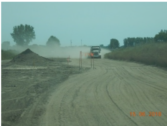
June 15 - P5 travel area of RoW dusty, beaten subsoil from dump truck traffic removing subsoil
