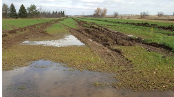
December 7 - HM45 tile installation trenches and compaction after completing in wet soil conditions
