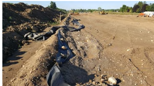
Aug 18-HM39 backfill completed after separating subsoil from pile barrier and grading level
