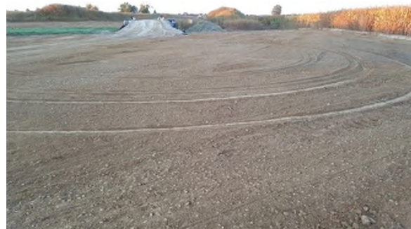
Oct 5 - P82 gravel remaining from stockpile graded out and mixed into subsoil surface
