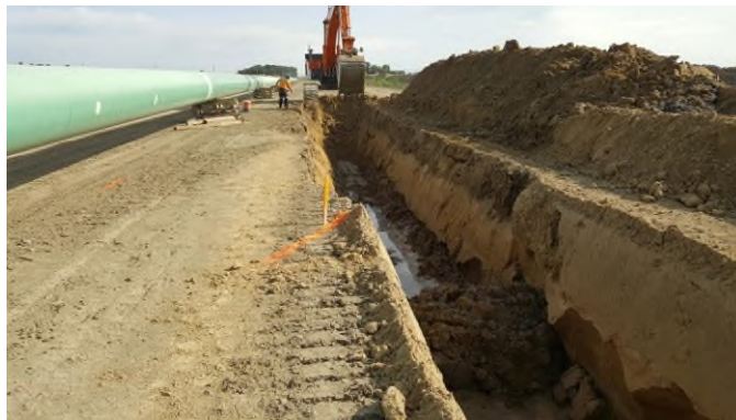
Aug 24 - P52 trench wall and pile size comparison of wheel trencher (foreground) and excavator bucket
