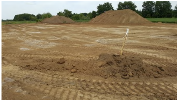
August 15 - HM36 topsoil piles of darker (back) and lighter colour from different stripping depths
