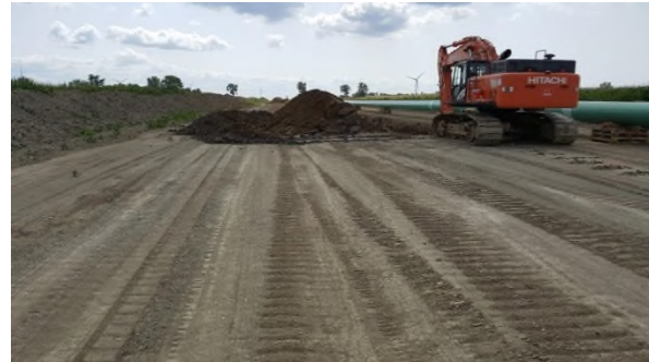
Aug 25 - P47 backhoe trenching separating heavy clay from deep trench into rear subsoil pile
