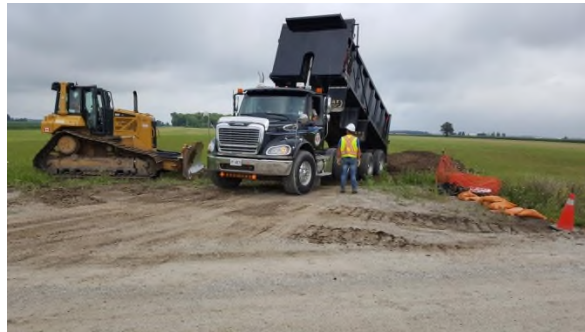
Aug 8 - P99 dumping unscreened topsoil at field edge and temporary piling beside low wet soil
