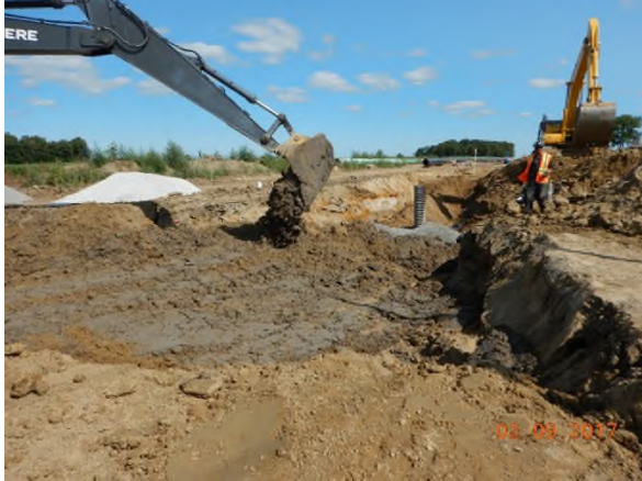
Sept 2 - P54 backfill of deep bell hole generally dry but wet mixed soil materials placed on top
