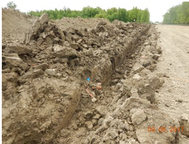
June 9 - P124 trenching of 16in. pipeline and capping of tile drains (blue) as they are excavated
