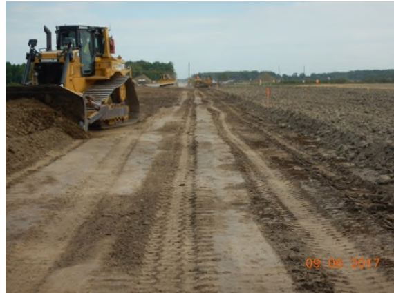
June 9 - P109 grader has made first cuts and bulldozer continues to strip topsoil
