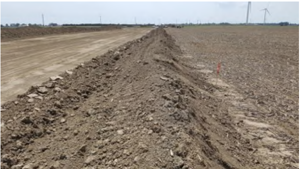
May 23 - P54 completed topsoil stripping of RoW into two piles, each with seconds pile at base
