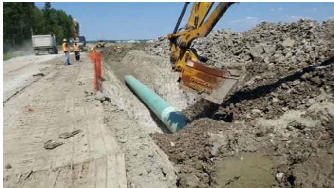
July 31 - P126 backfill over pipe using grinder bucket to break up hard clay soil clumps
