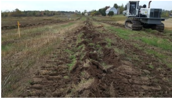
October 11 2017 - HM36 tile installation in dry to moist conditions with little compaction
