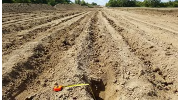
August 29 - HM46 decompaction of dry subsoil to 35cm using a bulldozer mounted ripper
