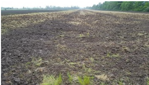
June 5 - HM44 uneven surface in area of tile drainage installation and trench line
