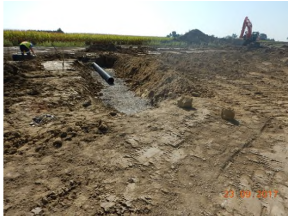
Sept 23/17 -P47 main drainage tile repair in progress under predominantly dry conditions
