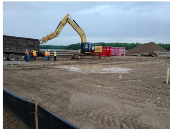
June 15 - P110 loading 16in. pipe scrap in wet soil conditions without sufficient matting
