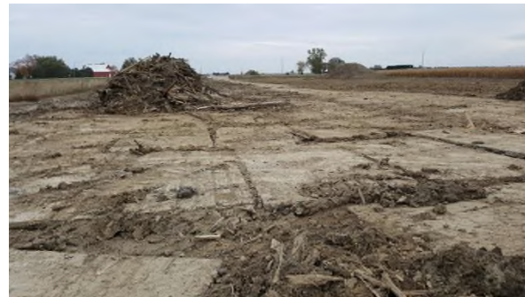
Oct 23 - P56 clean-up of bore site where broken construction wood mat pieces mixed into subsoil
