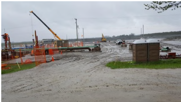
May 4 - P1 pipe work traffic and activities in TLU area in wet soil conditions
