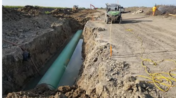
Aug 24 - P63 trench water sprayed onto topsoil piles causing minor eroding of soil
