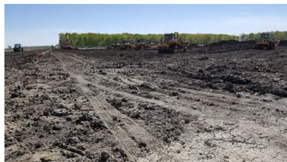
May 15 - P128 topsoil stripping using ten heavy machines done too early on moist clayey subsoils
