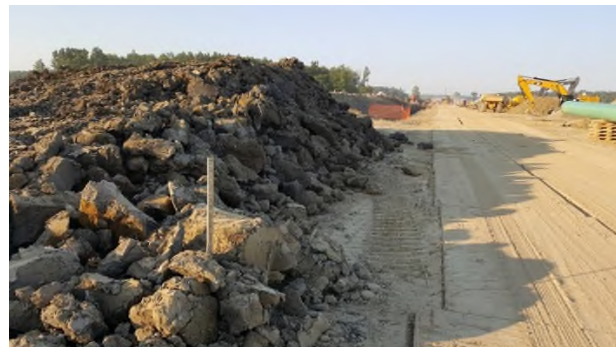
Aug 1 - P118 blue clay piled and signed separately to be hauled off site
