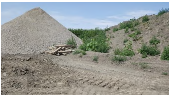
Sept 7 - P61 gravel stockpiled over topsoil seconds pile and onto topsoil pile
