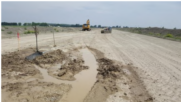
June 18 - P69 pumping standing water off RoW including into main tile after filter bag
