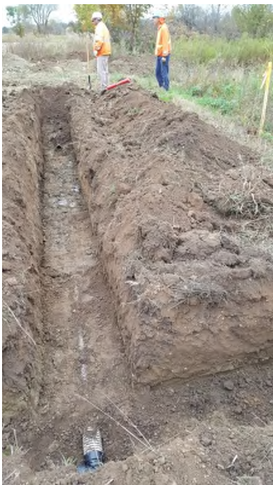
October 11 - HM36 tile main missing across trench line exposed for repair
