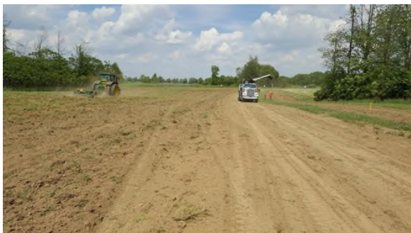
June 2 - HM33 topsoil disced under pile area to the right of the yellow stakes marking existing pipeline
