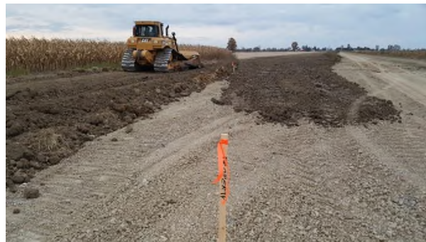
Oct 23 - P98 (SCN) and P97 (non SCN) boundary topsoil returned and separation maintained
