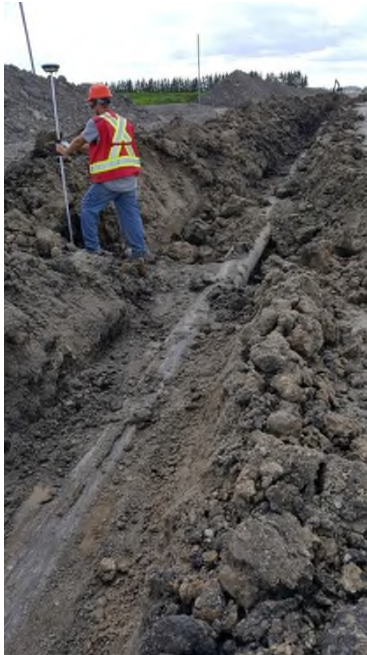
June 26 - P66 georeferencing lateral tile intercepted during trenching of 16in. pipe line
