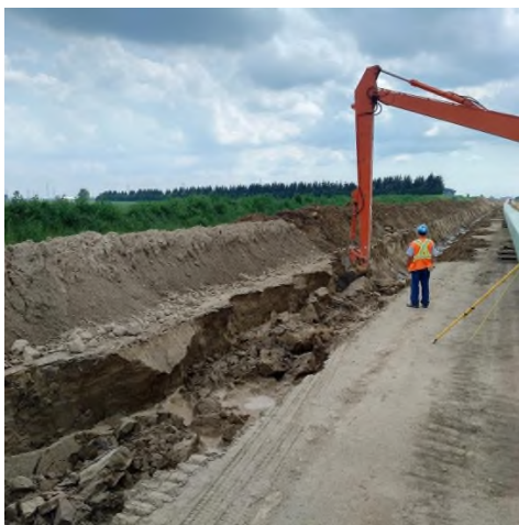
Aug 15 - P79 trench deepened after sidewall collapse of coarser soil material
