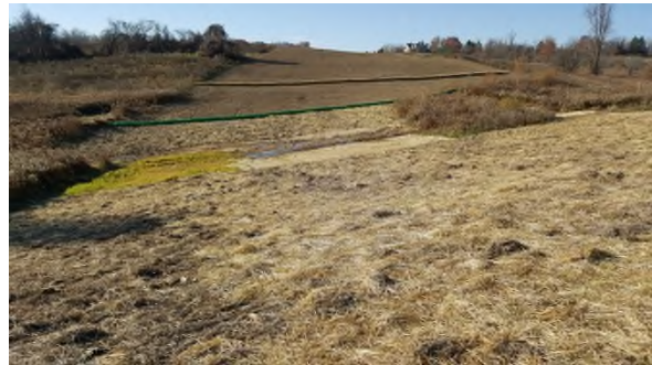
November 14 erosion sediment protection of creek but not for soil loss from susceptible slope
