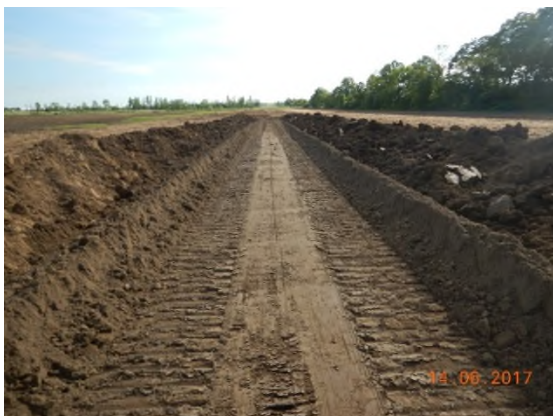
June 14 - HM44 topsoil stripping along low area of trench line and importing topsoil to mix
