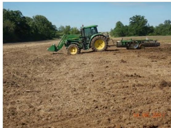
June 14 – HM44 angled tractor tilling surface across easement near tile install and trench line
