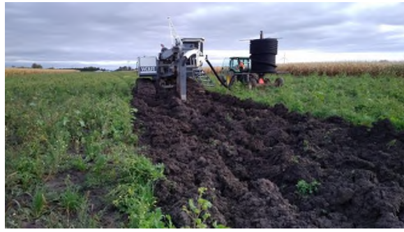
Oct 11 - P23 tile plow installation in very moist soil conditions causing severe rutting and mixing
