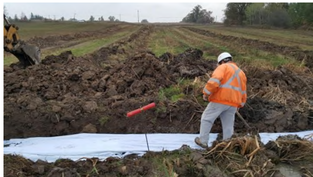
October 14 - HM40 wet area from damaged tile getting repaired with blind tile inlet
