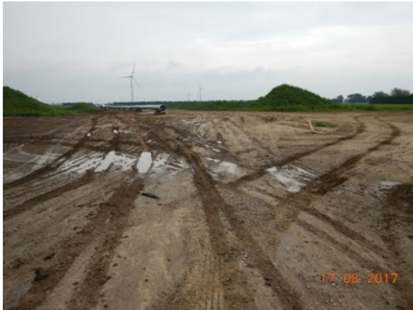
Aug 17 - P33 random pickup truck traffic in wet soil and through standing water
