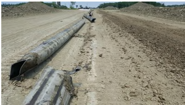
June 13 - P111 16in. pipe removed and snipped beside trench left for pickup and loading off site
