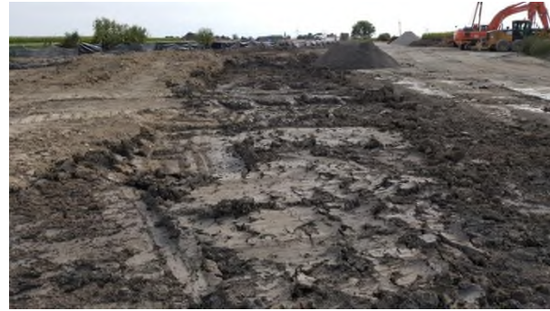
Sept 12 - P61 tie-in trench backfilled to top with deep trench clay vs. original sandy loam subsoil
