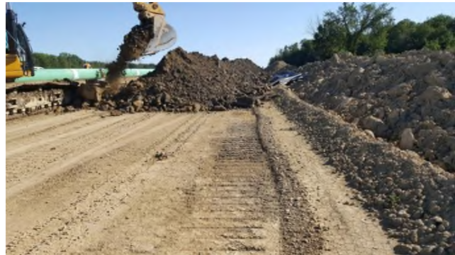
July 25 - P113 insufficient space to pile subsoil requiring geotextile separation with topsoil pile
