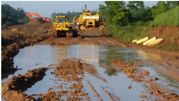
August 26 - HM31 heavy equipment driving through standing water for water crossing work
