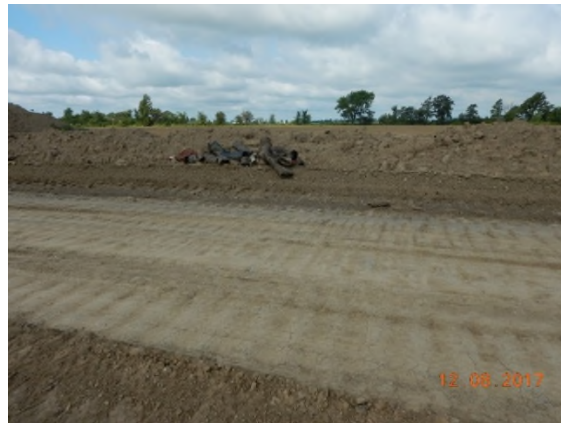
Aug 12 - P103 clean-up of plastic tile drain from subsoil during backfilling operations
