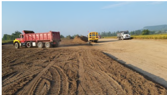
September 7 - HM46 dump trucks used to load out rock from water crossing turning on topsoil
