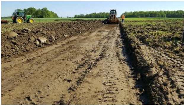
May 29 - P121 topsoil stripping initially by grader to proper depth separating undisturbed topsoil
