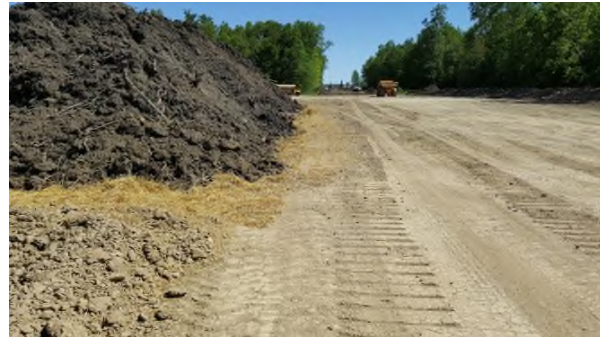
June 7 - P121 TLU area where topsoil from P122 woodlot stored on hay mulch layer
