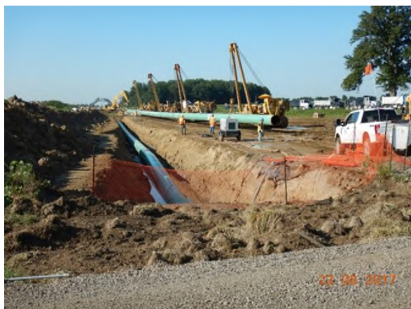
Aug 23 - P89 typical extent of open trench before pipe lowering-in operations and backfilling
