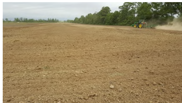
June 15 - HM44 restored grade of easement after importing topsoil and extensive leveling
