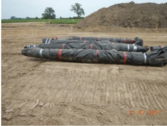
July 21 - P23 asbestos coated 16in. pipe encased in geotextile material for proper disposal
