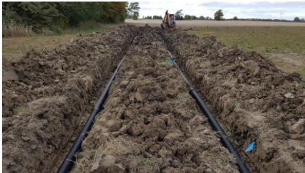
Oct 24 - P55 replacement of flattened main tiles with hard tile sections across easement
