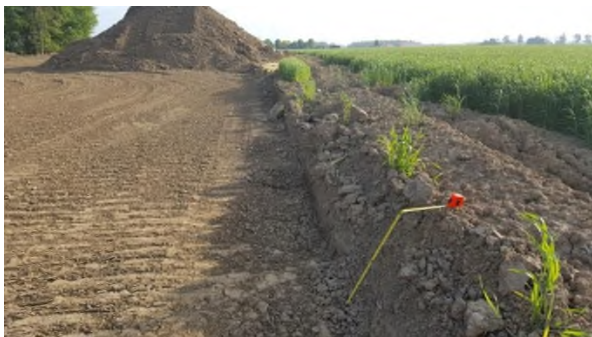
May 23 - P100 TLU topsoil stripping excessive with no separation of subsoil on topsoil pile
