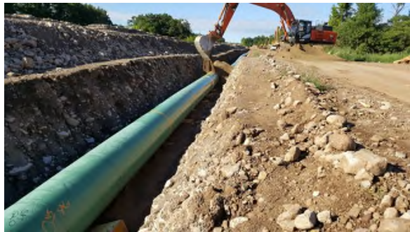
August 22 - HM30 extensive use of imported sand to cover pipe displacing bouldery subsoil
