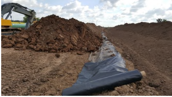
July 18 - HM48 trench subsoil piled on geotextile material separating from transition layer pile
