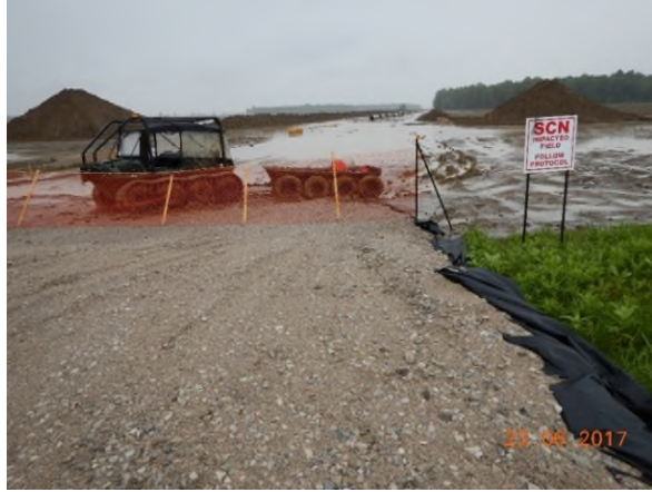
June 23 - P111 ponded water and tracks made by an Argo ATV transporting pump equipment
