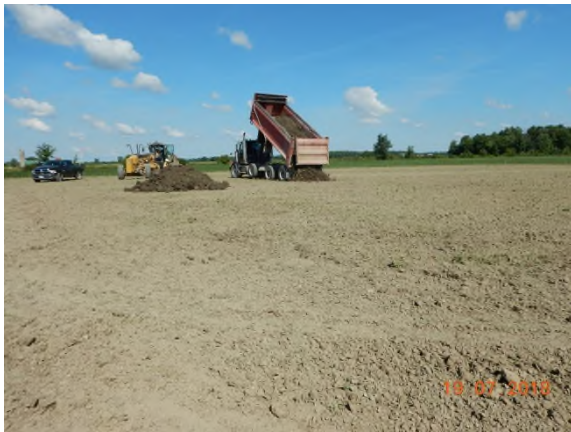
July 19 - P124 topsoil addition to low areas after disc and grader worked and levelled dry surface
