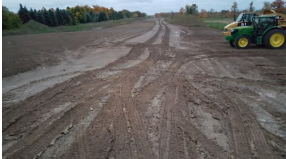
October 24 - HM30 truck tracks on wet subsoil from hauling extraneous material off easement
