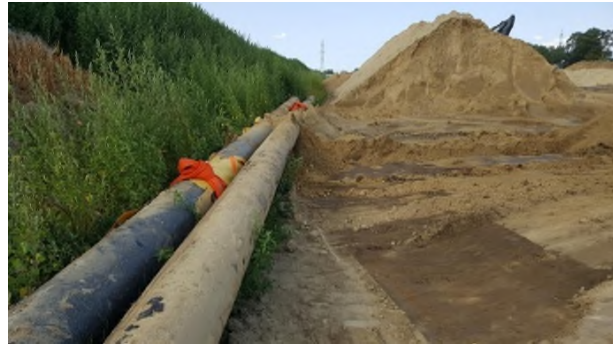
Aug 25 - P74 temporary storage of 16in. pipe, and subsoil, encroaching on topsoil seconds pile
