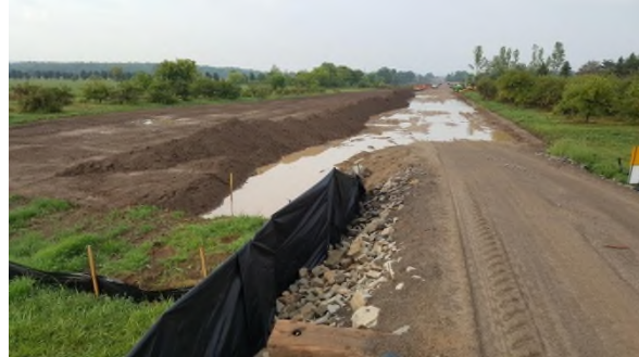
September 8 - HM45 wet soil shutdown from wet soil and standing water on driveway subsoil
