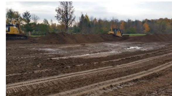
November 2 - HM38 topsoil being returned onto wet subsoil prior to subsoil decompaction
