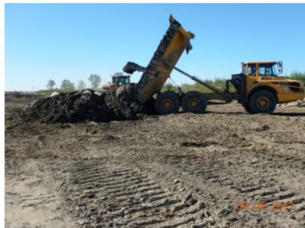
Sept 30 - P8 rock truck dumping excavated material on RoW from road and drain crossing
