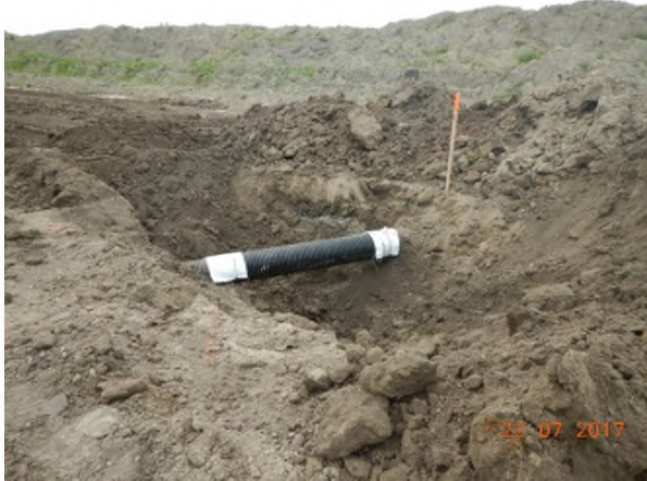
July 21/17 - P9 typical repair of plastic tile drain main completed during backfilling
