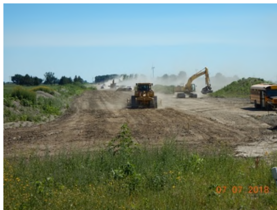
July 7 - P60 subsoil decompaction ripping and leveling under very dry good conditions
