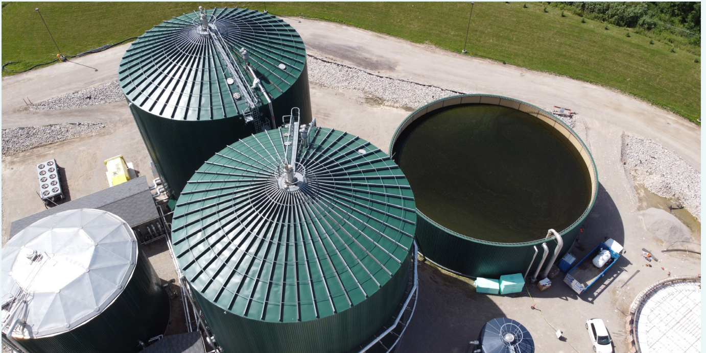
Biogas Digesters at StormFisher's London Biogas Facility.
