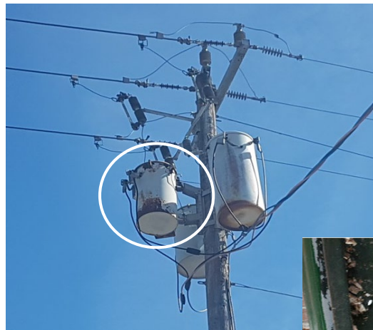
Rusted tanks (OH and UG)
