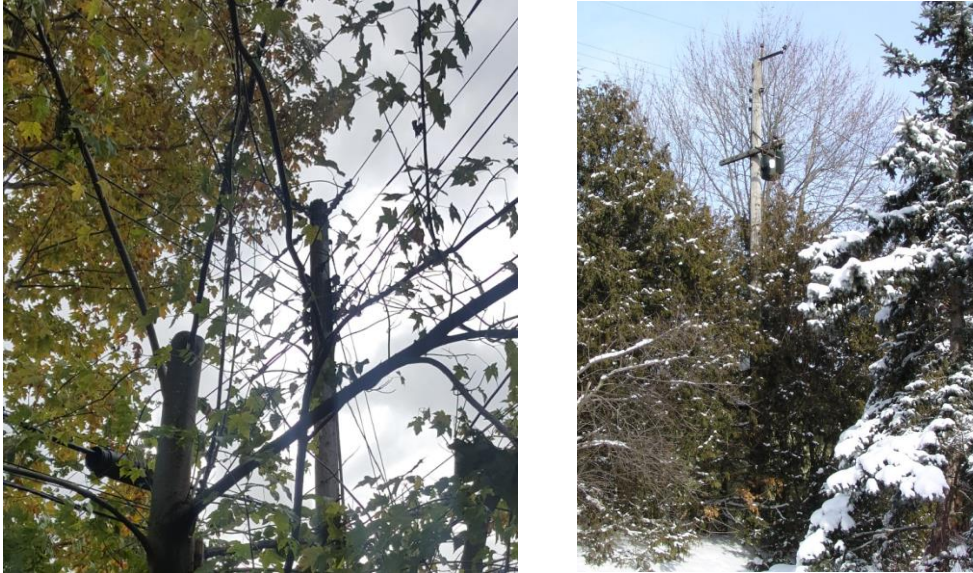
Figure 24: Excessive vegetation in close proximity of distribution equipment
