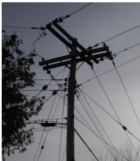
Figure 26: Reduced safe work clearances due to an outdated construction standard
