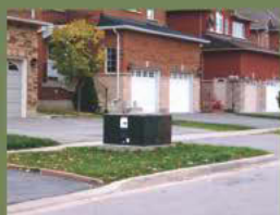
Pad mounted transformer
