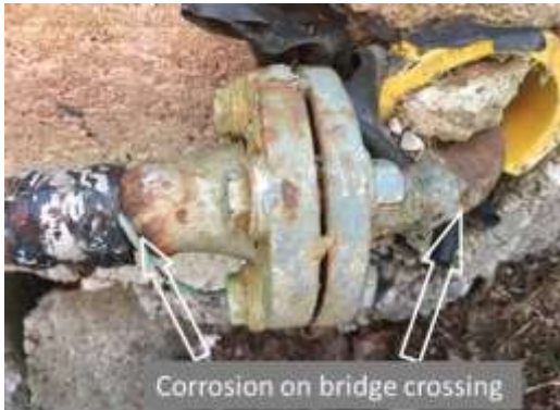
Figure 5.2-7: Severe corrosion on bridge crossing pipe
