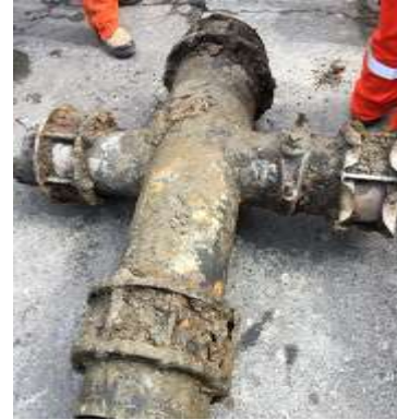
Figure 5.2-16: Detail of fabricated fitting after removal
