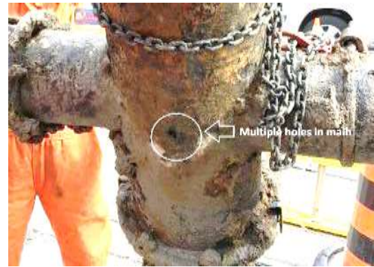
Figure 5.2-18: Multiple leaks on vintage NPS 12 gas main
