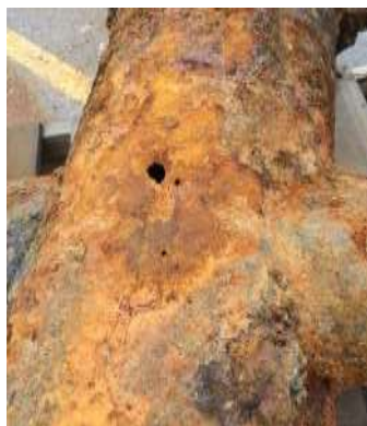
Figure 5.2-17: Multiple leaks due to severe corrosion on vintage NPS 12 gas main
