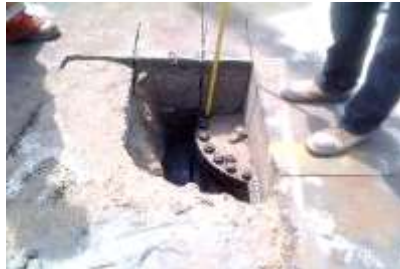
Figure 5.2-21: NPS 20 KOL shallow cover due to road grade changes
