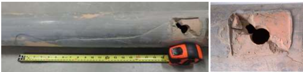
Figure 5.2-41: Rapid crack propagation on Aldyl A pipe from saddle tee fusion (Mississauga, ON)
