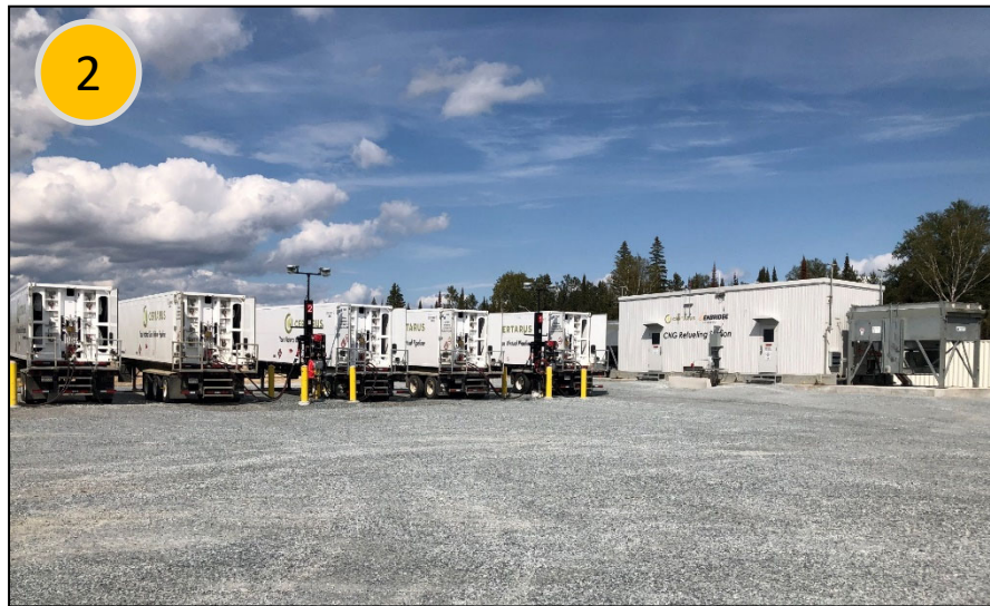
Source From Timmins, Ontario Certarus Permanent Facility
