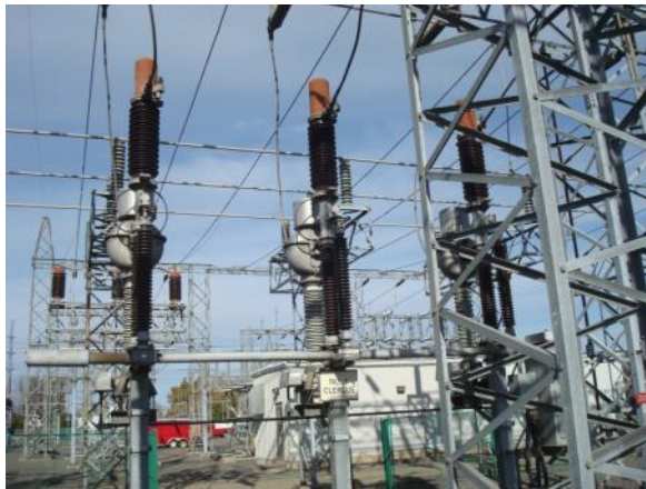
Figure 12-1: Steelton TS View 1
