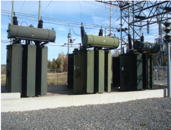
Figure 10-1: Goulais TS Transformers
