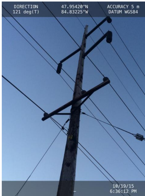
Figure 12-1: Magpie Transmission Line
