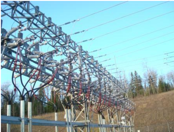
Figure 4-1: Watson TS High Voltage
