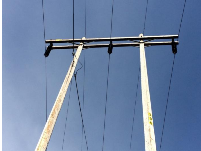
Figure 3-3: No.3 Sault Structure with Porcelain Insulators
