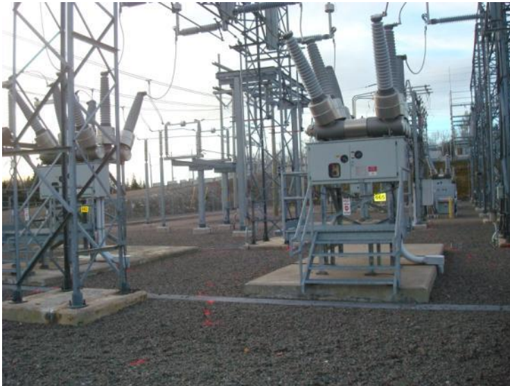
Figure 6-1: MacKay TS 115kV Circuit Breaker
