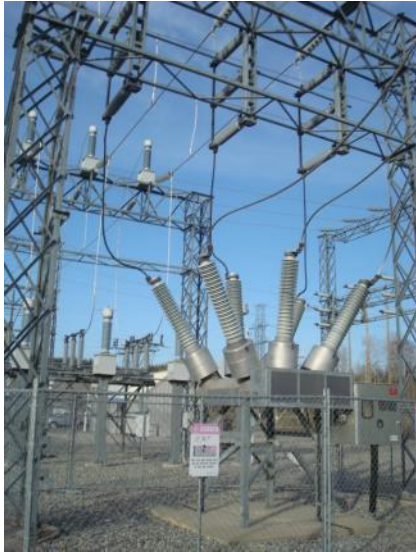
Figure 3-1: Anjigami TS Circuit Breaker
