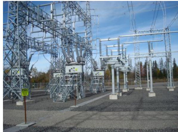
Figure 11-2: Third Line TS 115kV Circuit Breaker
