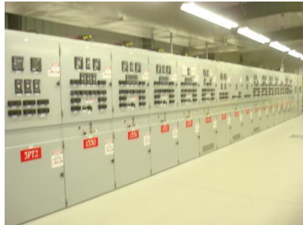
Figure 4-2: Watson TS Indoor Switchgear
