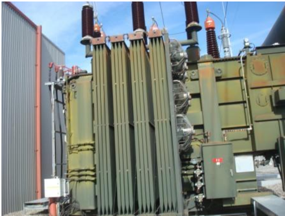
Figure 11-1: Third Line TS 230kV Transformer
