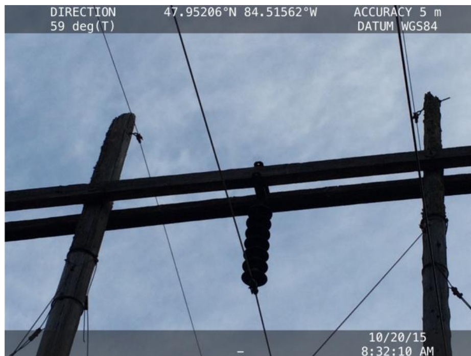
Figure 10-1: Hollingsworth Transmission Line
