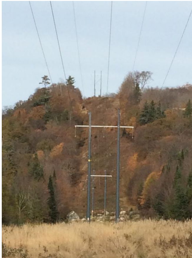
Figure 9-1: Hogg Transmission Line
