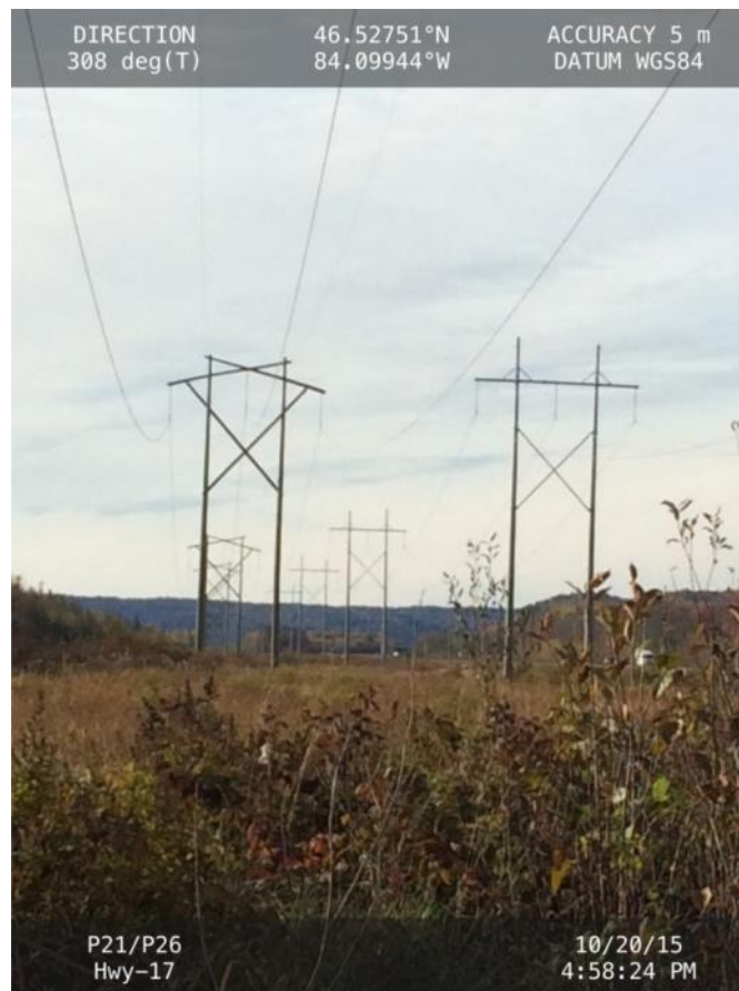
Figure 4-1: P21G and P22G Transmission Lines
