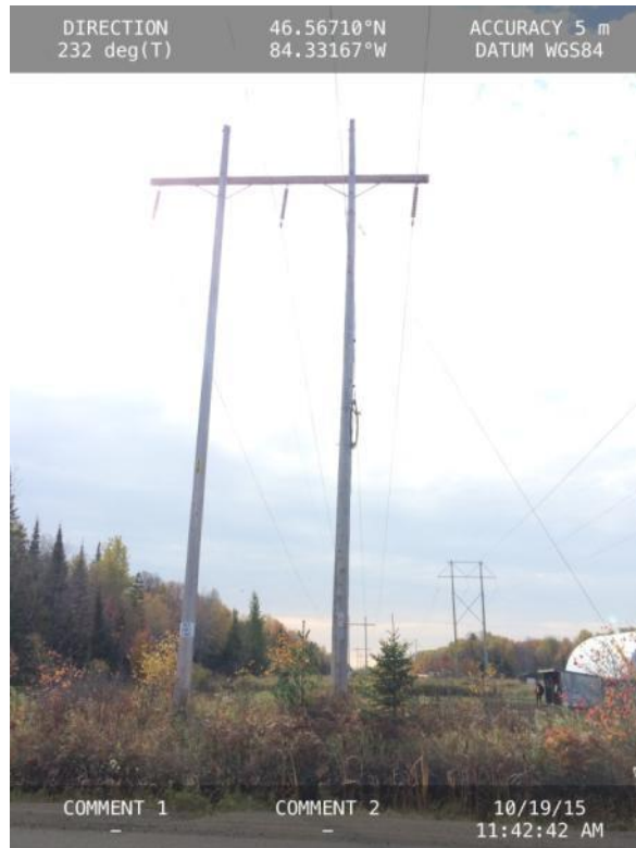
Figure 3-2: No.3 Sault Structure with Composite Insulators
