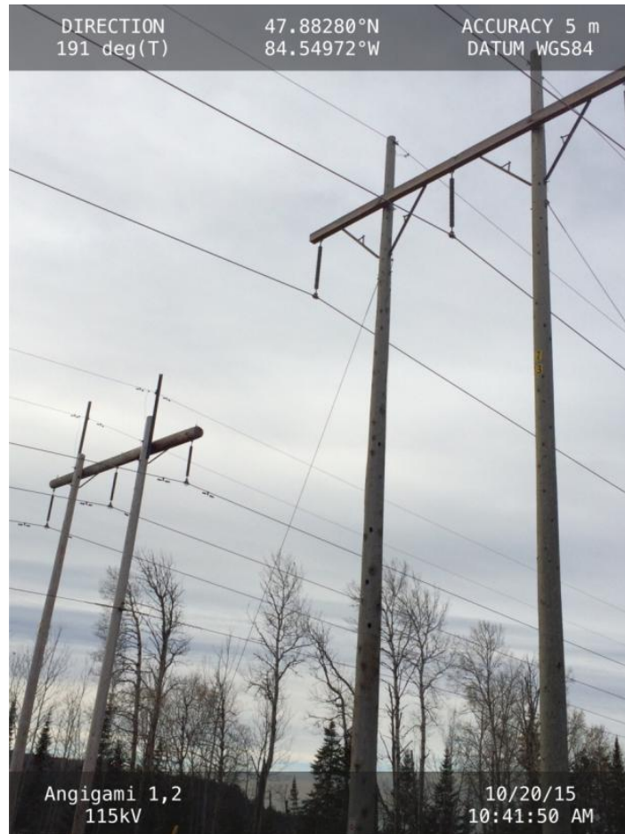
Figure 11-1: High Falls (No.1 & 2) Transmission Line
