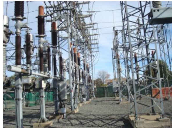
Figure 12-2: Steelton TS View 2
