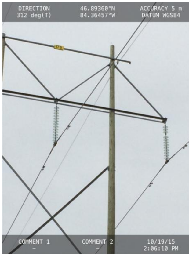
Figure 1-2: Broken Insulator Disc (Right Phase_Str-178)
