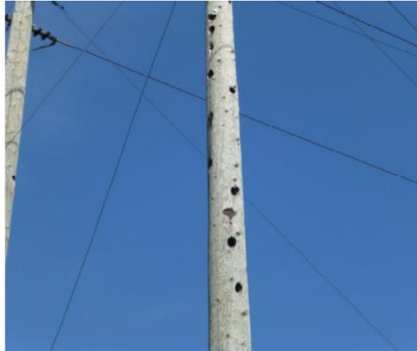
Figure 9-1: Example of a Wooden Pole with Woodpecker Damage
