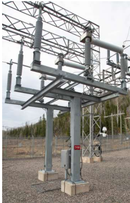
Figure 6.42: Circuit Switcher 598 at Batchawana Transmission Station
