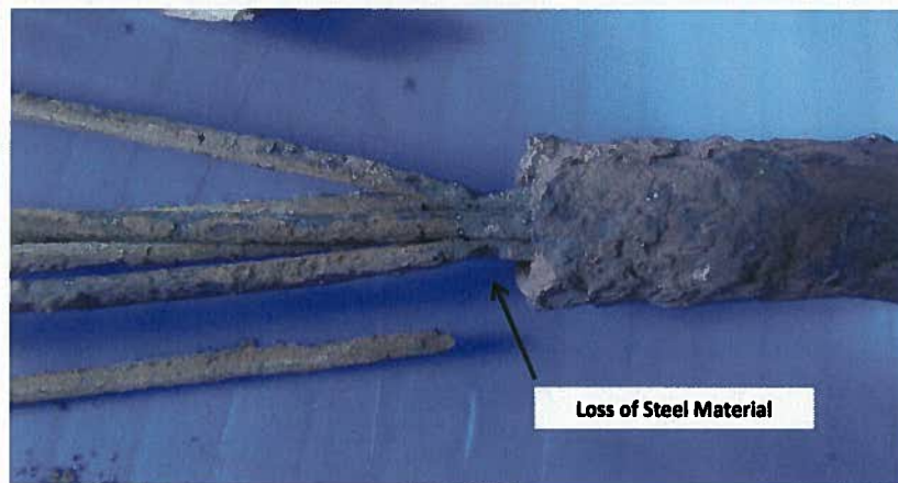
Figure 5 - Failed Side - Heavily Rusted Steel Wires at Mouth of Splice
