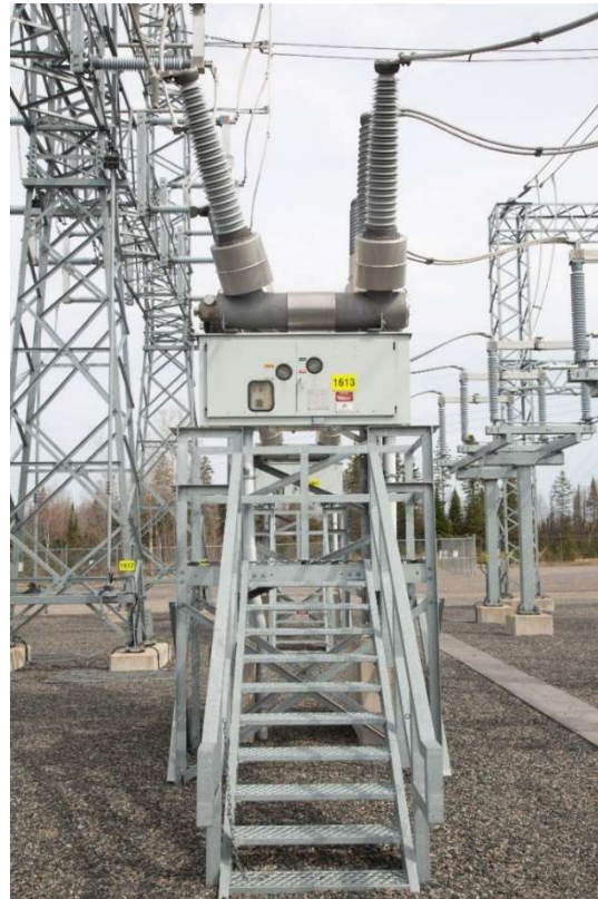
Figure 6.15: SF6 Circuit Breaker 1613 at Third Line Transmission Station
