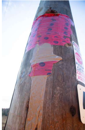
Figure 6.59: Heavy Woodpecker damage - holes filled with epoxy resin.
