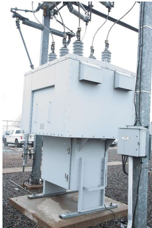
Figure 6.10 Vacuum Circuit Breaker 385 at Northern Avenue Transmission Station
