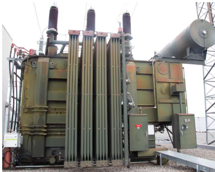
Figure 6.60: 230/115 kV Autotransformer T2 at Third Line Transmission Station
