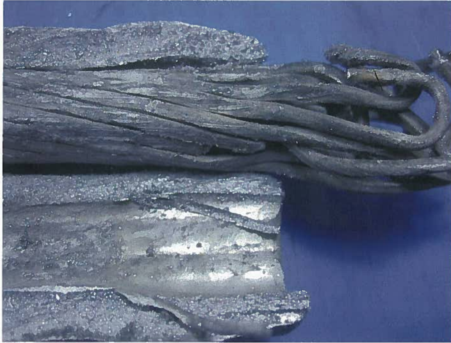
Figure 8: Failed Connector: failed conductor end, no signs of corrosion
