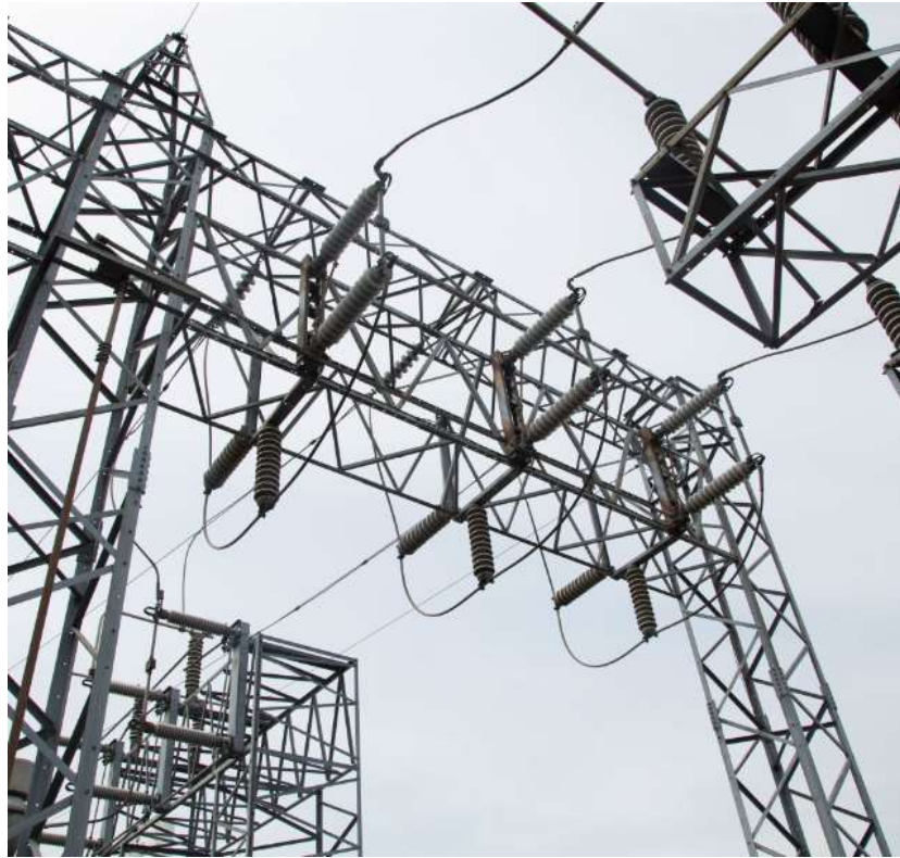
Figure 6.33: Overhead Disconnect Switch 203 at Steelton Transmission Station
