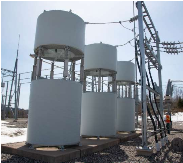
Figure 6.50: Air-core Shunt Reactor R1 at Mackay Transmission Station
