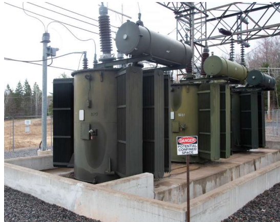
Figure 6.61: Banked Transformers at Goulais Transmission Station
