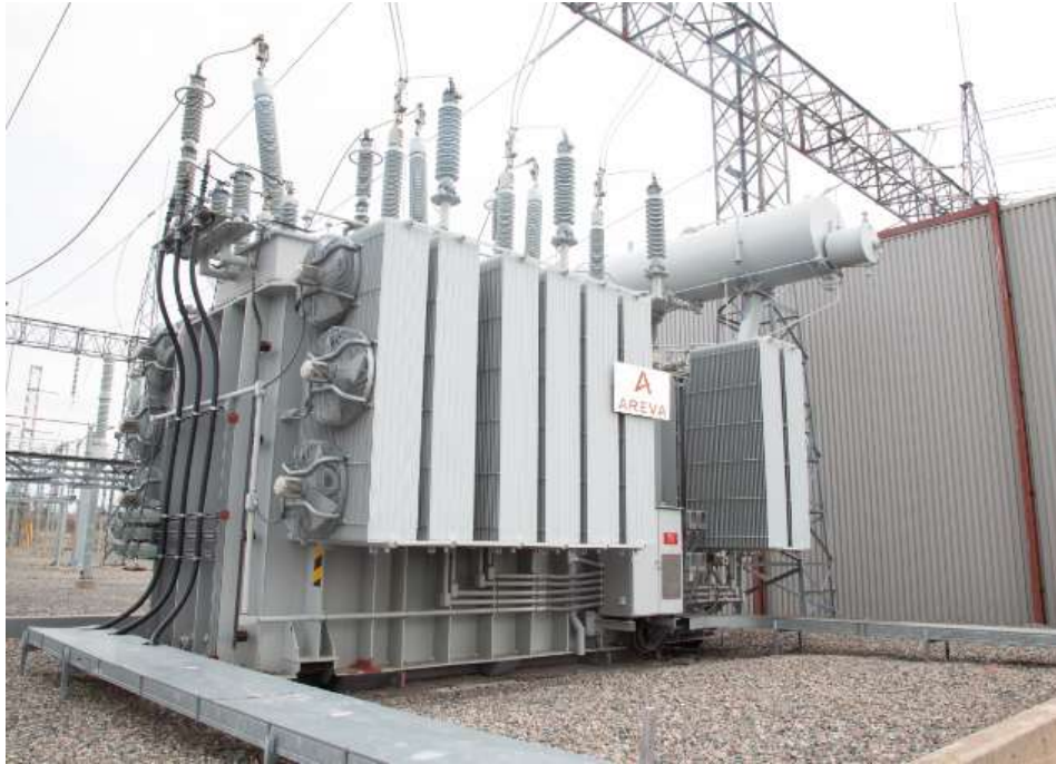
Figure 6.5: 230/115 kV Autotransformer T1 at Third Line Transmission Station
