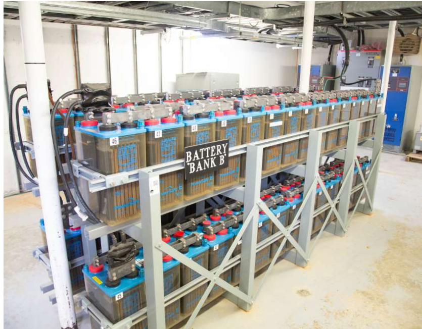
Figure 6.29 Vented-type Battery Bank 'B' at Third Line Transmission Station
