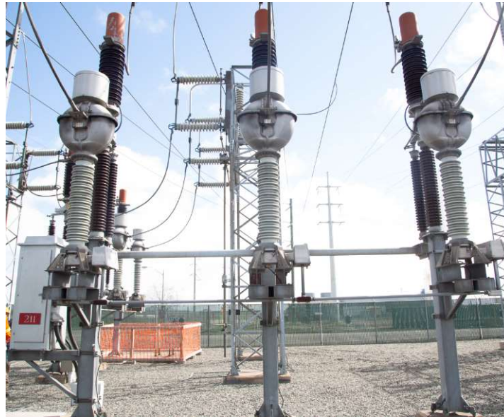
Figure 6.20: Oil Circuit Breaker 211 at Steelton Transmission Station
