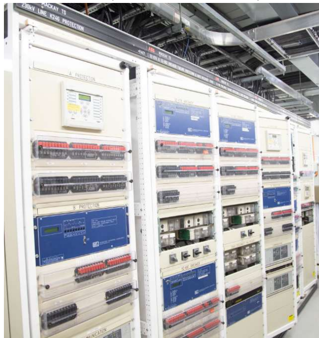
Figure 6.38: Electronic Relay Cabinets at Mackay Transmission Station
