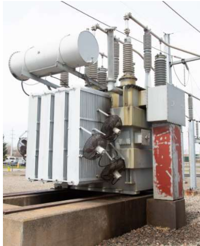
Figure 6.62: Transformer MT2 at Clergue Transmission Station
