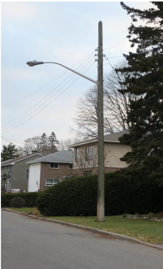
Figure 1 a): A Joint-Use Utility Pole (Without Carrier Attachments)
