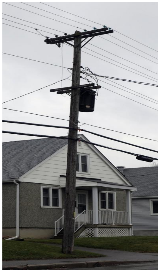
Figure 1 b): A Joint-Use Utility Pole (With Carrier Attachments)
