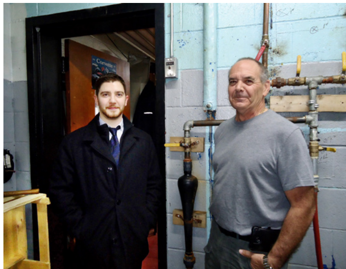
Enbridge Energy Solutions Consultant, Daniel Duhamel, being shown the compact REALice installation by Facilities Manager, Larry Woodley
