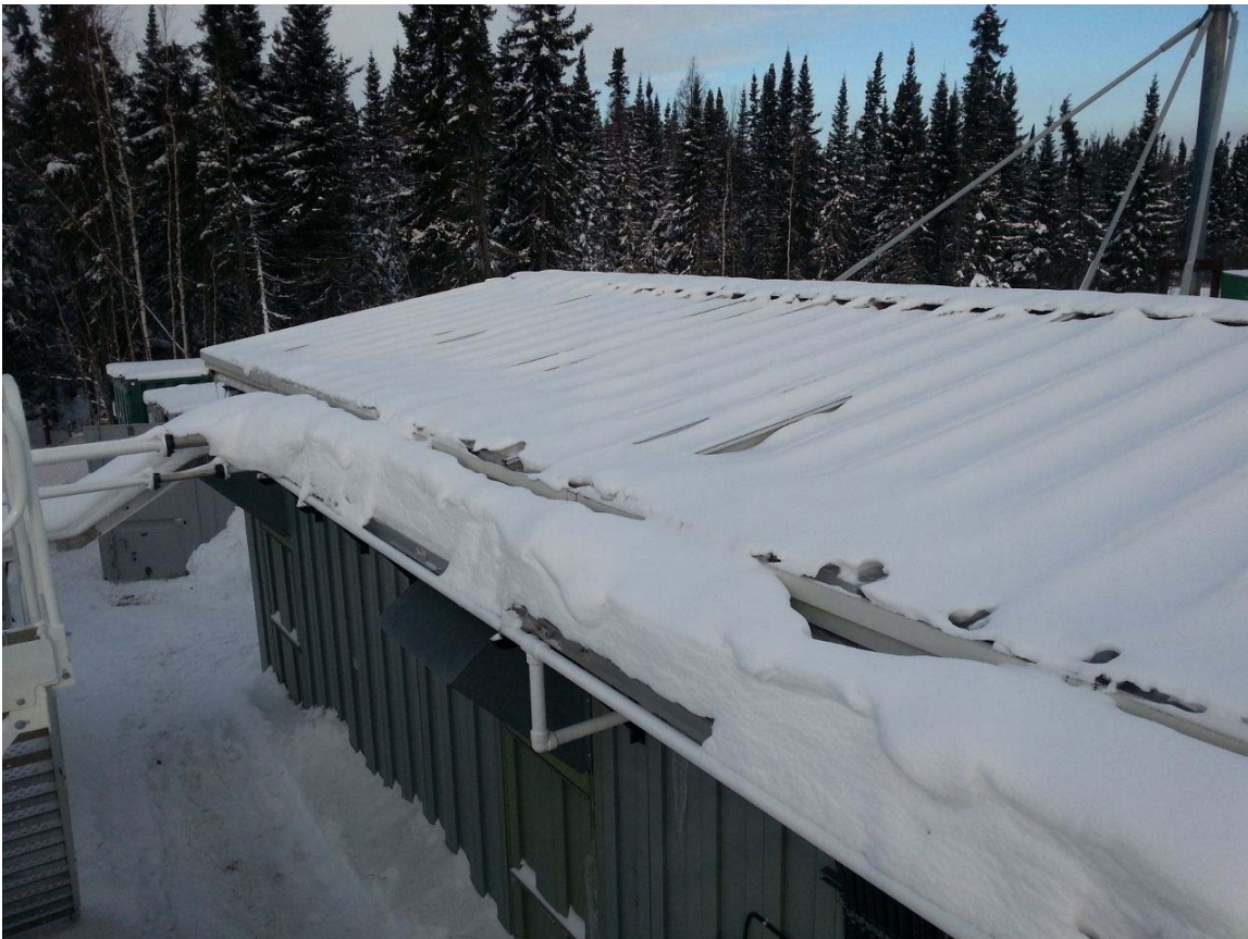
Photo#17 – Exposed Fuel Line Tray & Visible Heat Loss (Weagamow)
