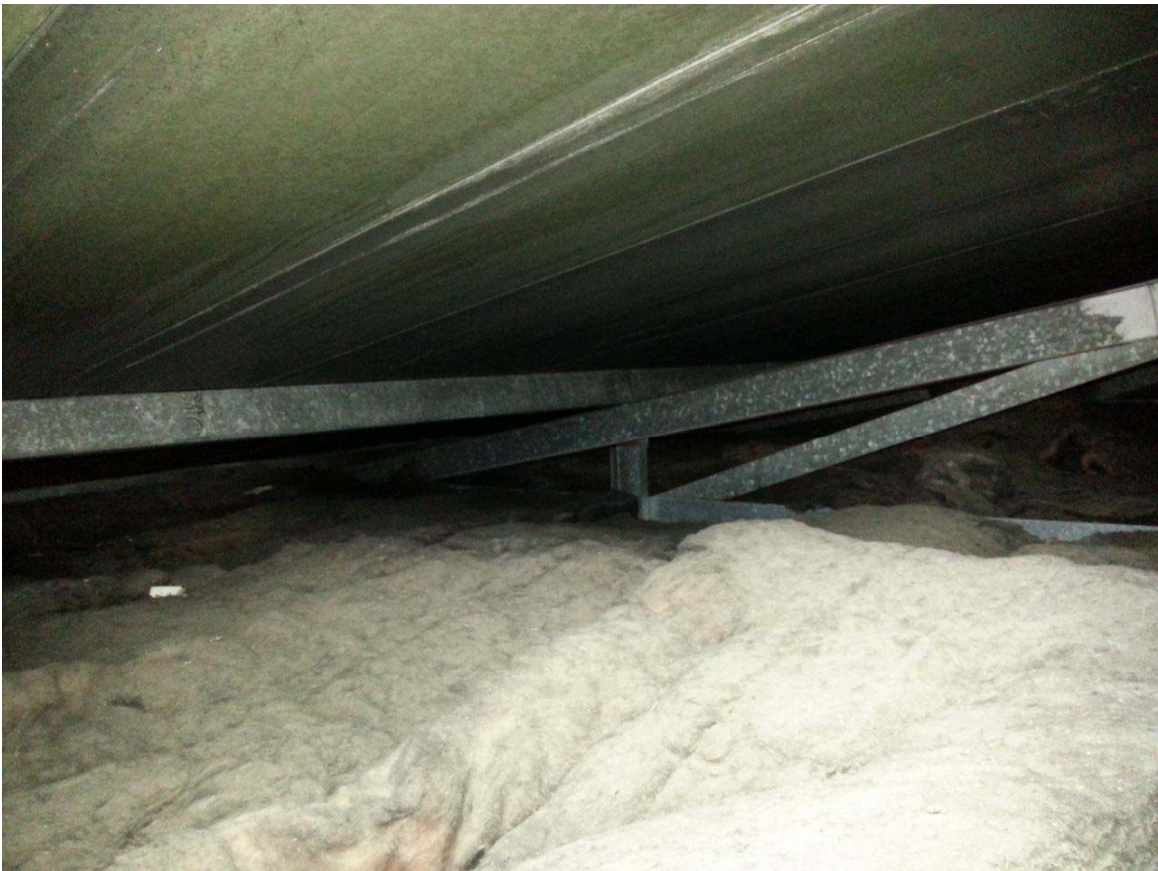
Photo#16 – Insufficient Air Space (Weagamow)
