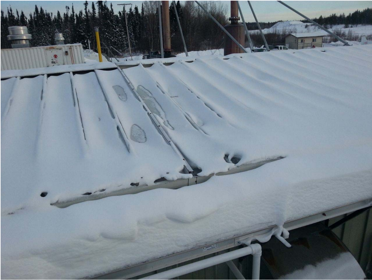
Photo#18 – Visible Heat Loss & Roof Panel Deterioration Signs (Weagamow)
