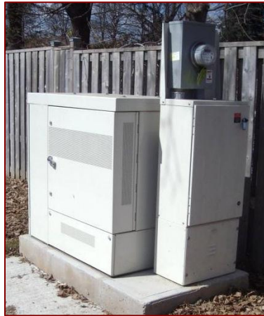
Figure 5-1, Bell Communications Enclosure
