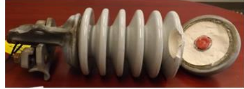
Failed Porcelain Insulator
