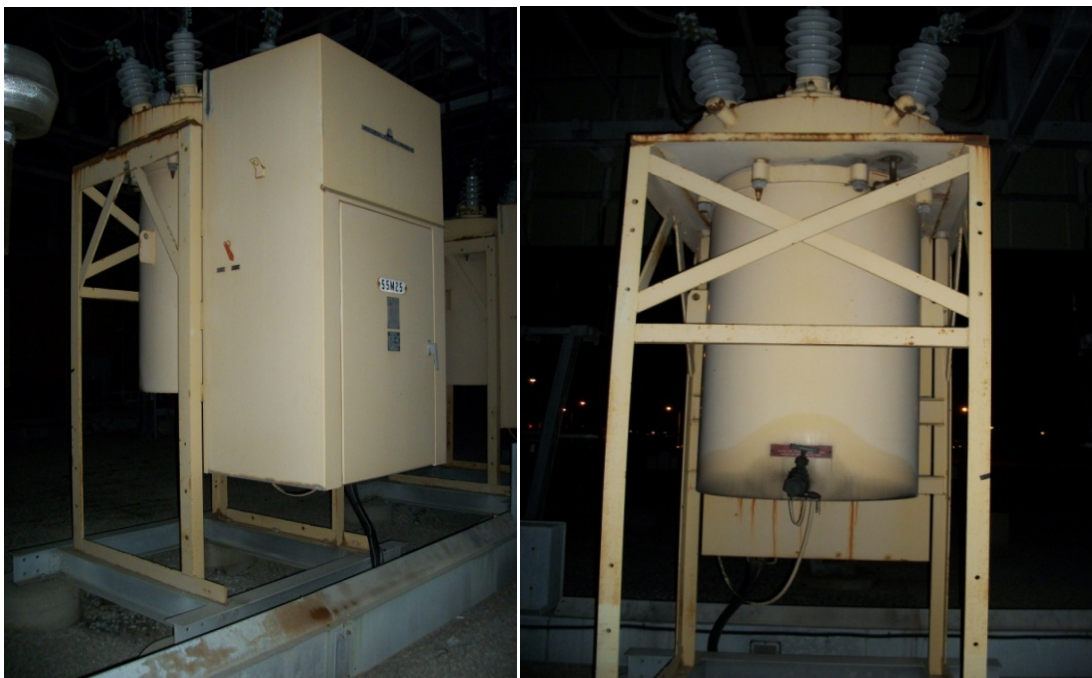
9 Figure 8: Circuit Breaker at Finch TS 55M25 (February 2, 2012)
