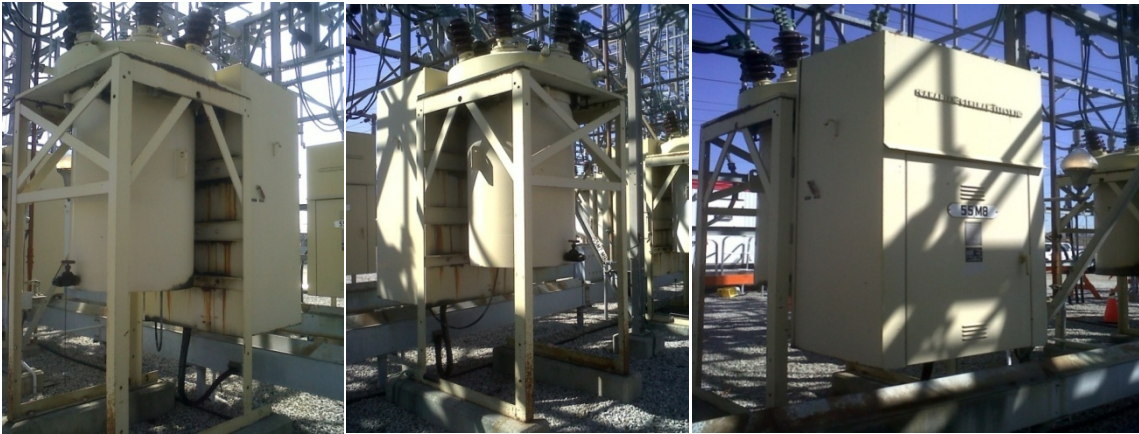
9 Figure 9: Circuit Breaker at Finch TS 55M8 (March 14, 2012)
