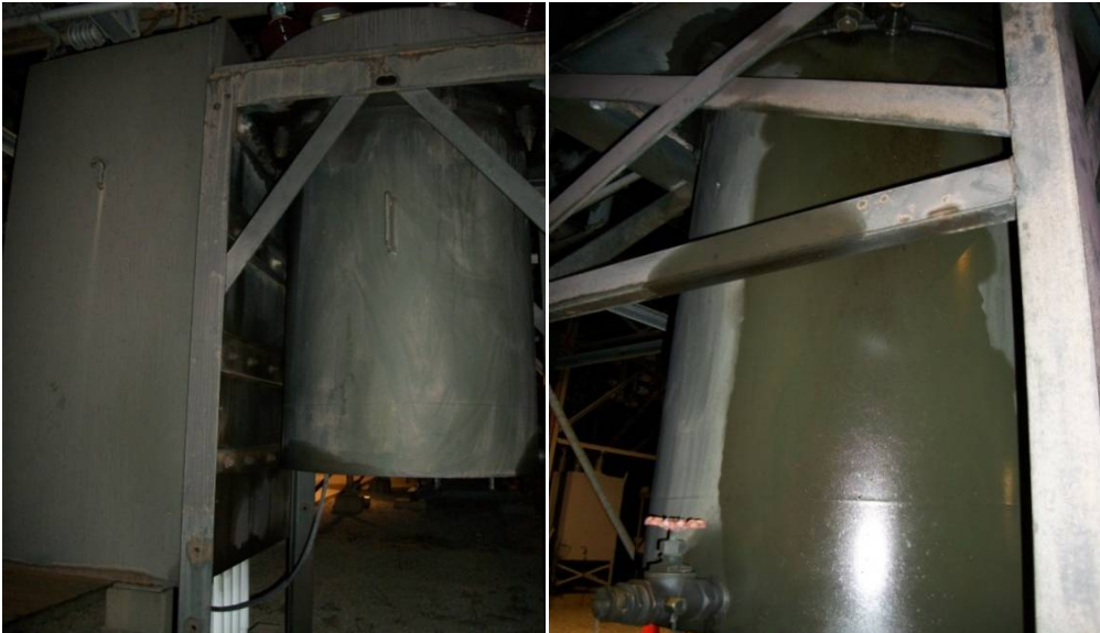
9 Figure 11: Circuit Breaker at Bathurst TS 85M4 (February 2, 2012)
