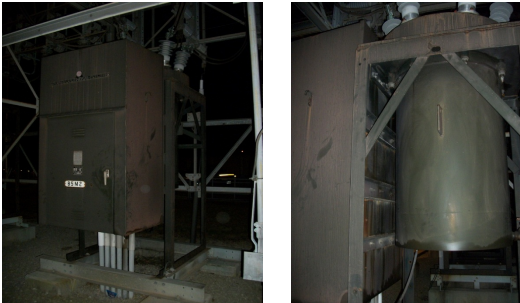
9 Figure 12: Circuit Breaker at Bathurst TS 85M2 (February 2, 2012)
