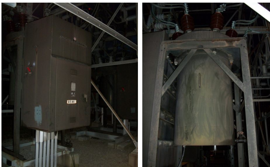
9 Figure 10: Circuit Breaker at Bathurst TS 85M1 (February 2, 2012)
