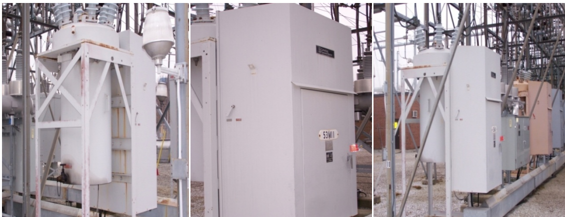
9 Figure 6: Circuit Breaker at Bermondsey TS 53M11 (February 3, 2012)
