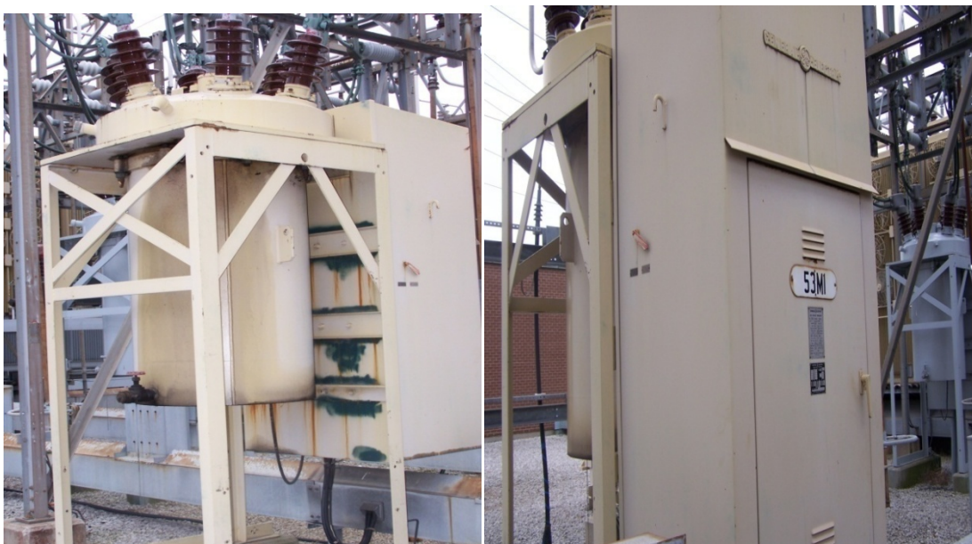
9 Figure 4: Circuit Breaker at Bermondsey TS 53M1 (February 3, 2012)
