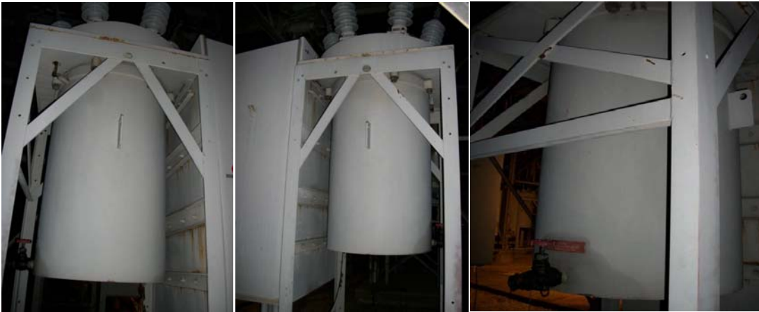
9 Figure 13: Circuit Breaker at Bathurst TS 85M25 (February 2, 2012)
