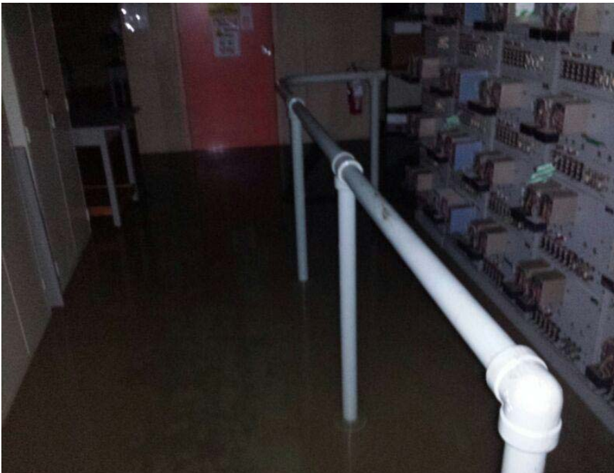
3 Figure 10: Flooded substation equipment at HONI's Manby TS - July 8-10, 2013
