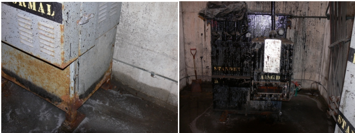
Figure 2: Photo of ATS and Transformer in Location D3008
