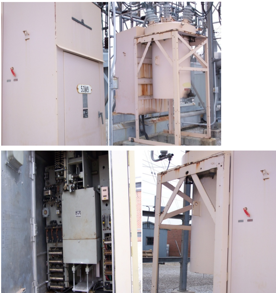
9 Figure 5: Circuit Breaker at Bermondsey TS 53M9 (February 3, 2012)
