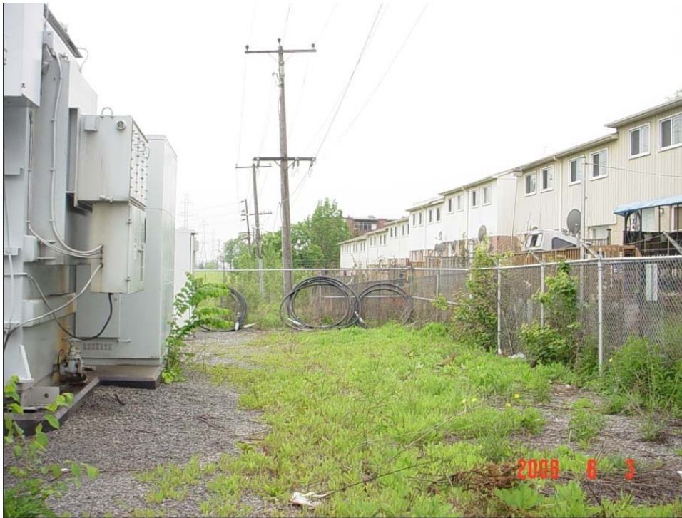
4 Figure 4: Jane MS Transformers
