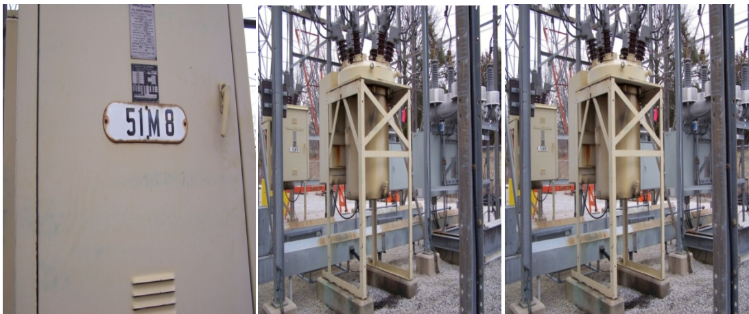
9 Figure 3: Circuit Breaker at Leslie TS 51M8 (February 3, 2012)
