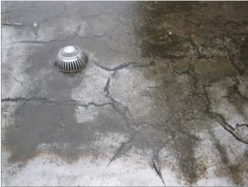
1 Figure 6: Cracked roof of Merton MS
