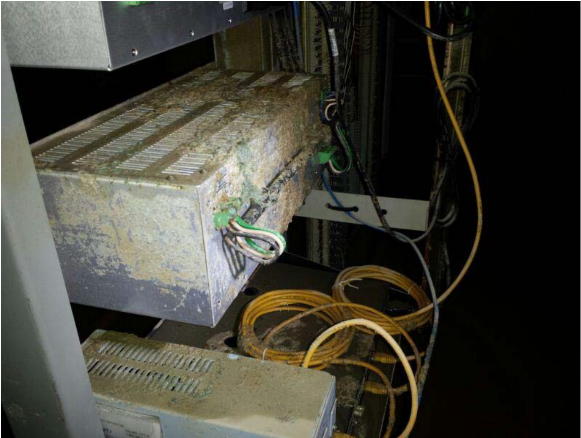
1 Figure 11: Flood damaged substation equipment at HONI's Manby TS - July 8-10, 2013
