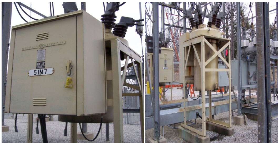
9 Figure 2: Circuit Breaker at Leslie TS 51M7 (February 3, 2012)
