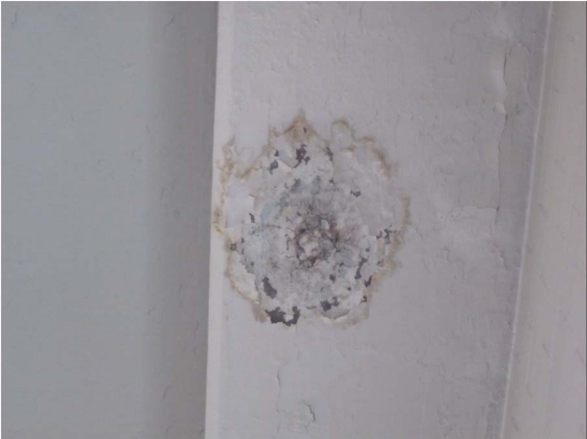
1 Figure 9: Leaking roof of Danforth MS
