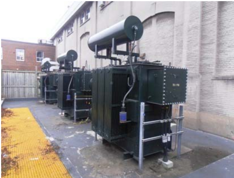
8 Figure 3: 1 Strachan B Power Transformers
