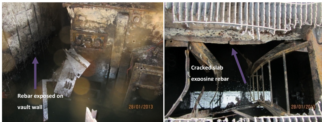
1 Figure 4: Images of the damaged civil structure caused by the fire.
