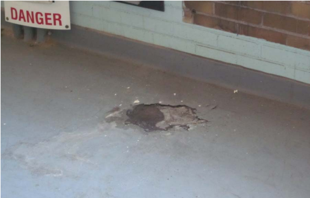
1 Figure 8: Roof leak at Danforth MS Floor
