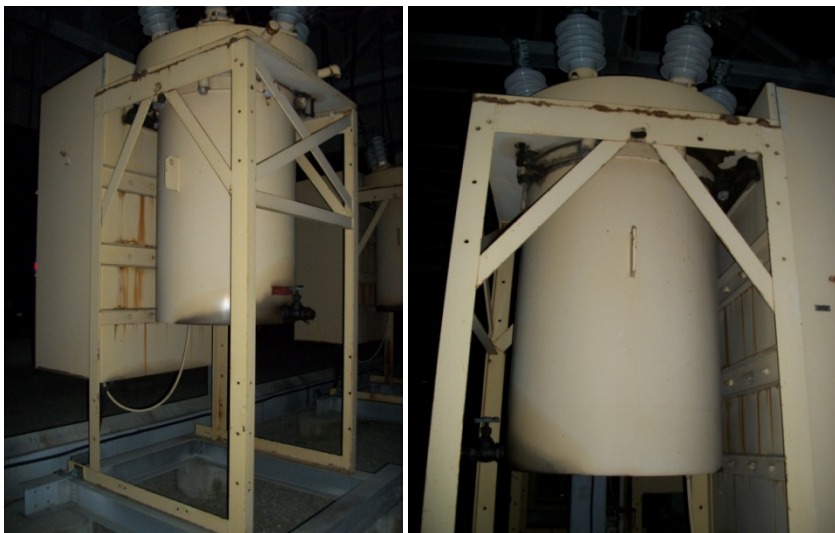
9 Figure 7: Circuit Breaker at Finch TS 55M24 (February 2, 2012)
