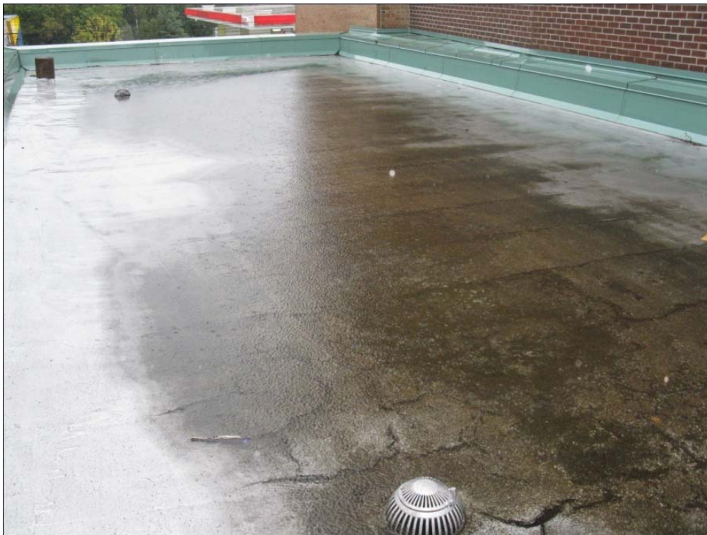
3 Figure 7: Cracked roof of Merton MS
