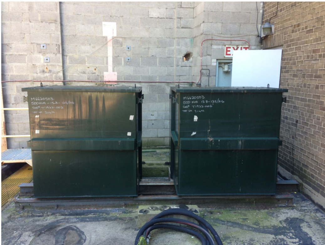
9 Figure 5: Glengrove TS station service transformers
