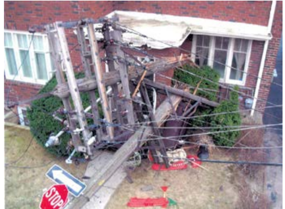
B4 - Fig 13 Broken pole on home - Acacia Rd.
