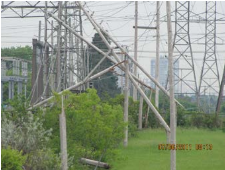
B4 - Fig 8 Multiple pole failure
