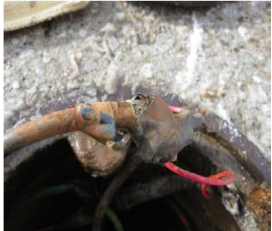
B3 - Fig 3 Degraded conditions of split bolt connectors in handwells
