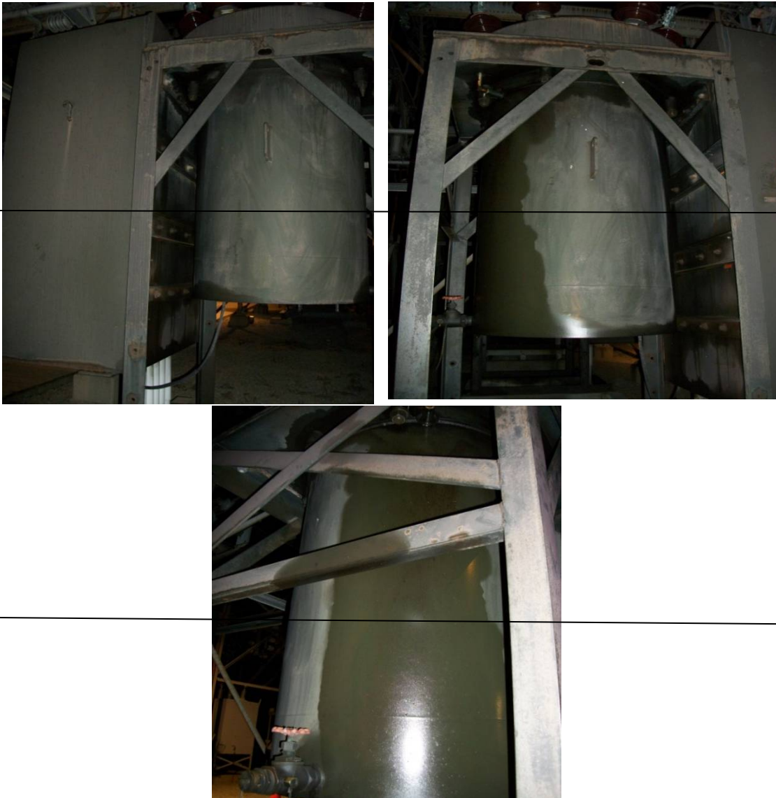
Figure 21: Circuit Breaker at Bathurst TS 85M4 (February 2, 2012)
