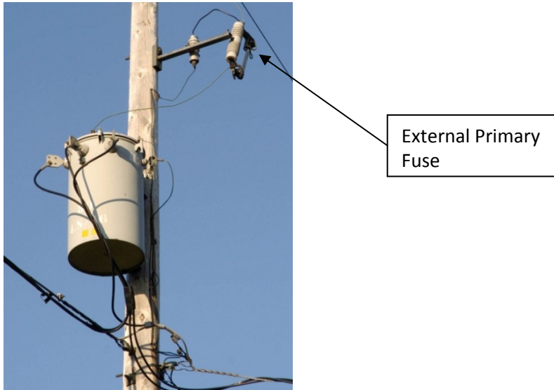
1 Figure C: Standard Non-CSP Transformer
