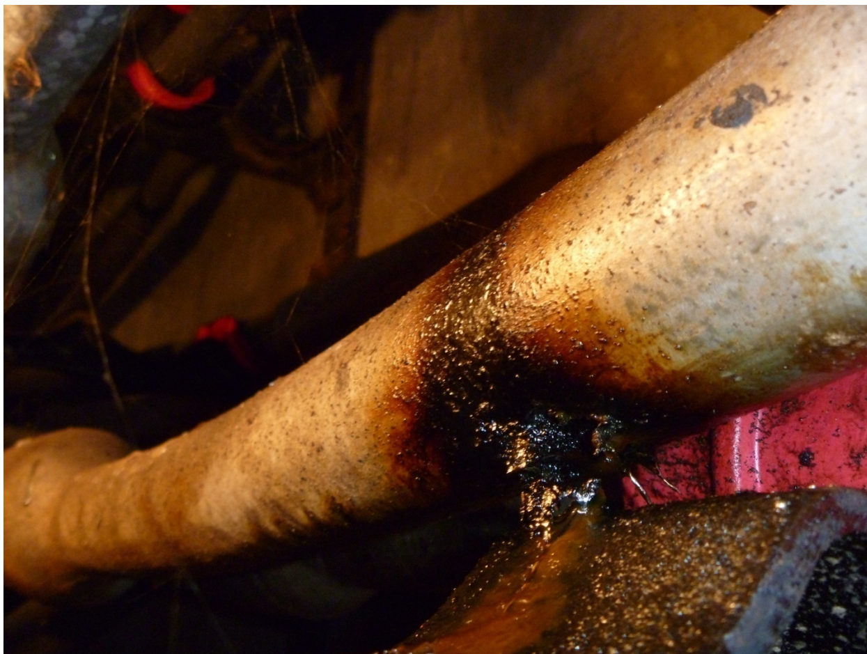
1 Figure 5: Leaking Oil from PILC Cables Connecting Bridgman to High Level Stations 2 (January 18, 2012)
