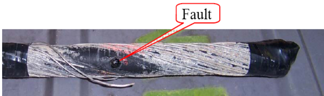
Figure 40: Fault due to premature insulation failure (taken on January 14, 2009)
