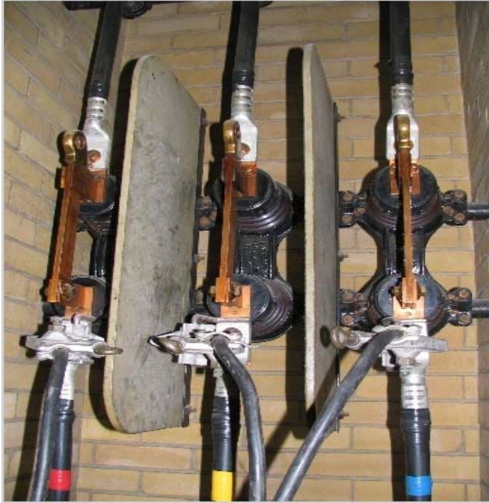
1 Figure 8: Carlaw TS 13.8kV live parts of a switchgear in an open brick structure
