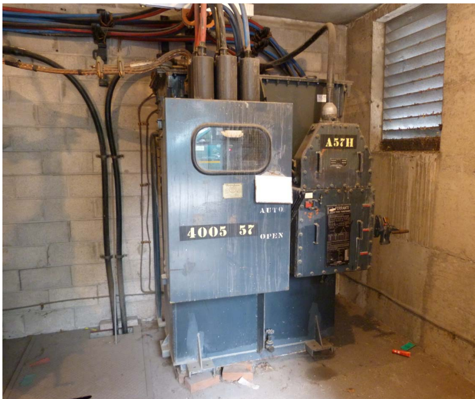
1 Figure 10 – Walk-in Building Network Vault. (November 2011)
