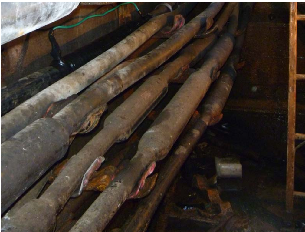
3 Figure 9: After — Cable Chamber showing properly supported cables and splices in a cable 4 rack within the cable chamber (January 18, 2012)
