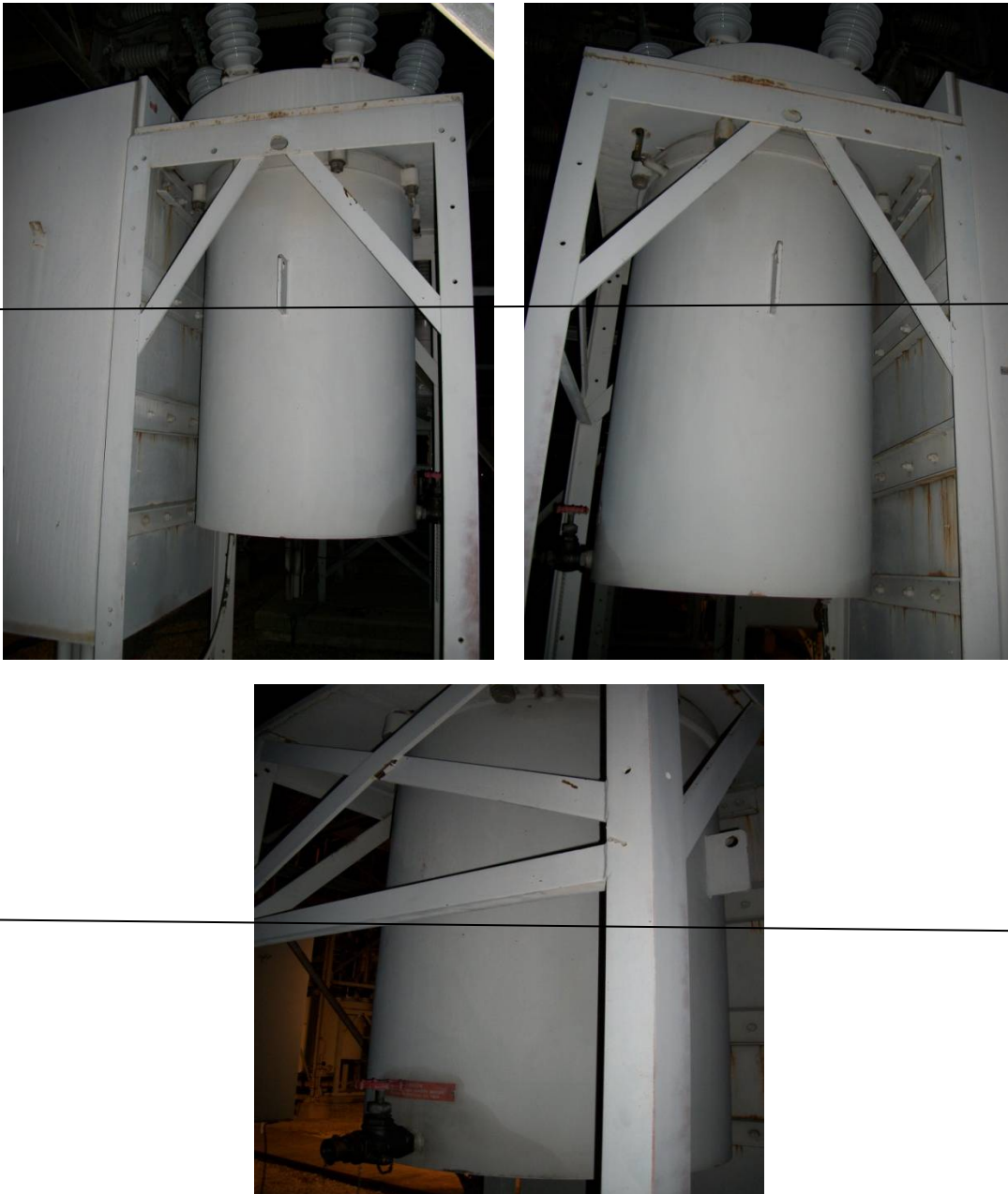
Figure 23: Circuit Breaker at Bathurst TS 85M25 (February 2, 2012)
