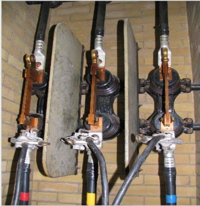
1 Figure 8: Carlaw TS 13.8kV live parts of a switchgear in an open brick structure
