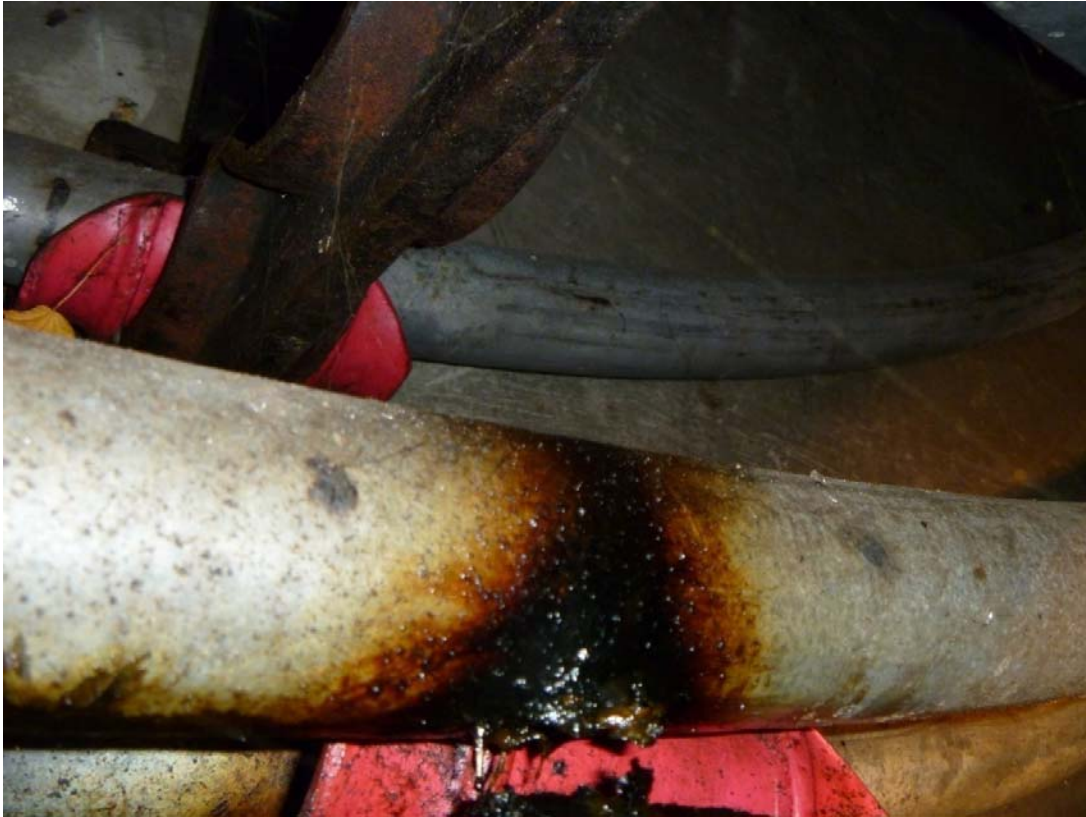
1 Figure 1: Leaking PILC Cable (January 18, 2012)
