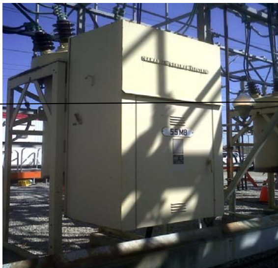
Figure 19: Circuit Breaker at Finch TS 55M8 (March 14, 2012)
