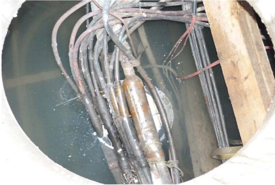
1 Figure 8: Before — Cable Chamber Requiring Piece Outs at Yonge and Merton 2 (January 16, 2012)
