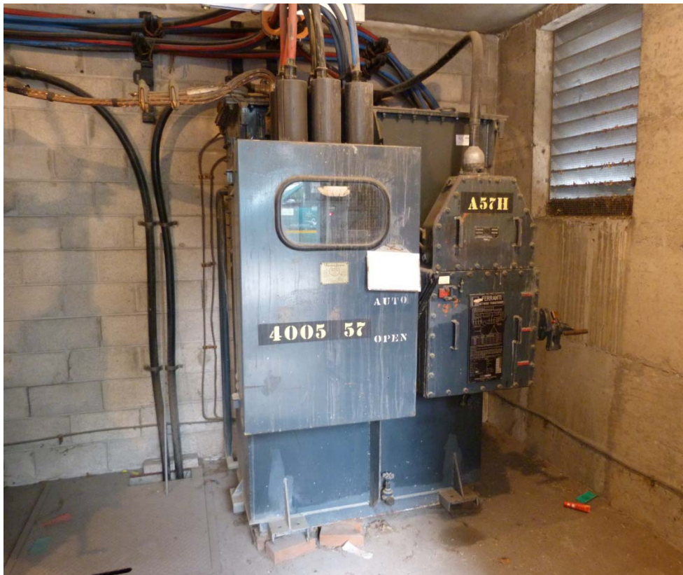
1 Figure 10 – Walk-in Building Network Vault. (November 2011)
