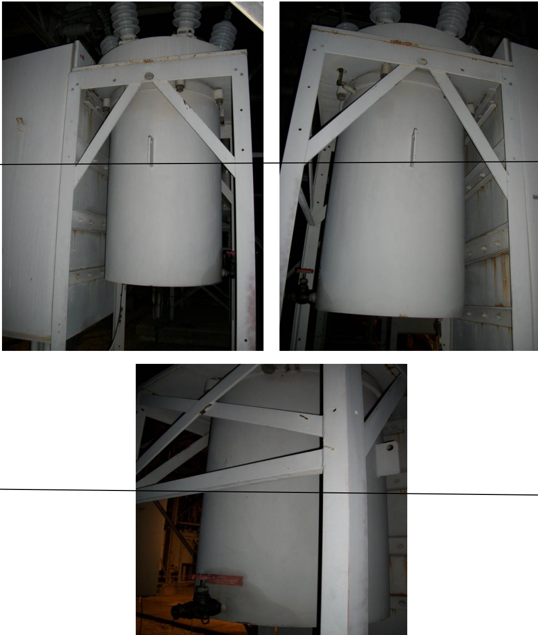
Figure 23: Circuit Breaker at Bathurst TS 85M25 (February 2, 2012)
