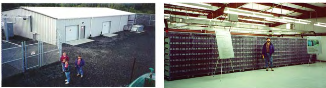
Figure 4-7 1-MW/1.5-MWh Lead-Acid System at Metlakalta, Alaska
