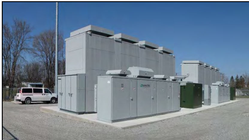
Figure 4-11 AEP Distribution Substation with Sodium-Sulfur Unit
