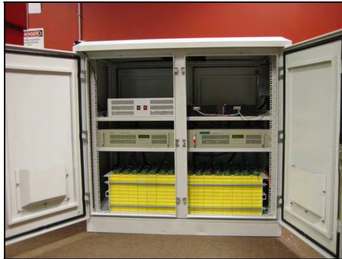
Figure 4-20 6-kW/20-kWh Li-ion system with inverter and controls by GreenSmith Energy Management. EPRI will be testing a 25-kW/50-kWh GreenSmith system in late 2010.
