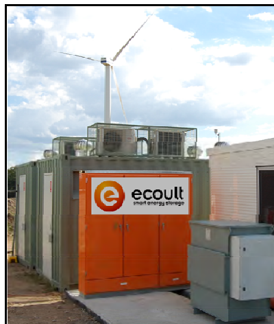
Figure 4-8 Phase 1 of Ecoult 1-MW/1-MWh UltraBattery system at Hampton Wind Smoothing Project in Australia (Source: Ecoult).
