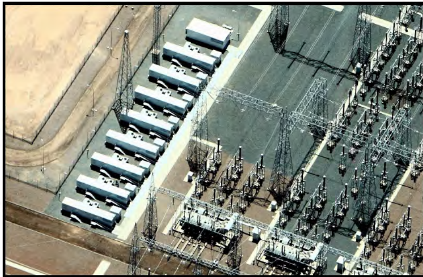
Figure ES-7 Commercial operation of a 12-MW frequency regulation and spinning reserve project at AES Gener's Los Andes substation in the Atacama Desert, Chile. The system uses A123 Systems' Li-ion Hybrid Ancillary Power Units (Hybrid-APUs™).
