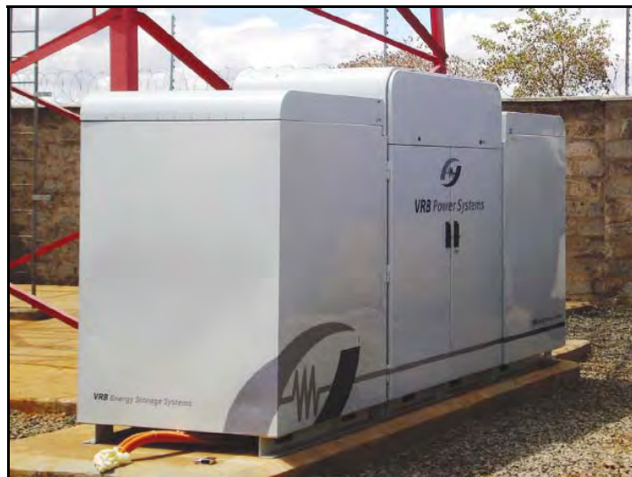
Figure 4-12 Prudent Energy 5-kW/30-kWh VRB-ESS installed at Kitangi, Kenya works alongside a diesel generator to comprise a hybrid power system at an off-grid site.
