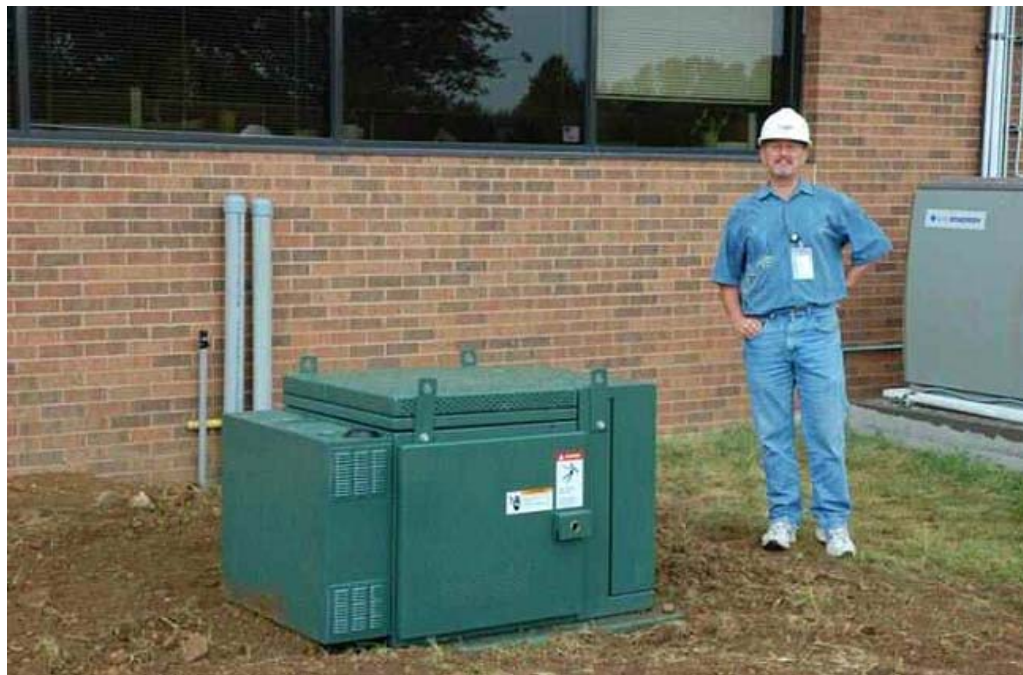
Figure H-5. Completed 25 kW CES Installation at AEP
