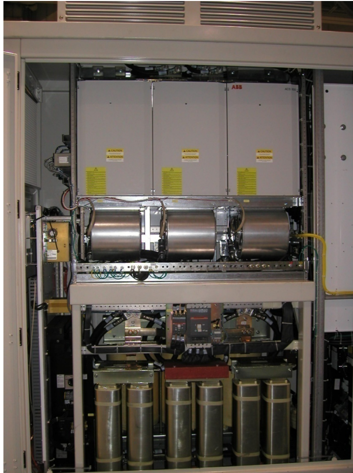
Figure 30. Inside View of 500 kVA PCS Provided by ABB for AEP Pilot
