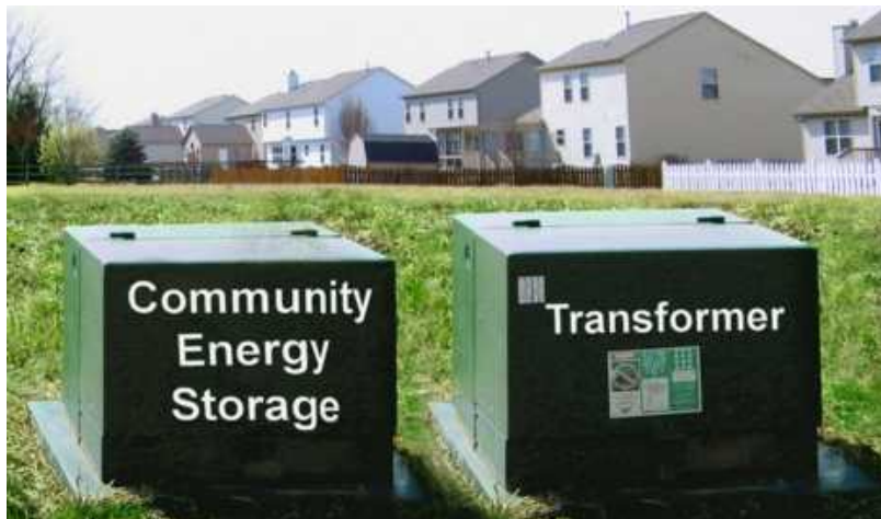
Figure 26. Padmount Community Energy Storage next to Padmount Transformer (Ref. -11)
