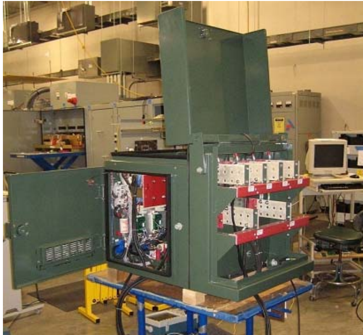
Figure 28. S&C 2.0 MW / 2.5 MVA Smart Grid SMS™ Storage Management System (Ref.-15)
