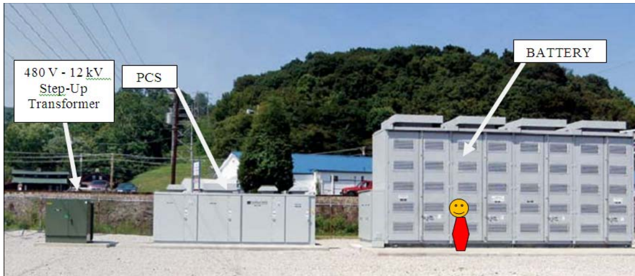
Figure 31. AEP Distributed Energy Storage (1.2 MW 7.2 MWh NaS Battery) S&C / NGK
