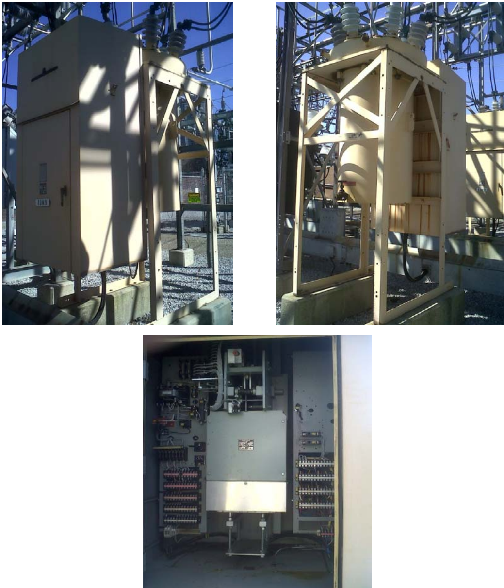
Figure 11: Circuit Breaker at Fairchild TS 80M9 (March 14, 2012)
