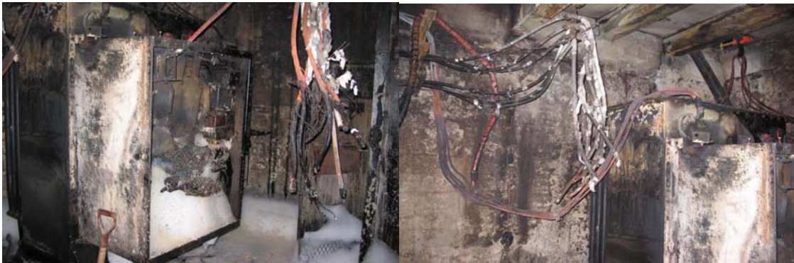
1 Figure 6 - LEFT: Failed Protector. RIGHT: Burnt AIRC cables. (March 24, 2007)
