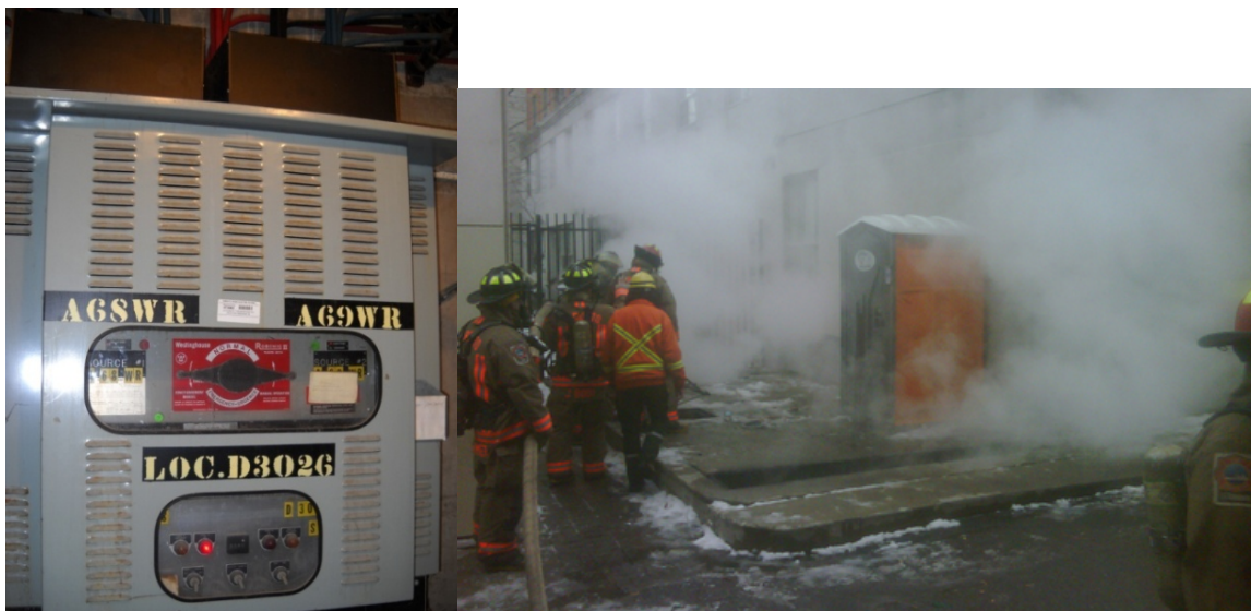
4 Figure 3: LEFT: Photo of a typical ATS unit. RIGHT: The fire department putting out the fire at 5 33 Princess Street. PHOTO TAKEN January 16, 2012
