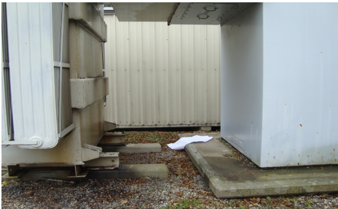
1 Figure 2: Station Transformer, TR1, leakage at Scarborough Golf Club MS (November 16, 2011)
