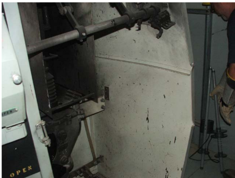
2 Figure 2: [2007] Impact of internal arc fault in a switchgear
