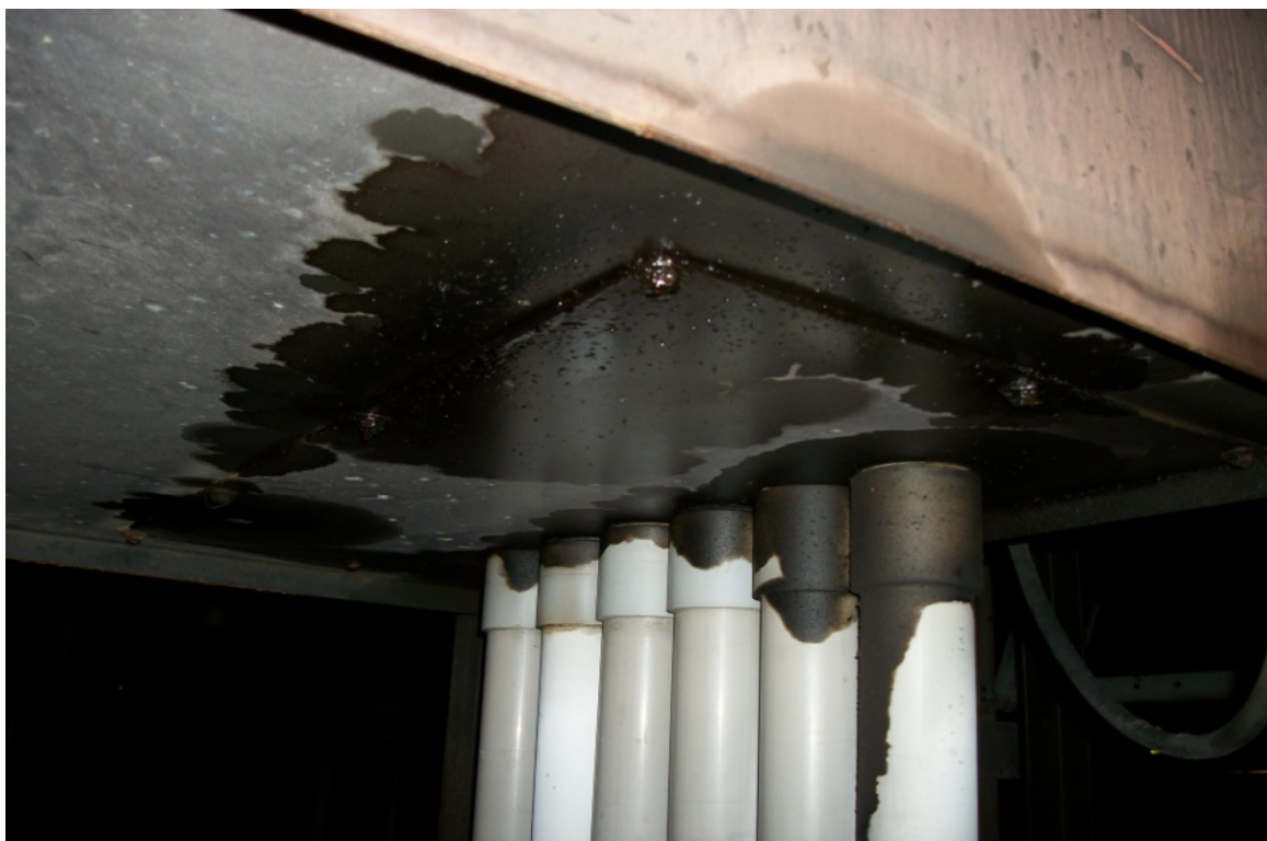
Figure 20: Circuit Breaker at Bathurst TS 85M1 (February 2, 2012)
