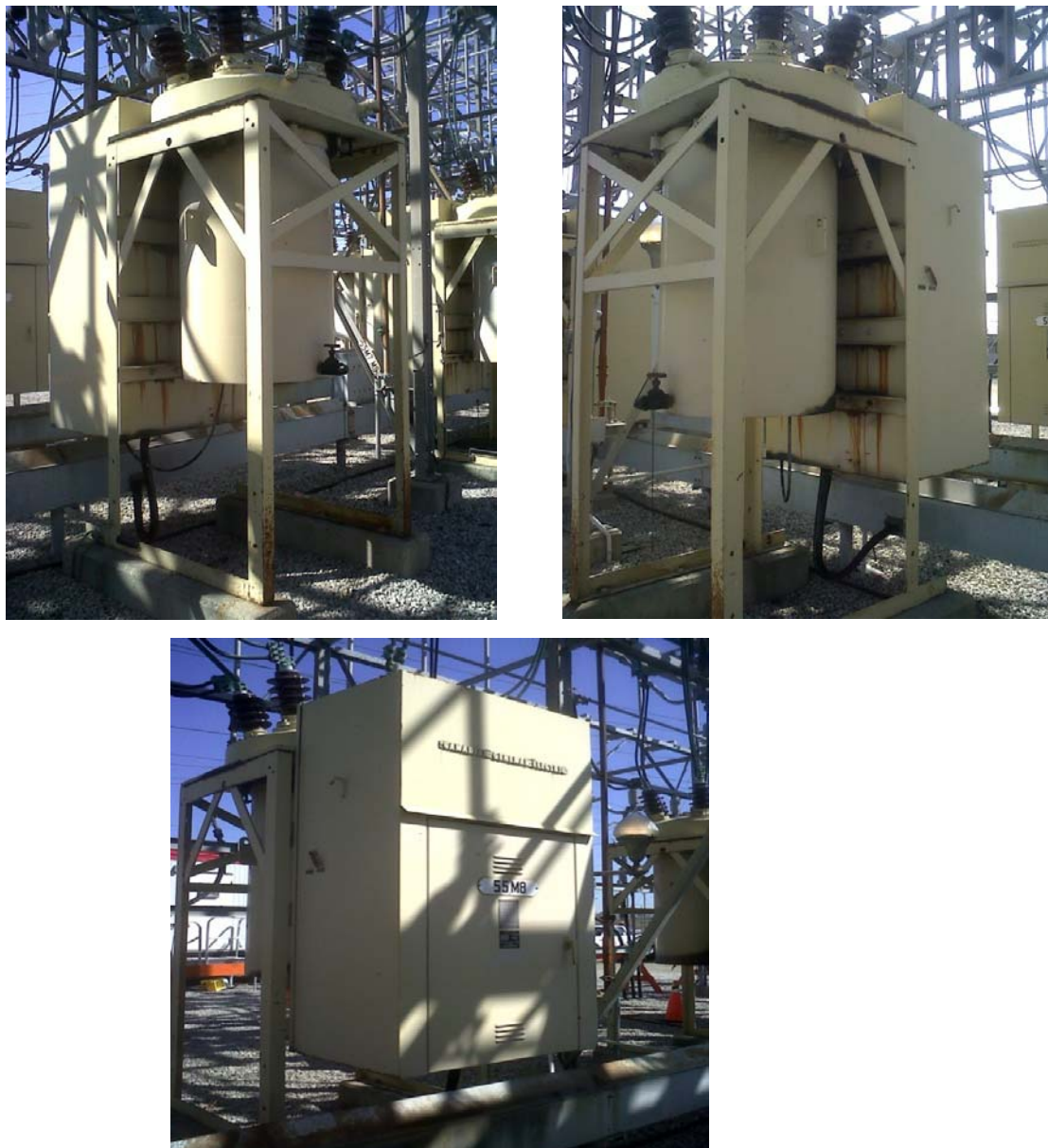
Figure 19: Circuit Breaker at Finch TS 55M8 (March 14, 2012)
