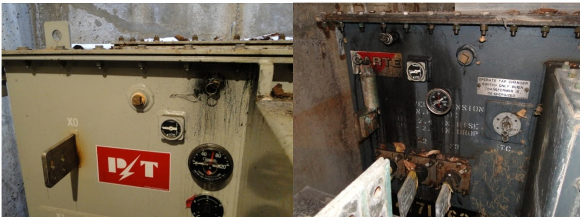
3 Figure 7: Damaged transformers at 50 Marlborough. PHOTOS from January 10, 2010
