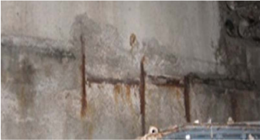
1 Figure 6: Network Vault Wall with Exposed Rebar
