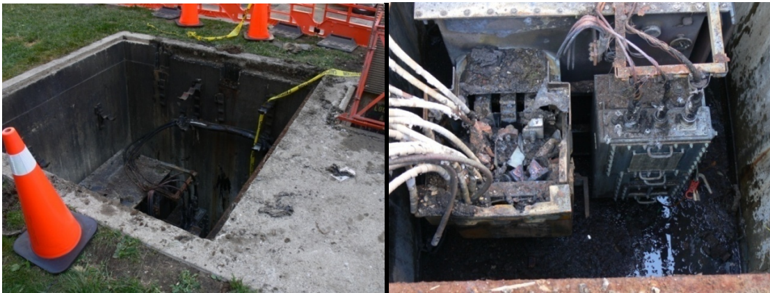
1 Figure 7 - LEFT: Vault 4557 with roof slabs off, signs of heavy smoke apparent in vault. RIGHT: 2 damaged Fibertop Network Unit. (June 1, 2010)
