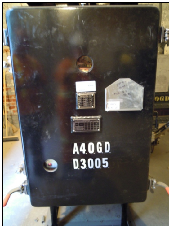
1 Figure 14: Stand alone network protector (submersible equipment)
