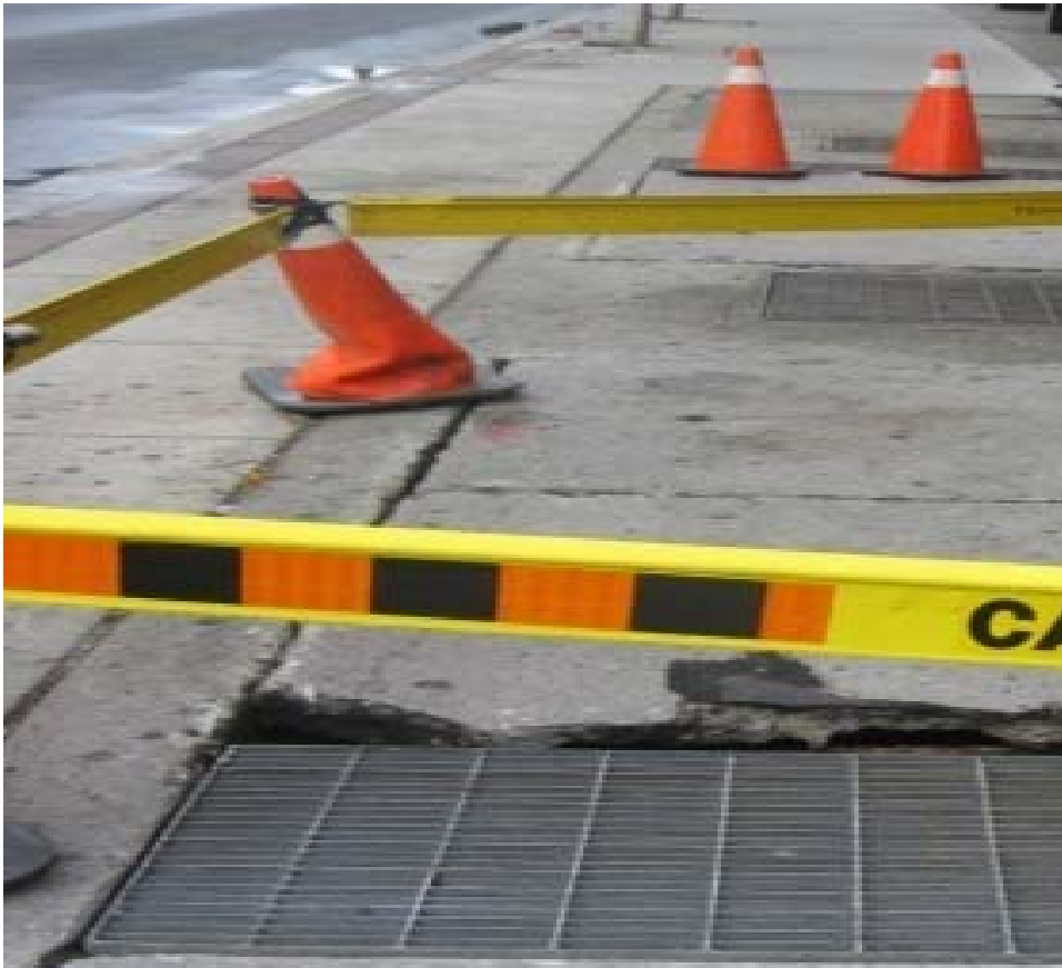
1 Figure 13: Photo of a vault roof collapsed due to failed supporting beam
