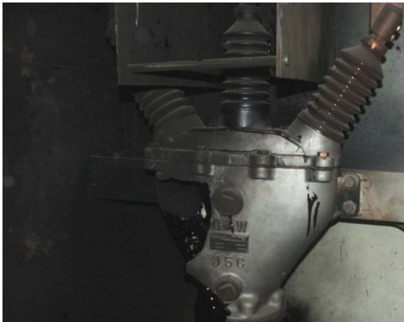
1 Figure 1: [2007] Pothead failed inside Terauley TS switchgear
