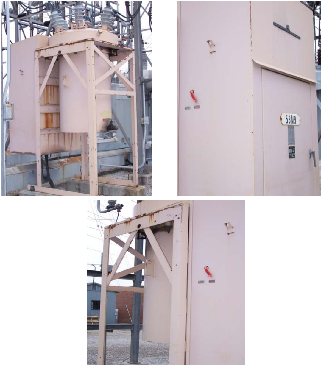
Figure 15: Circuit Breaker at Bermondsey TS 53M9 (February 3, 2012)
