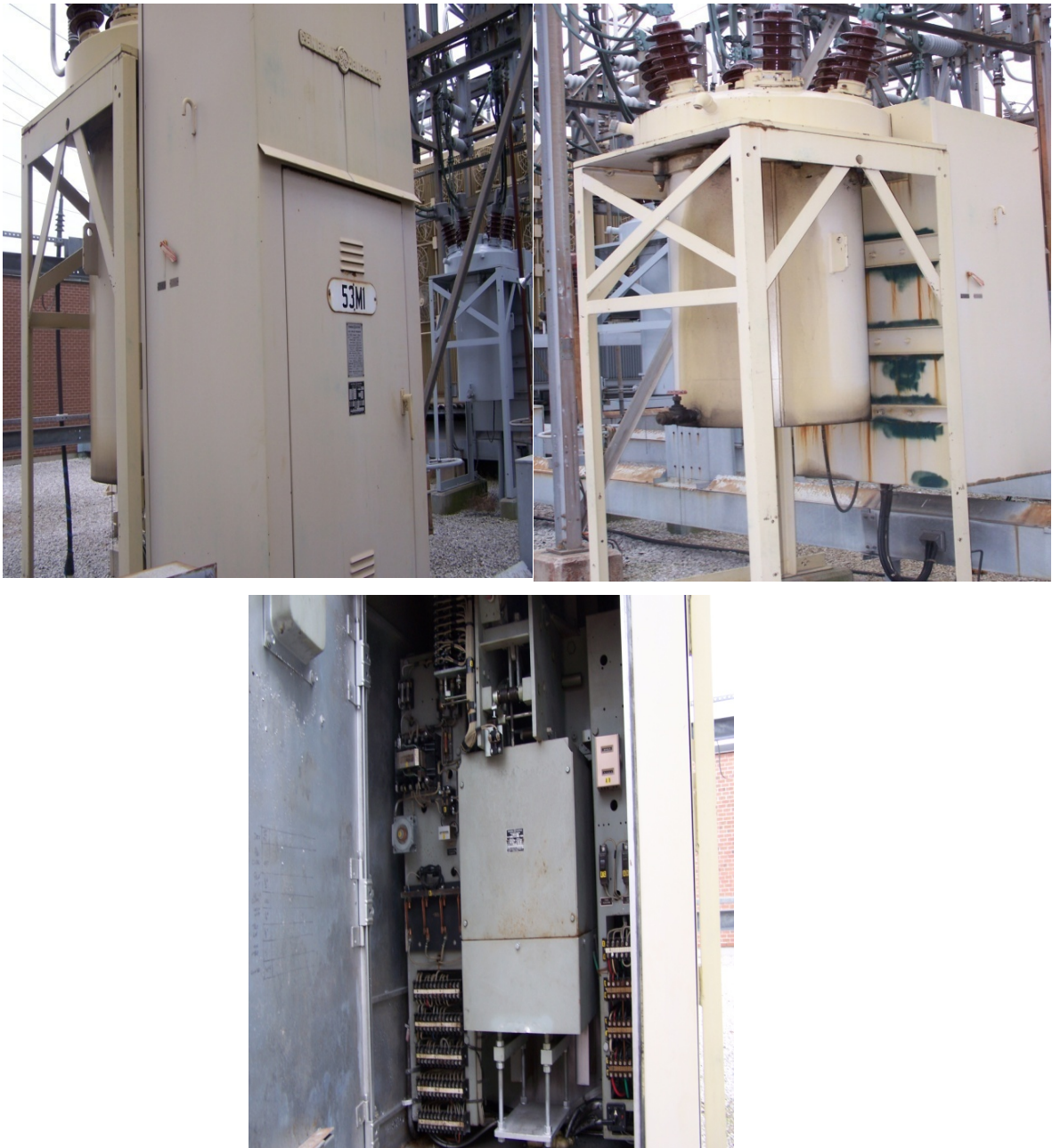
Figure 14: Circuit Breaker at Bermondsey TS 53M1 (February 3, 2012)
