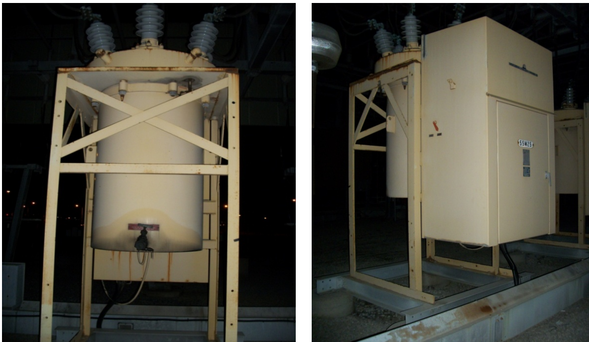
Figure 18: Circuit Breaker at Finch TS 55M25 (February 2, 2012)
