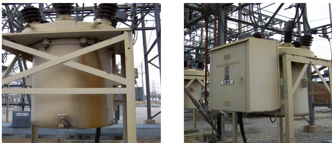
Figure 7: Circuit Breaker at Leslie TS 51M6 (March 12, 2012)
