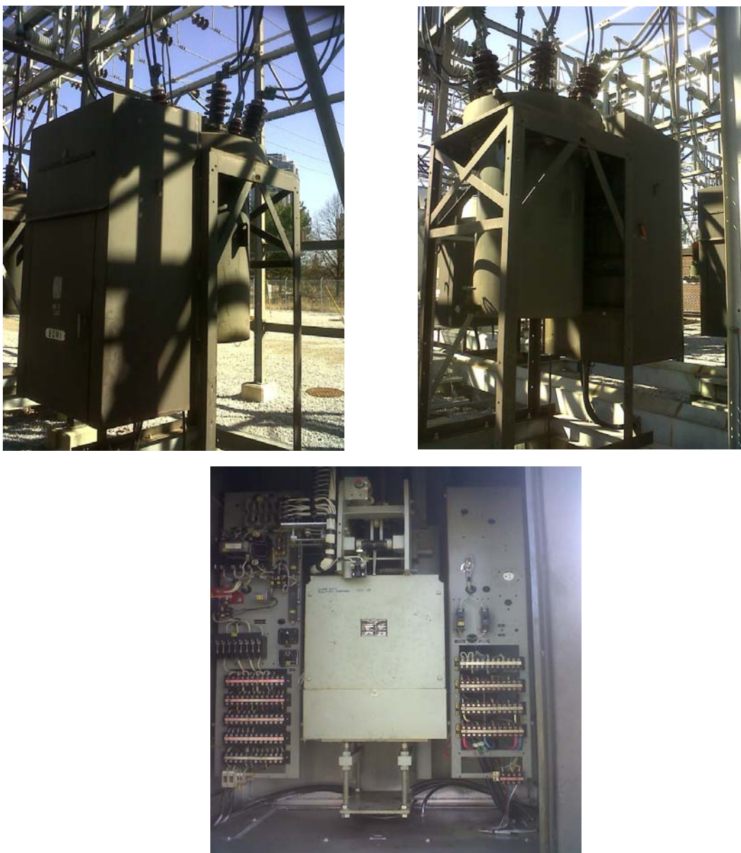
Figure 8: Circuit Breaker at Fairchild TS 80M1 (March 14, 2012)
