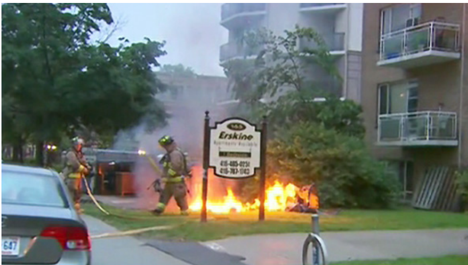
4 Figure 8 - Vault fire on Erskine Ave, near Yonge and Eglinton. Photo from ctv.ca, taken June 1, 5 2010.
