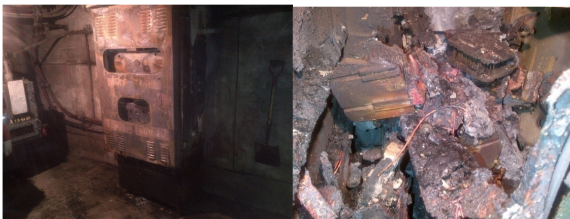
6 Figure 4: The figures above show the damaged equipment from the failure at 33 Princess 7 Street. The fire destroyed the ATS unit (right). PHOTO TAKEN January 17, 2012
