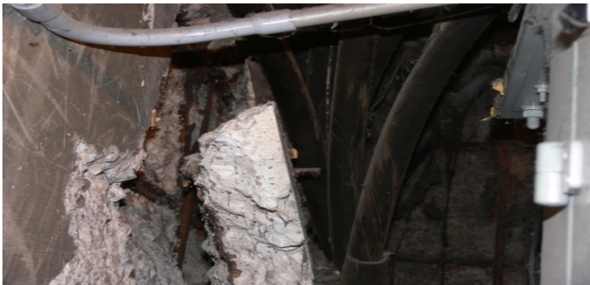
Figure 12: Photo of a large portion of concrete detached from vault wall King/Yonge St
