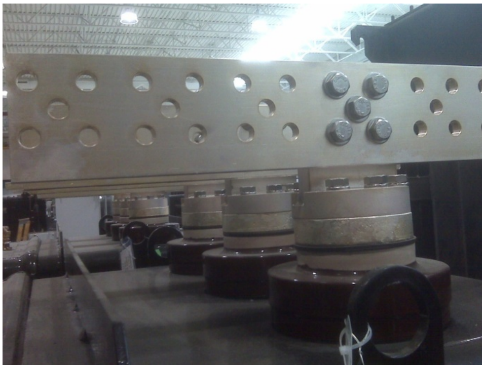
1 Figure 8 - Submersible Network Unit. Secondary Bus raised above top of Protector. 2 (September 4, 2009)
