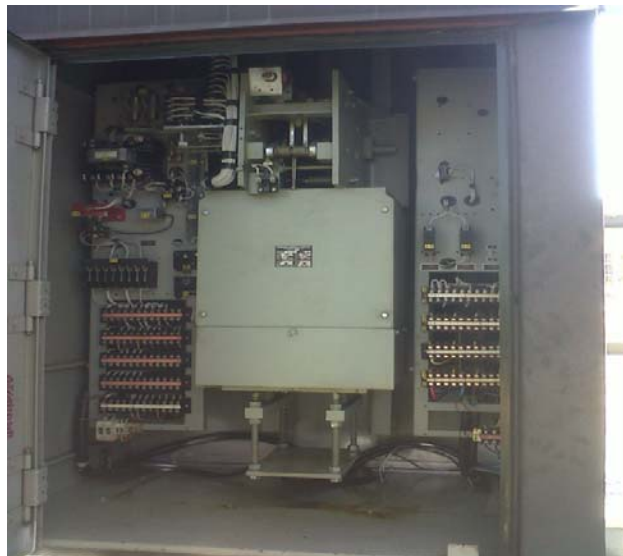
Figure 10: Circuit Breaker at Fairchild TS 80M5 (March 14, 2012)
