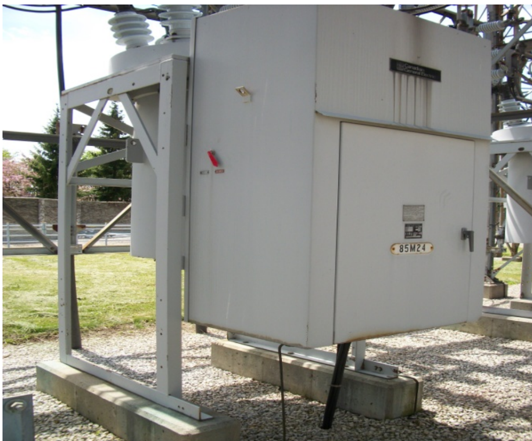
Figure 5: Circuit Breaker at Bathurst TS 85M24 (May 20, 2011)
