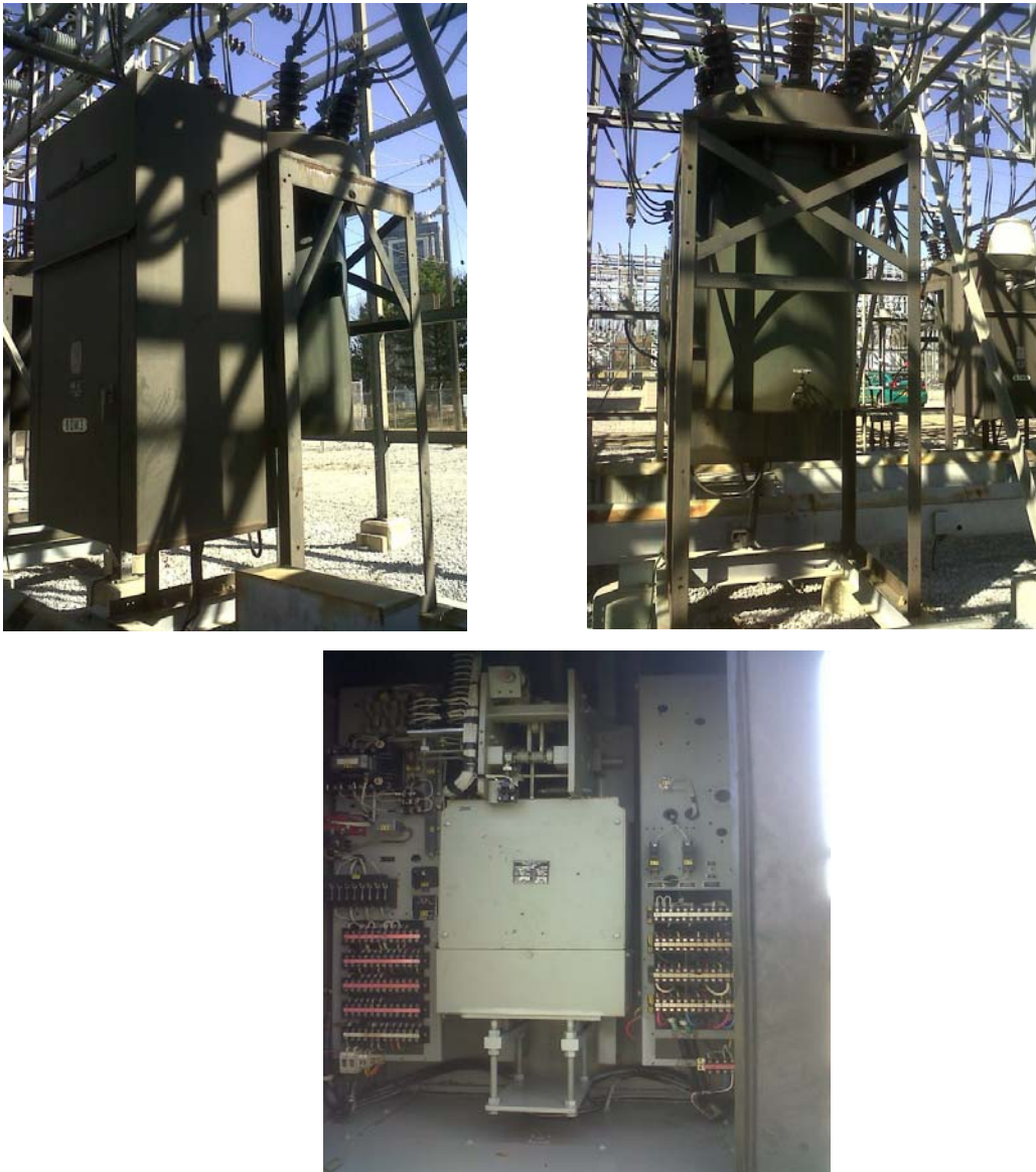
Figure 9: Circuit Breaker at Fairchild TS 80M3 (March 14, 2012)
