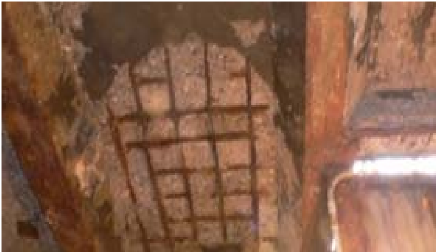
13 Figure 5: Roof Exposed Rebar
