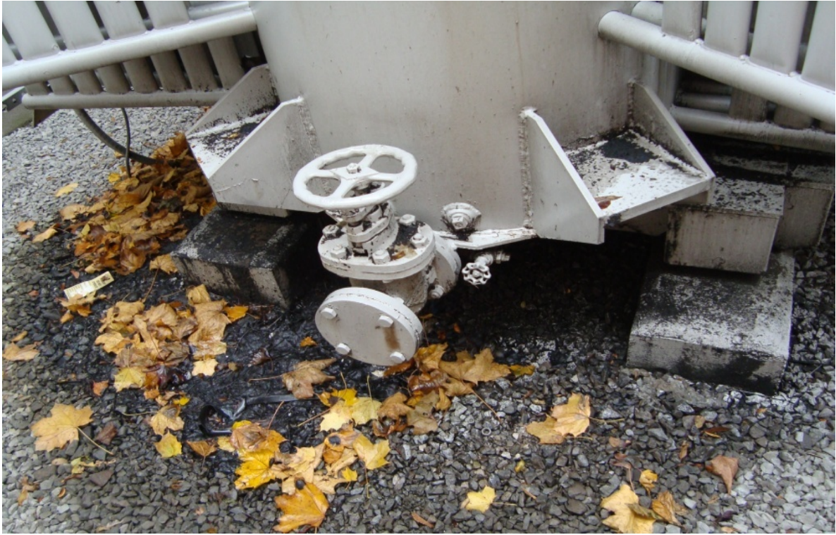
1 Figure 1: Station Transformer, TR1, leakage at Ellesmere White Abbey MS (November 16, 2 2011)
