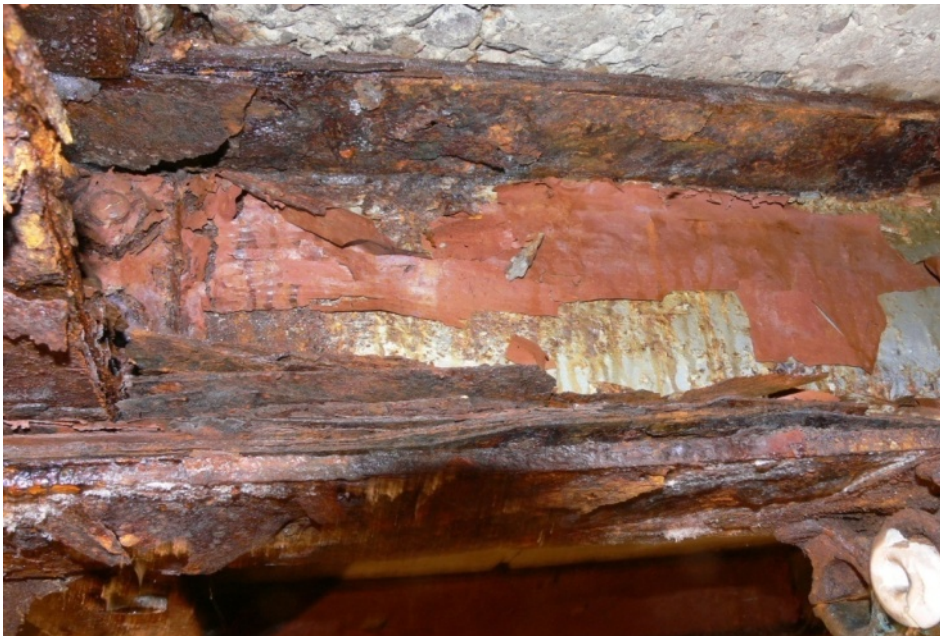
8 Figure 7: Corroded I-Beams
