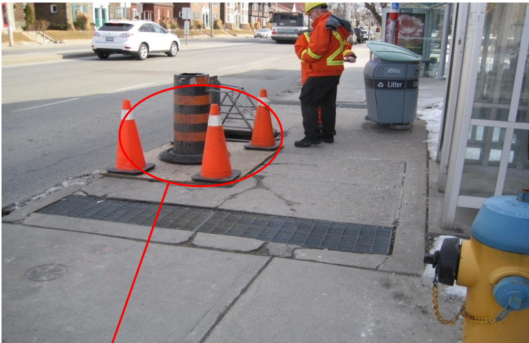
Figure 10: Structural failure of vault located near Lawrence/Yonge St front of a bus shelter, with plywood temporarily covering the hole in sidewalk.
