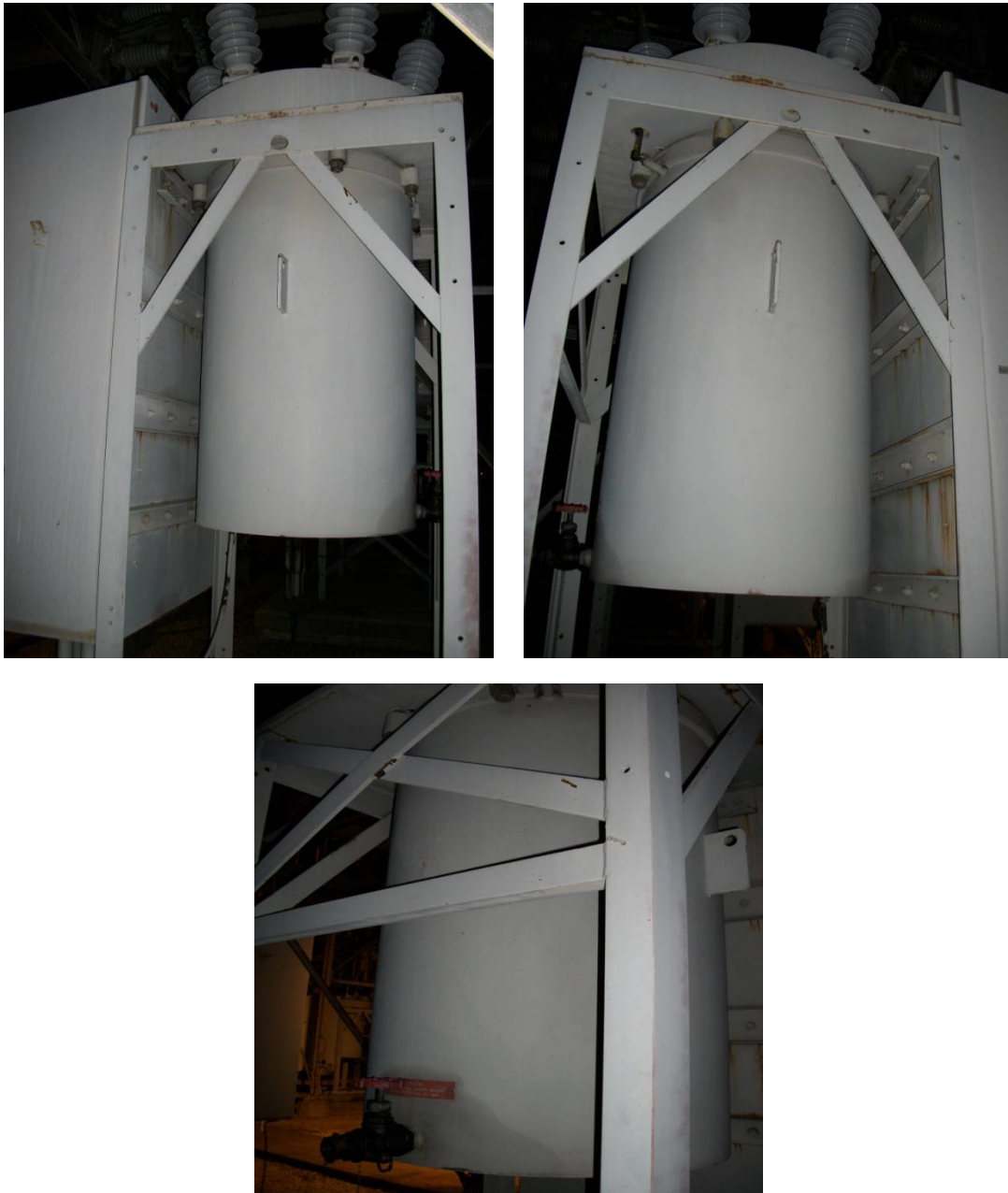
Figure 23: Circuit Breaker at Bathurst TS 85M25 (February 2, 2012)
