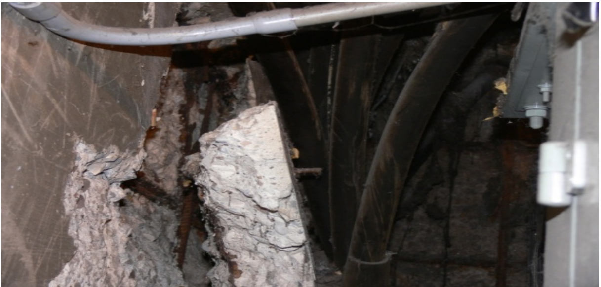
Figure A: Photo of a large portion of concrete detached from vault wall King/Yonge Street
