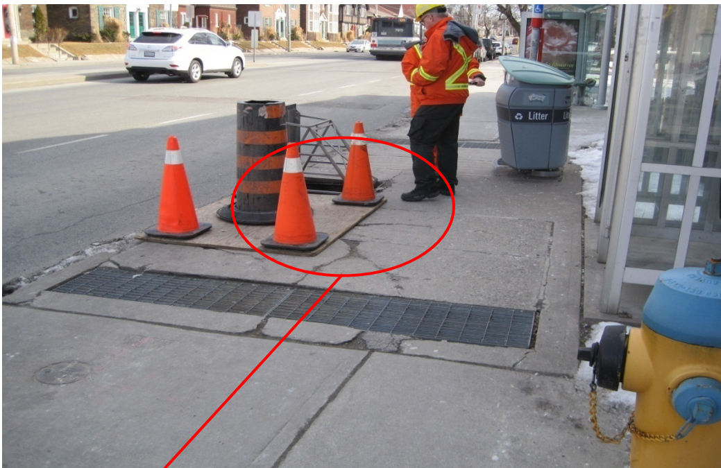
14 Figure B: Structural failure of vault located near Lawrence/Yonge Street front of a bus shelter, 15 with plywood temporarily covering the hole in sidewalk.
