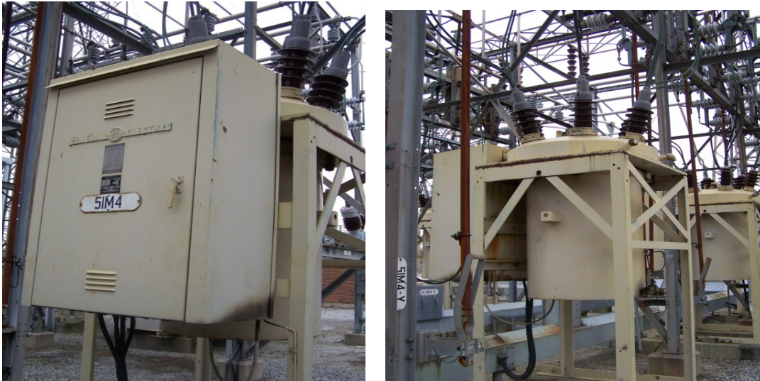
Figure 6: Circuit Breaker at Leslie TS 51M4 (February 3, 2012)
