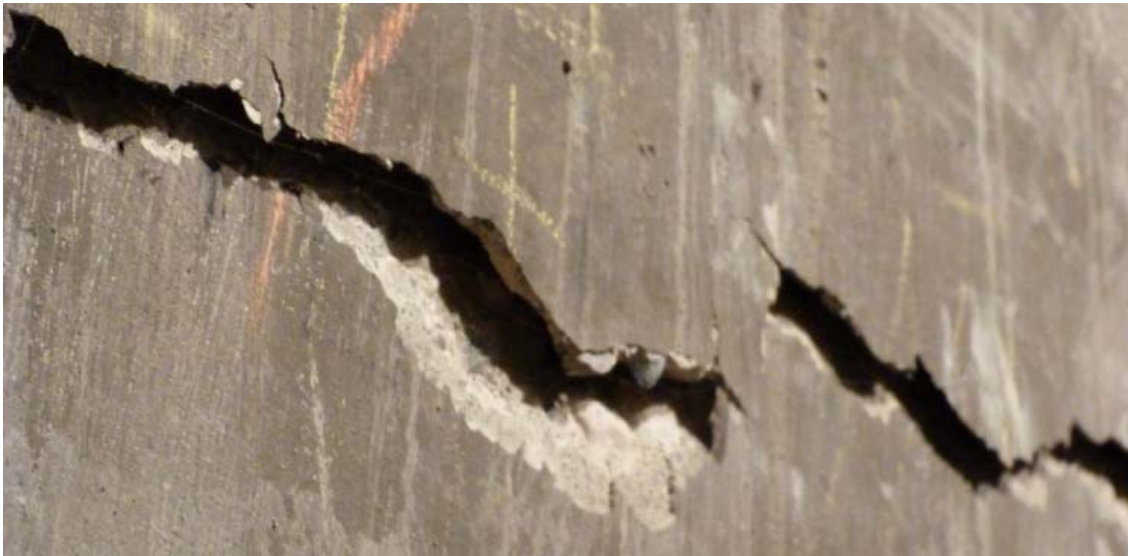
1 Figure 9: Cracked Wall
