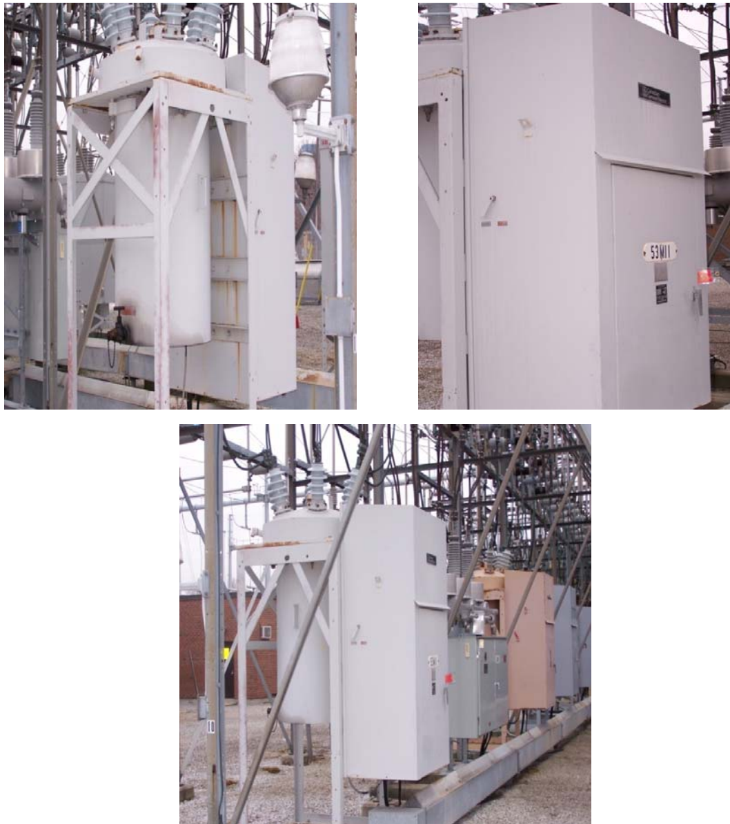
Figure 16: Circuit Breaker at Bermondsey TS 53M11 (February 3, 2012)
