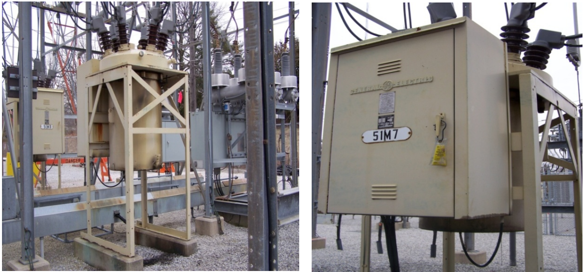
Figure 12: Circuit Breaker at Leslie TS 51M7 (February 3, 2012)
