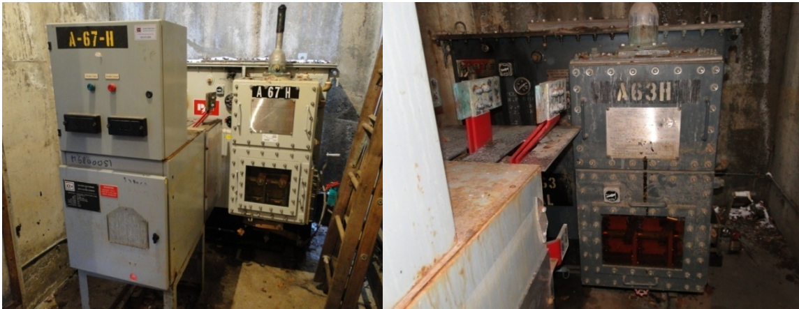
1 Figure 6: RPB units following failure at 50 Marlborough. PHOTOS from January 10, 2010
