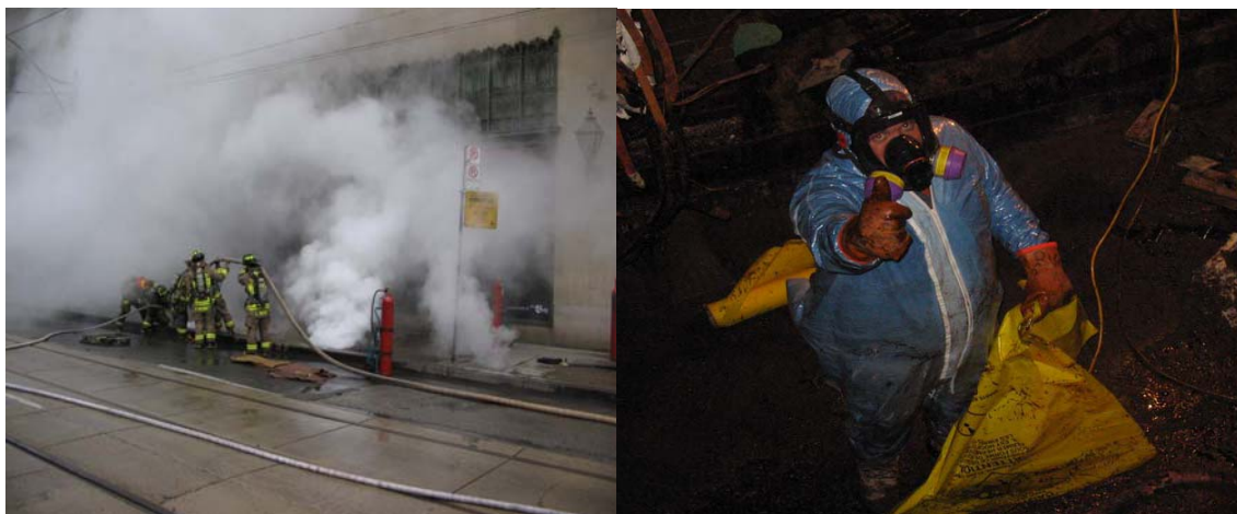
15 Figure 5 - LEFT: Fire fighters working to extinguish the fire. RIGHT: Asbestos Clean-up.
