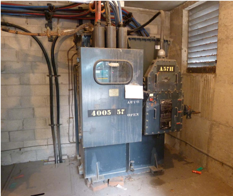
1 Figure 10 – Walk-in Building Network Vault. (November 2011)
