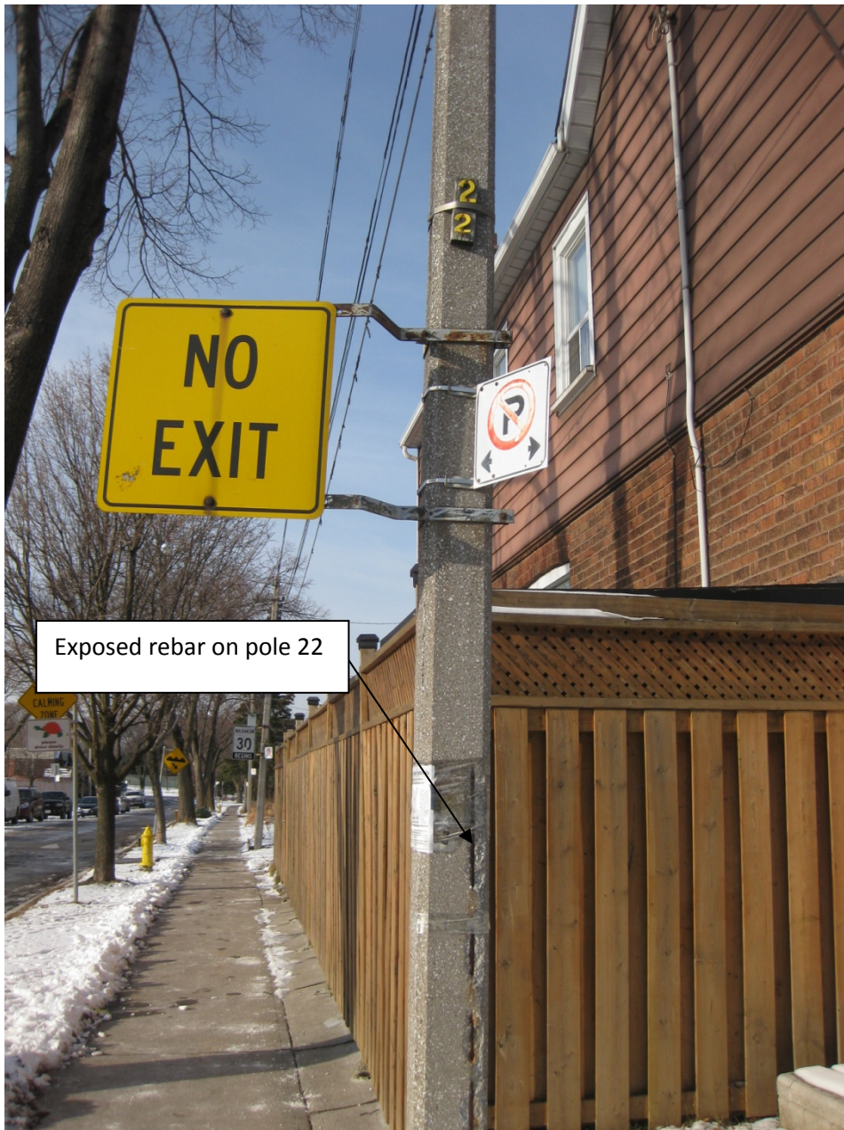
1 Figure 18: Exposed Rebar on B5HW (January 16, 2012)
