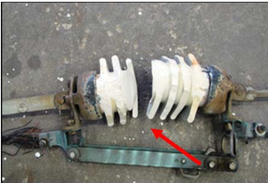
2 Figure 48: Broken Porcelain In-Line Switch
