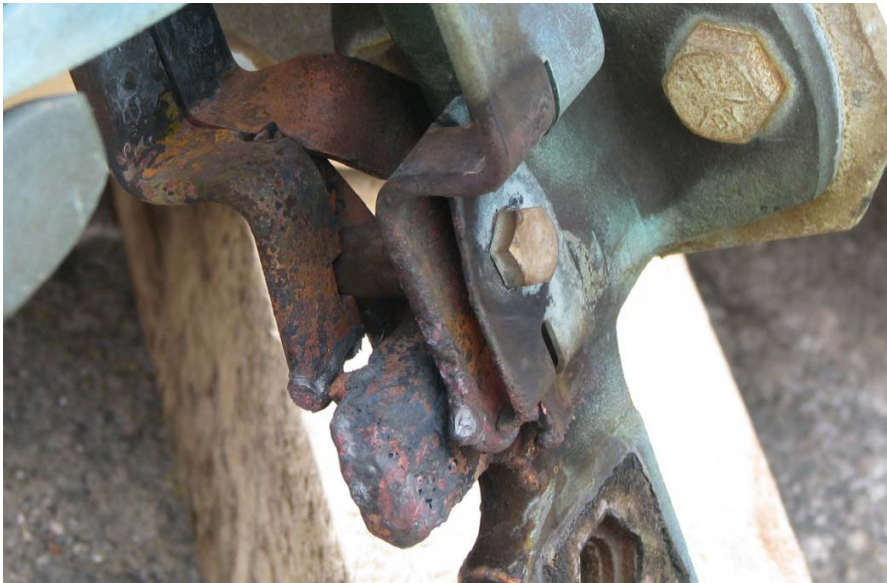
1 Figure 52: Severely corroded switch blade
