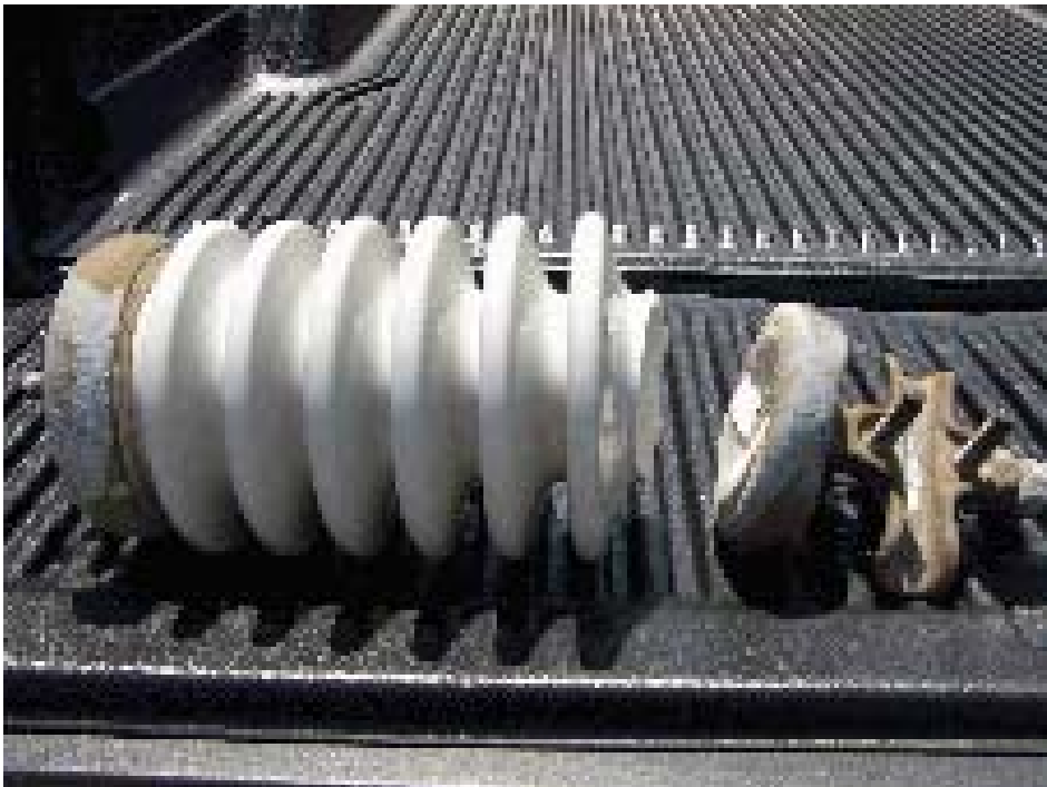
1 Figure E: Broken Porcelain Insulator
