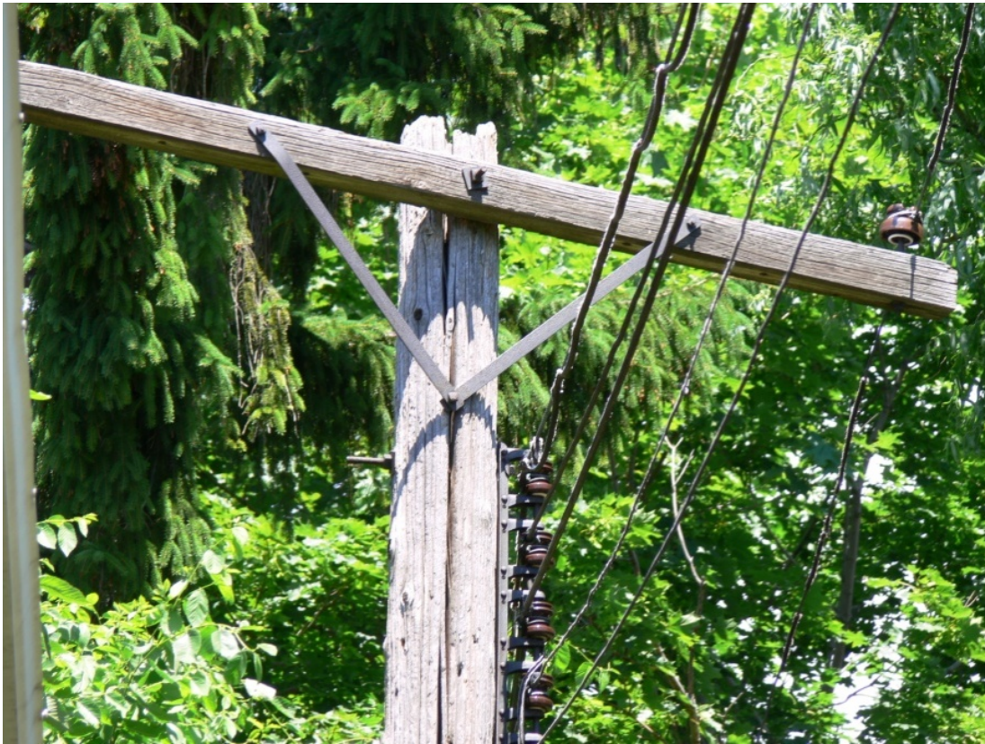
1 Figure 4: Rear lot pole in poor condition
