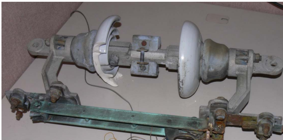
4 Figure 46: In-line disconnect with part of the porcelain insulation broken off
