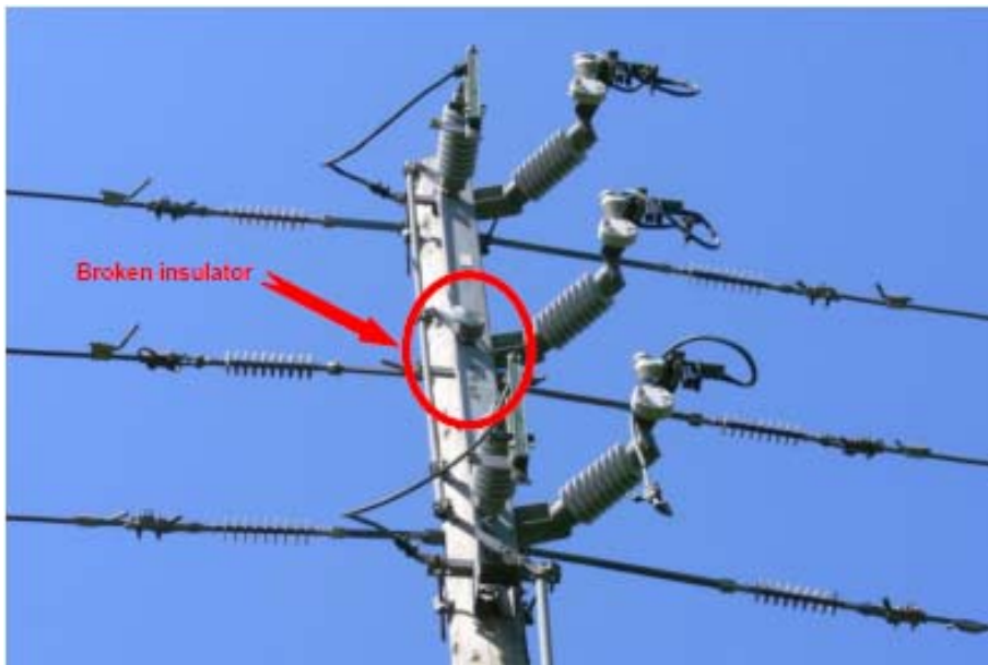
9 Figure 49: OSL65907 with broken center phase insulator
