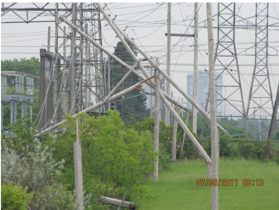
10 Figure 8: Multiple Pole Failure
