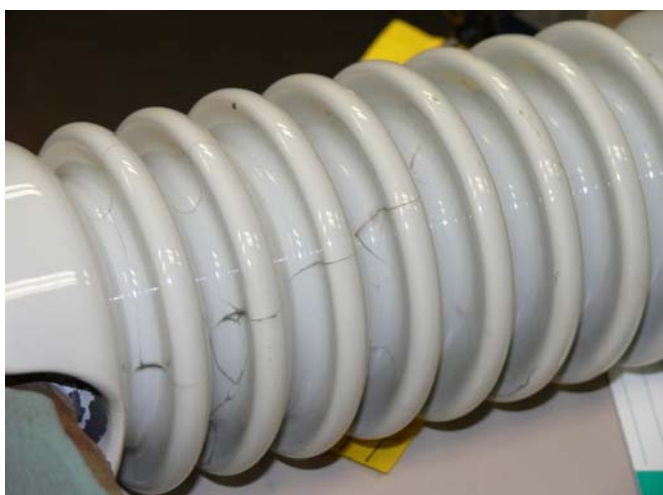
18 Figure 38: Cracked porcelain insulation
