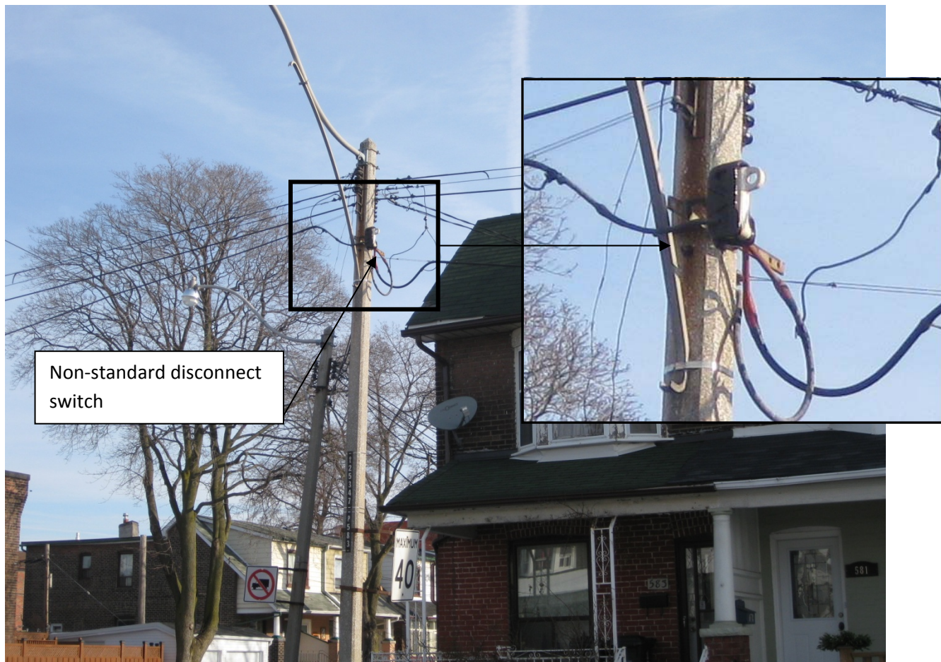
1 Figure 17: Obsolete Disconnect Switch on B5HW (January 16, 2012)
