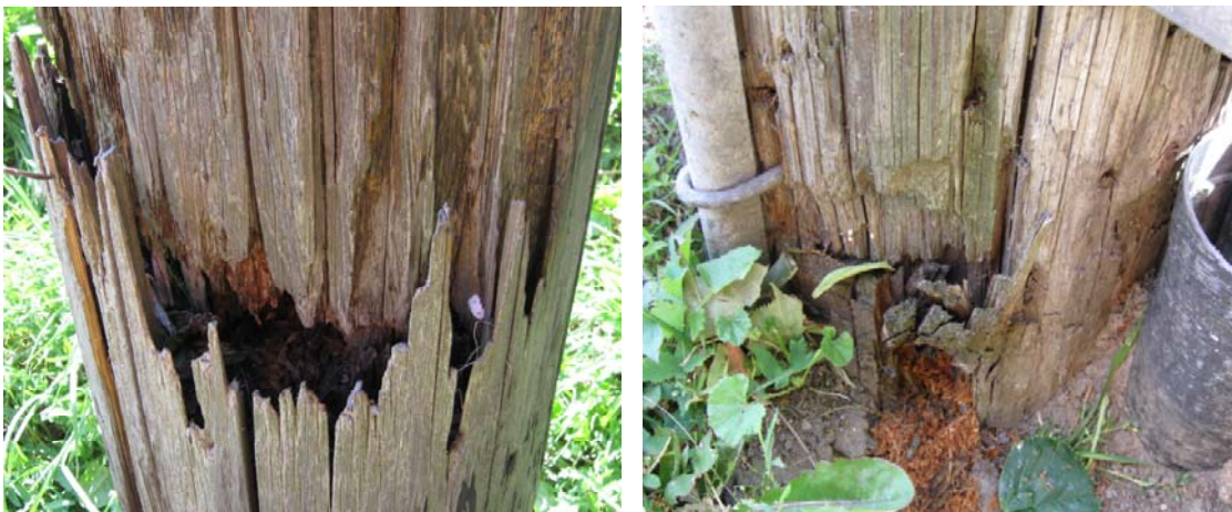
7 Figure 4: Internal base rot
