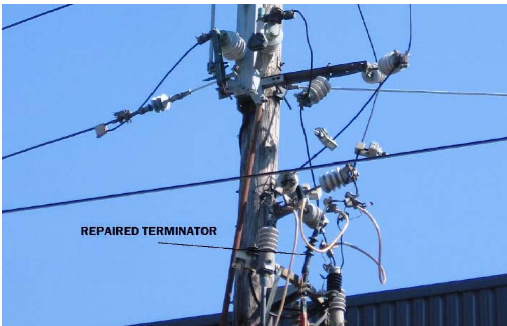
3 Figure 57: Replaced Porcelain Pothead Terminator
