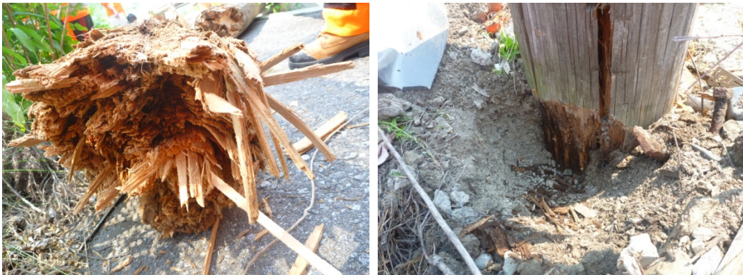
1 Figure 7: Deteriorated pole base
