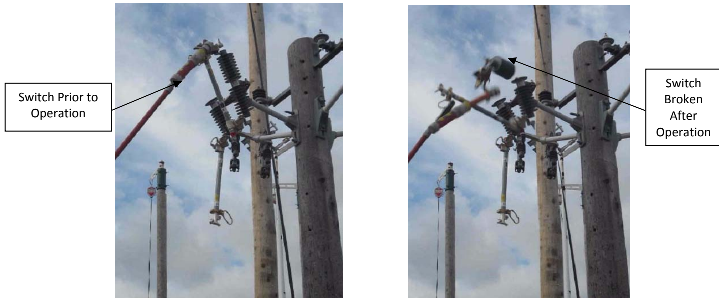
Figure 4: Before and After Switch Operation
