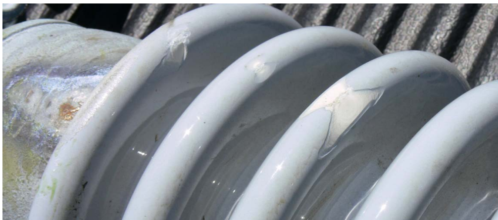
1 Figure 50: Close-up of Damaged Porcelain Switch Insulator showing tracking
