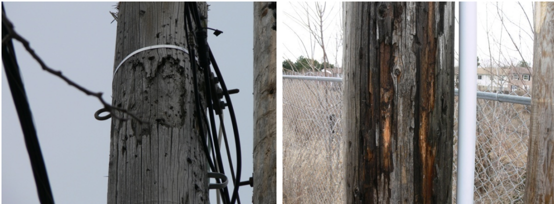
3 Figure 6: Body of the pole rot and burnt
