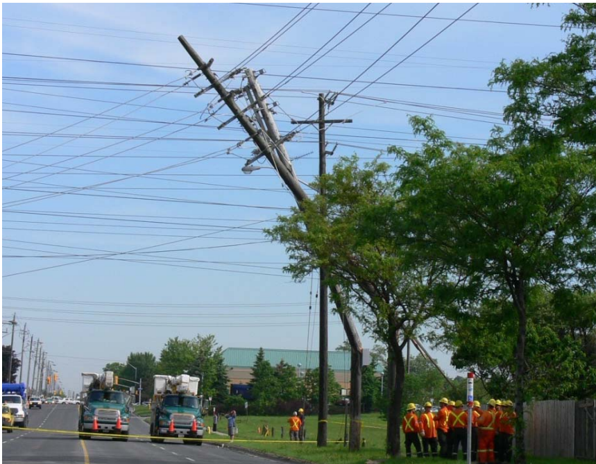
1 Figure 9: Multiple Pole Failure
