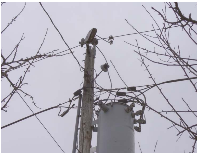
8 Figure 9: Example of Non-standard Assets in the Rexdale Colony Rear Lot Area (photo taken in 9 2012)
