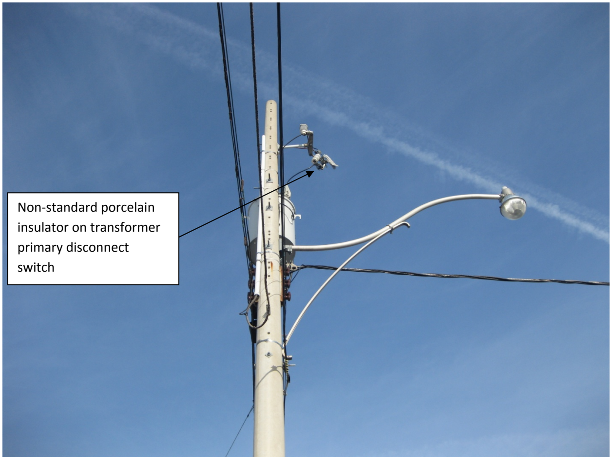
1 Figure 16: Non-Standard Porcelain Insulator on B5HW (January 16, 2012)
