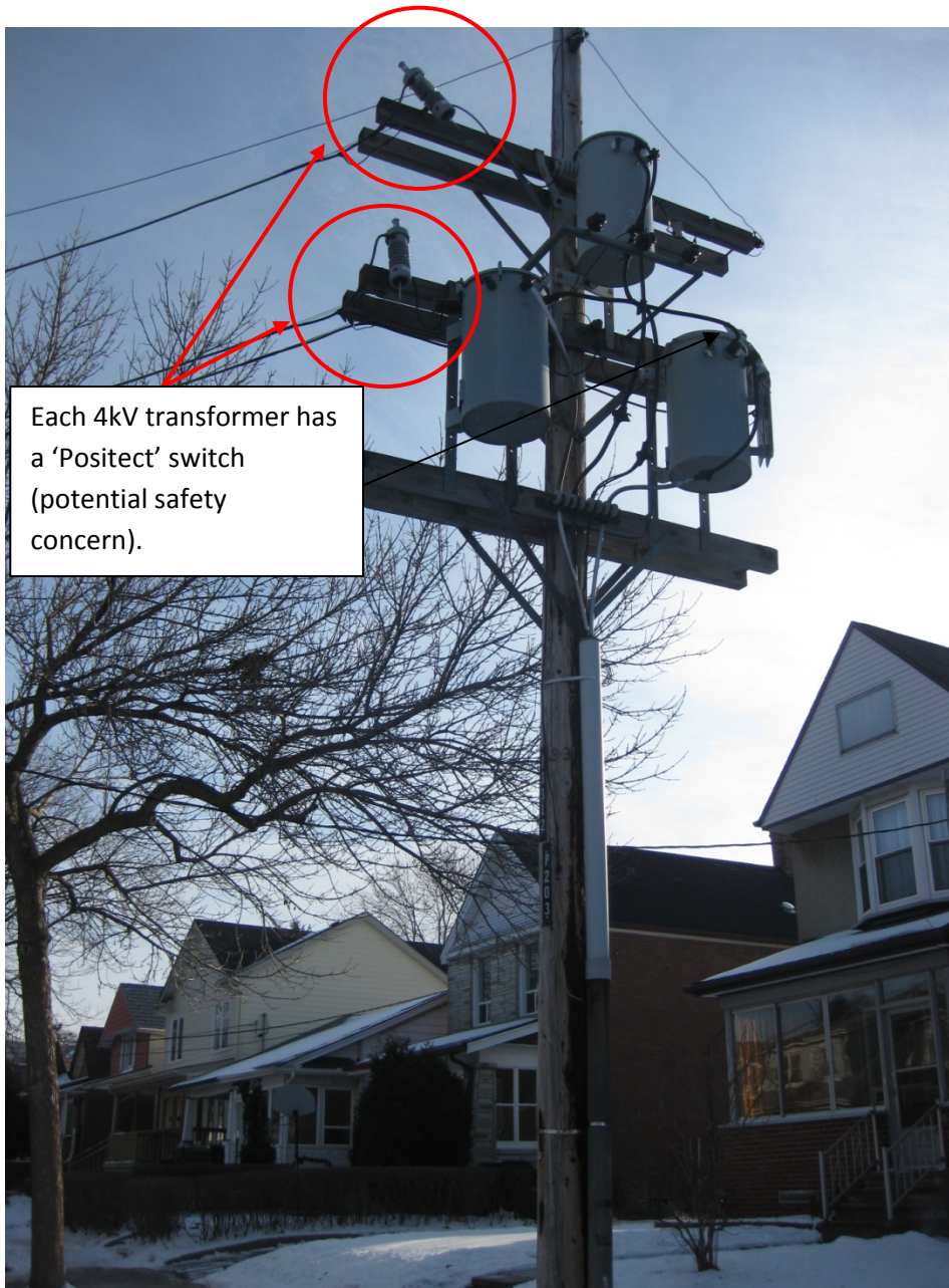
1 Figure 15: 'Positect' Disconnect Switch on B3HW (January 16, 2012)
