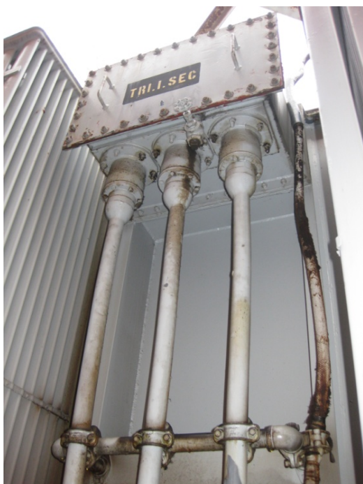
8 Figure 8: Transformer TR1 with signs of oil leakage (January 16, 2012)
