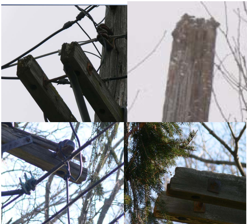
1 Figure 5: Aging and poor condition plant in the Rexdale Colony, Forest Hill, and Thorncrest 2 rear lot area (photo taken in 2012)
