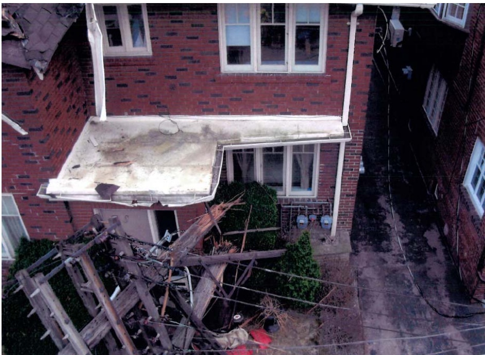
2 Figure 14: Damage from Pole Down on Acacia Road
