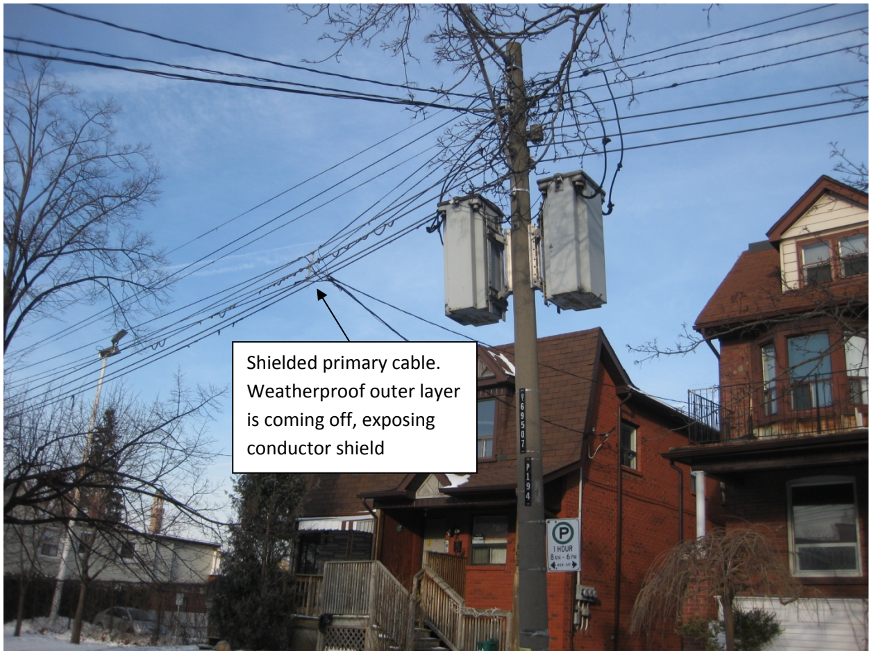
1 Figure 19: Poor Condition Equipment on B3HW (January 16, 2012)
