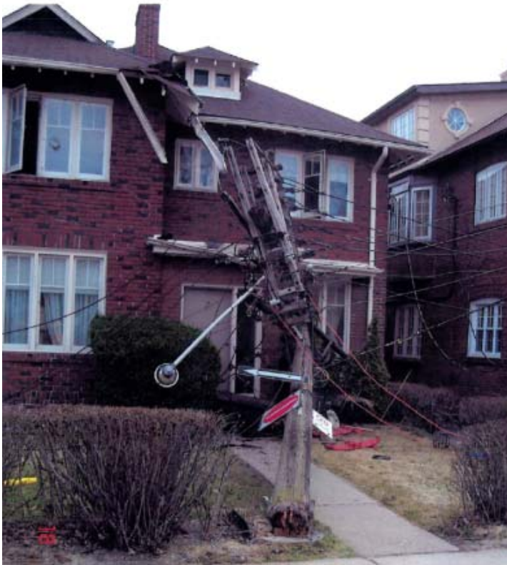
1 Figure A: Fallen Pole on Acacia Road with Rotten Base
