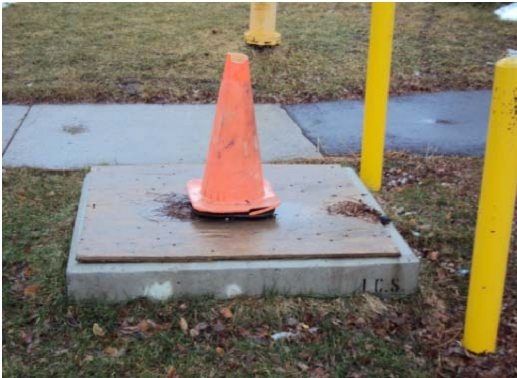
1 Figure 16: Civil work that has been completed in the Rexdale Colony rear lot area, awaiting 2 electrical installation (photo taken in 2012)
