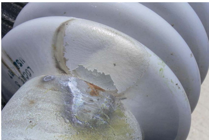
3 Figure 51: Close-up of Damaged Porcelain Switch Insulator showing tracking
