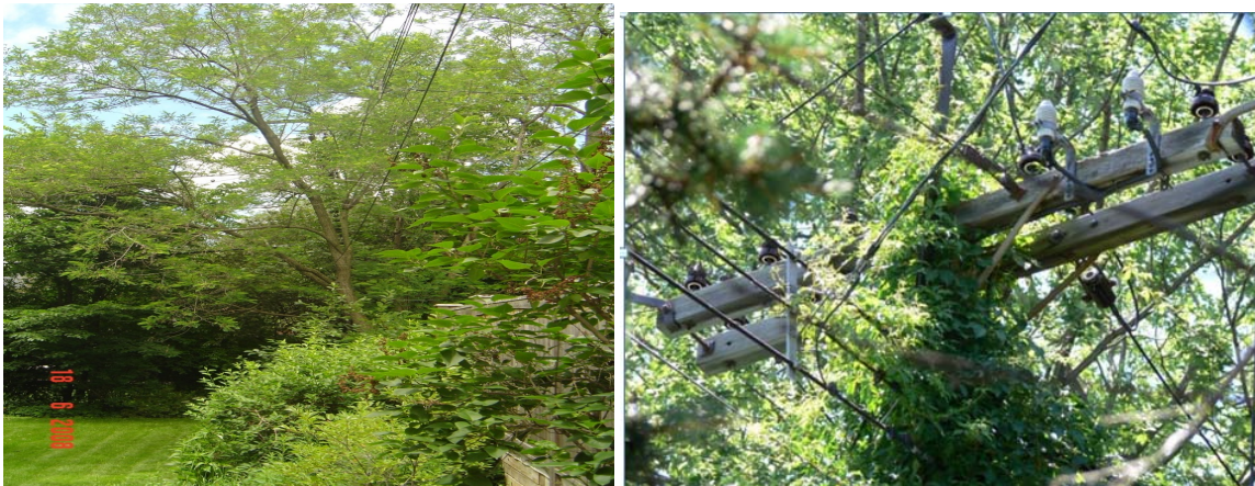
10 Figure 10: Excessive vegetation in close proximity to rear lot distribution assets
