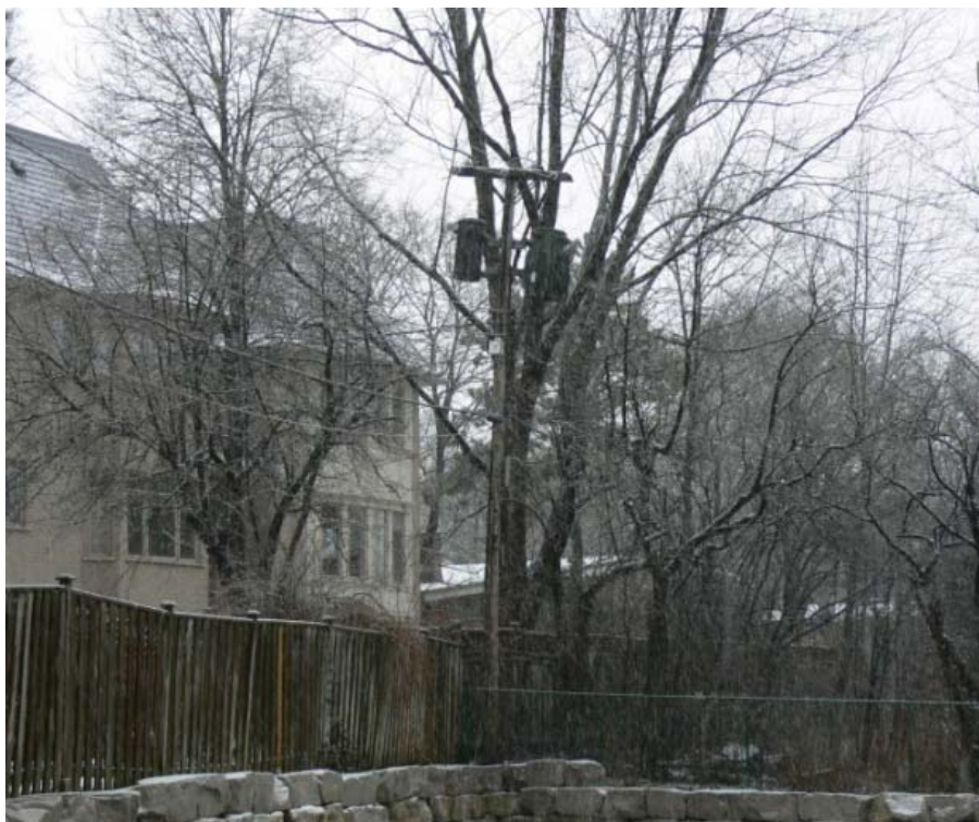
1 Figure 7: Limited access to critical THESL asset –transformer (photo taken in 2012)
