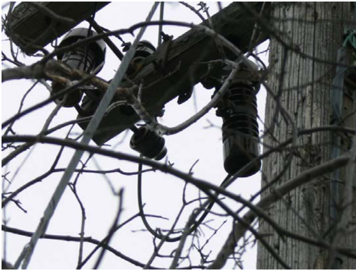
1 Figure 8: Non-standard Positect switches in the Rexdale Colony rear lot area (photo taken in 2 2012)
