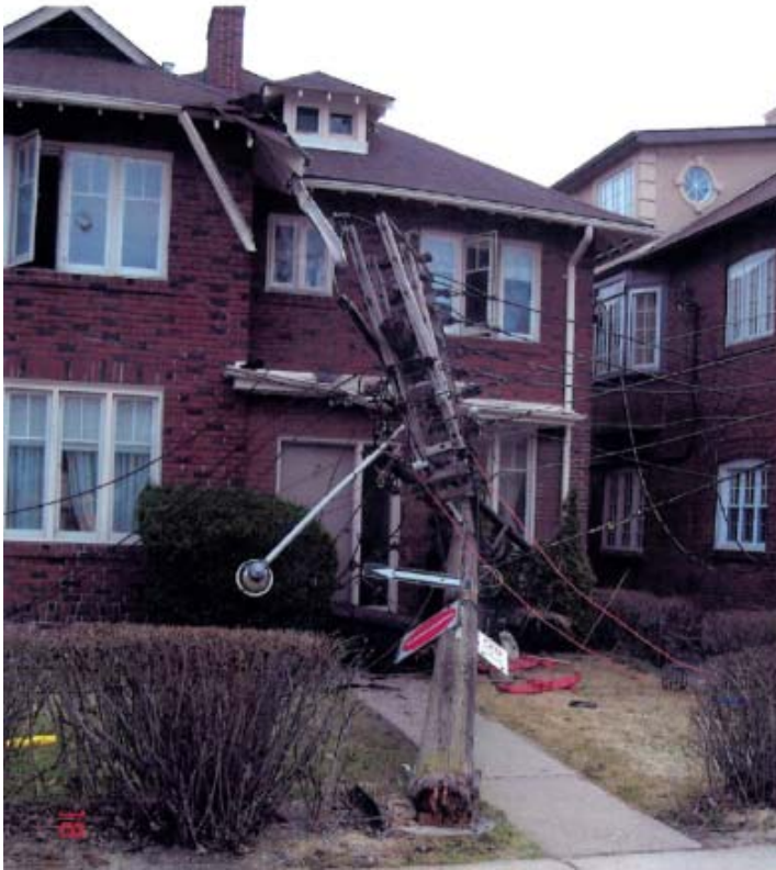
1 Figure 15: Fallen Pole on Acacia Road with Rotten Base
