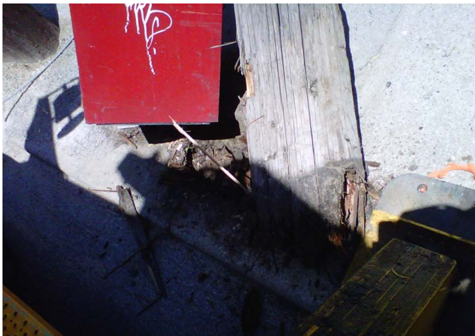
1 Figure 12: Pole base rot at Pape Avenue
