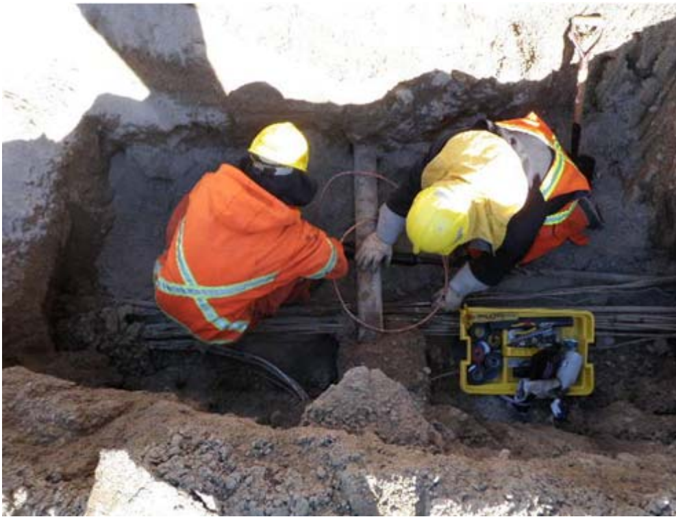
1 Figure 1: Field personnel within a splice-pit preparing to splice a faulted cable to restore 2 service to area. (Taken on February 15, 2011)
