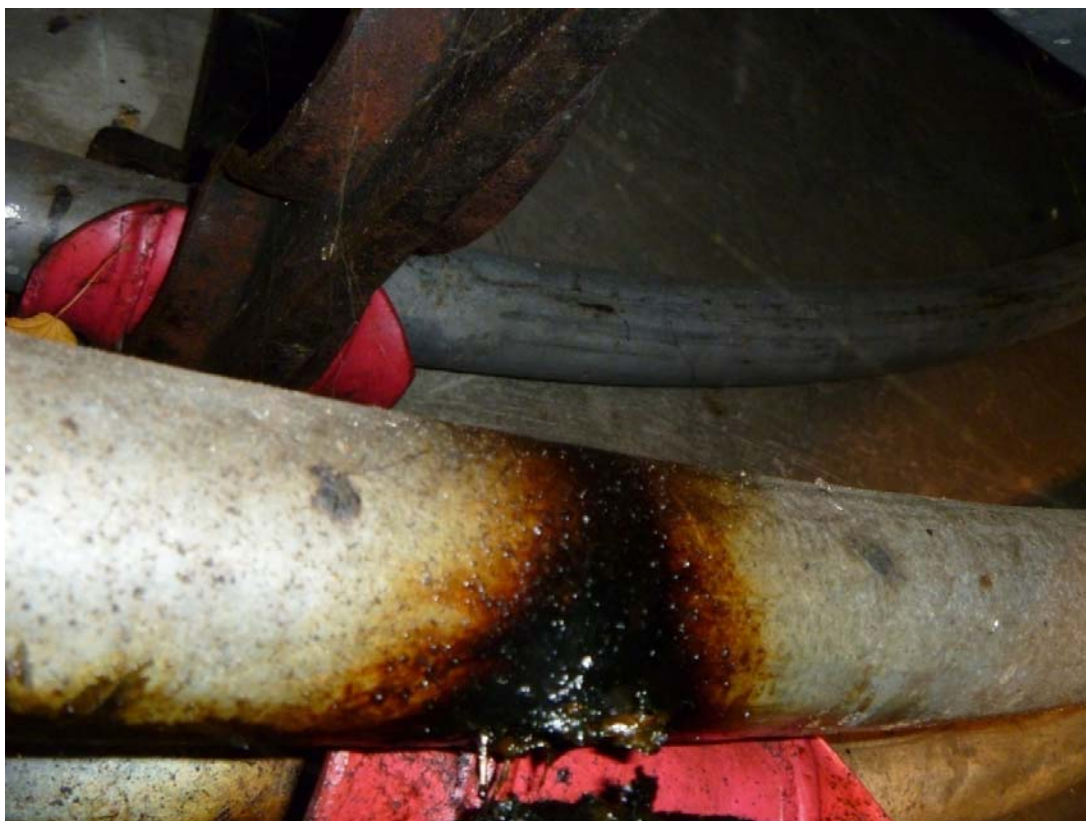
1 Figure 1: Leaking PILC Cable (January 18, 2012)
