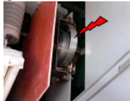
BROKEN SPRING IN PS11787
