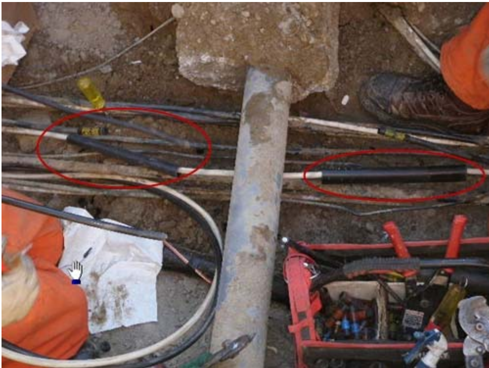
1 Figure 3: Field personnel completed splicing the cable. Notice two splices required for each 2 faulted cable segment. (Taken on February 15, 2011)
