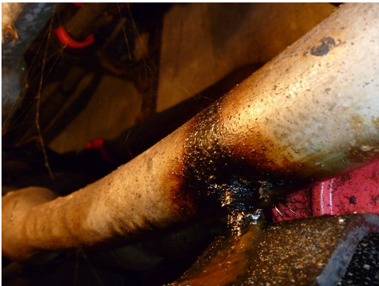
1 Figure 5: Leaking Oil from PILC Cables Connecting Bridgman to High Level Stations 2 (January 18, 2012)
