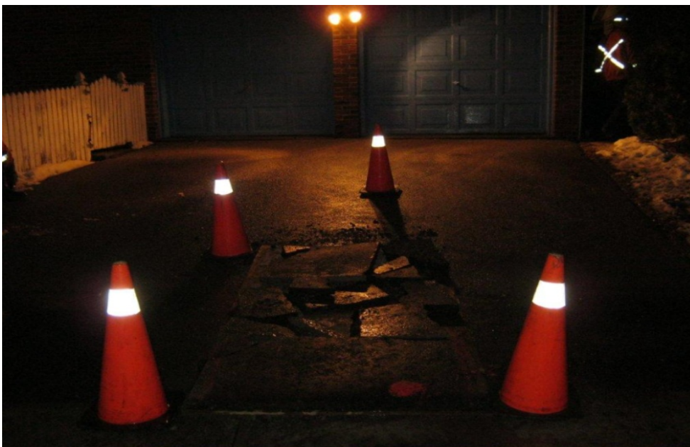
3 Figure 4: Disturbance to customer in the middle of the night to repair cables and restore 4 service. (Taken on January 27, 2012)
