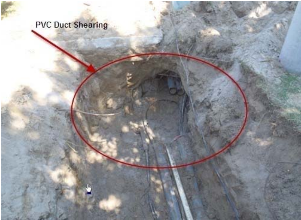
1 Figure B3: Shearing of PVC ducts due to the natural movement of the earth (taken on July 12, 2 2011)
