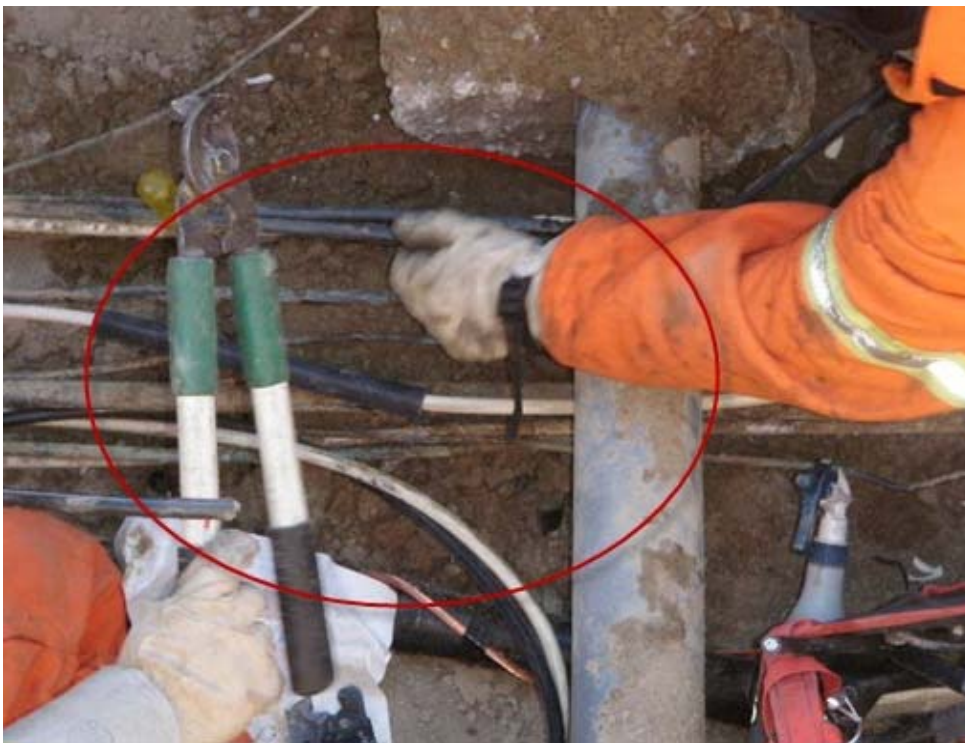
11 Figure 2: Field personnel within splice-pit, removing faulted cable segment. (Taken on 12 February 15, 2011)
