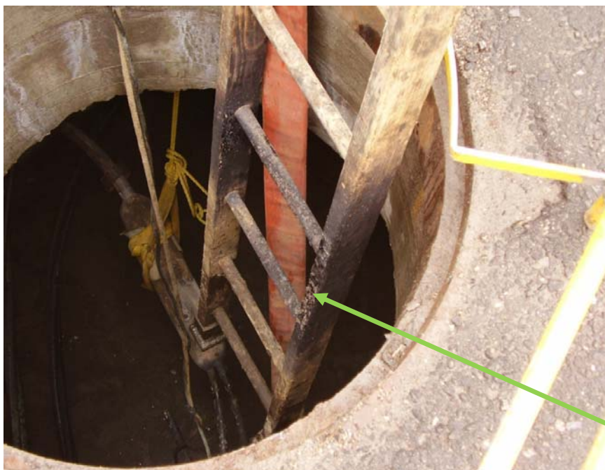
1 Figure 11: Piece out cable is shown obstructing entry to cable chamber. Burns are seen on the 2 ladder where the cable made contact with the ladder (Note: ladder not in original position 3 but raised for the photo, April 27, 2007)
