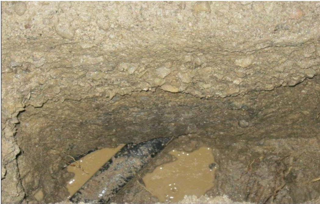
1 Figure 5: Typical environment of direct buried cable over its service life—surrounded by rocks 2 and immersed in mud. (Taken on January 27, 2012)
