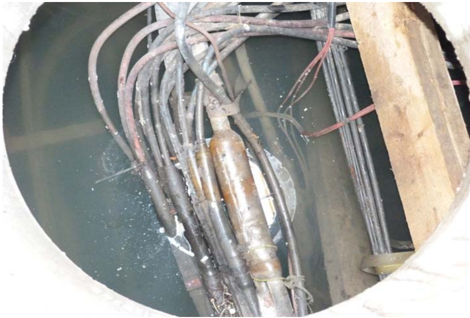
1 Figure 8: Before — Cable Chamber requiring Piece Outs at Yonge and Mt. Pleasant 2 (January 16, 2012)
