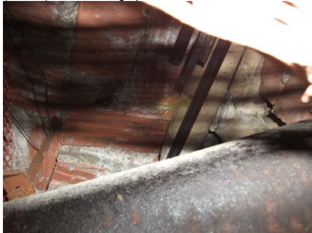
Photograph 10: [Rm. 24] Two damaged asbestos-containing pipe fittings in bulkhead/ceiling space.
