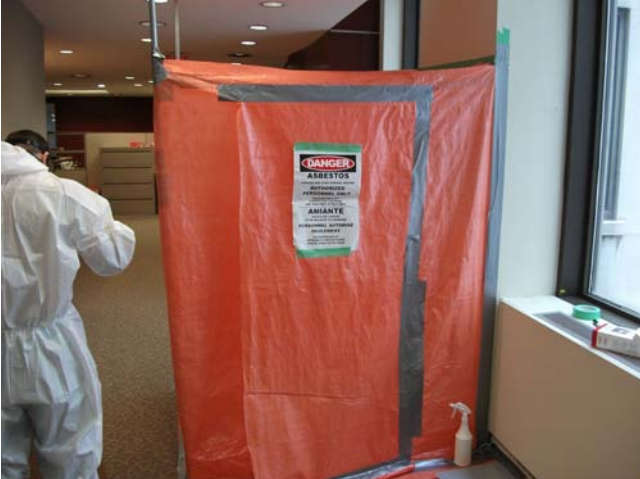
Photograph 13: [Rm. 6] View of enclosure to control asbestos release during 1'x1' hatch installation (#1).
