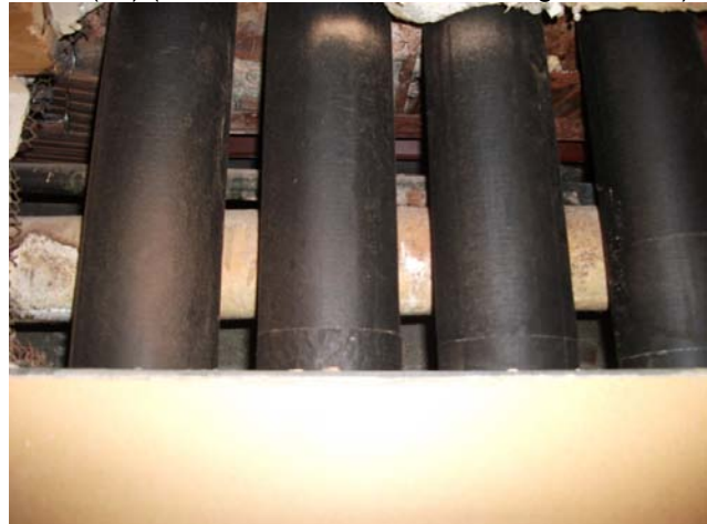
Photograph 16: [Rm. 16] View inside newly-installed hatch (#2). Asbestos-containing white mag block pipe insulation in background (Sample set TH-9).
