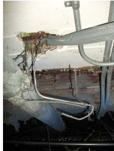
Photograph 4: [Rm. 8] Damaged plaster and fibrous fireproofing in ceiling space.
