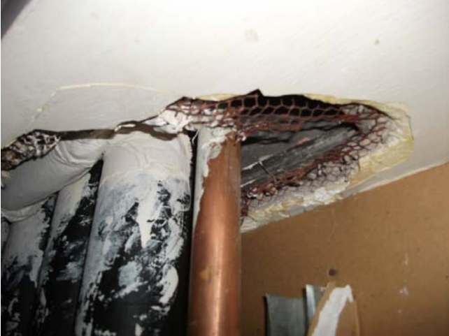
Photograph 1: [Rm. 1] Damaged plaster bulkhead (Sample set TH-2) and asbestos-containing mag block pipe straight insulation (Sample set TH-9).
