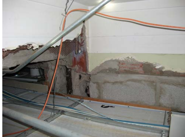
Photograph 2: [Rm. 5] Damaged plaster and lead-containing green paint in ceiling space (Sample TH-L4).
