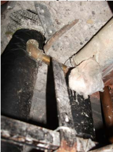
Photograph 9: [Rm. 10] Damaged asbestos-containing pipe fitting in bulkhead/ceiling space.
