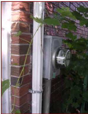
Figure 5-1, Electric Meter at Rear Left Corner of Dwelling
