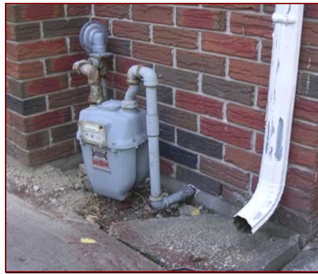
Figure 5-2, Outdoor Gas Meter at Rear Right Corner of Dwelling
