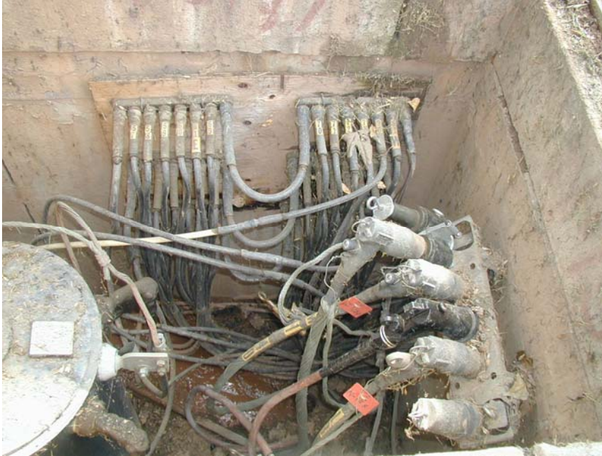
1 Submersible Transformer Vault before rebuild project is complete
